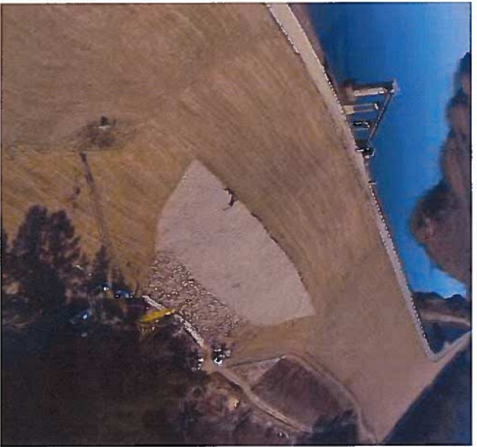
Completed work on the dam embankment undertaken as part of the Pine Creek Lake dam safety project.
