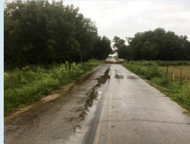
Before: road damage with closed road barrier
