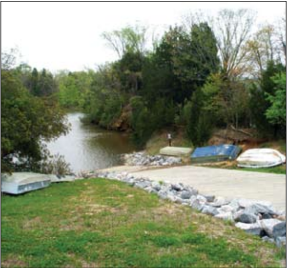
A disappearing act: inappropriate vegetation overgrows an embankment dam, now obscured.
