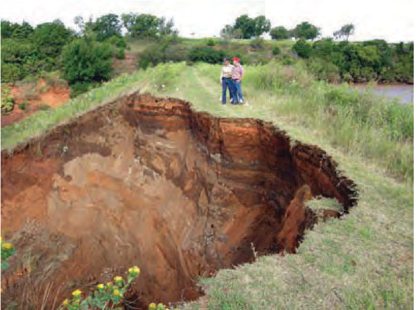
SCS Sugar Creek Site # 44 dam, Caddo Cnty, OK washed out from heavy rains - 2007
