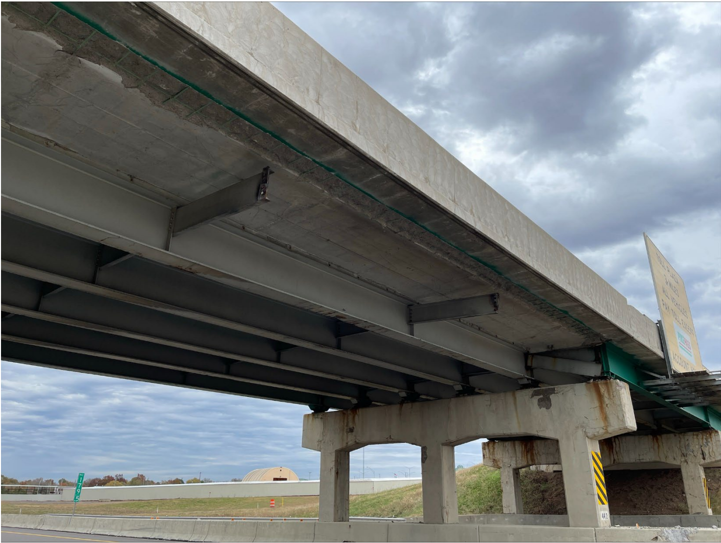
This photo was taken Nov. 9 showing the damage to the westbound I-44/Turner Turnpike bridge to Stroud where a bridge beam was dislodged by an illegal, over-height semi-truck late Nov. 8.
