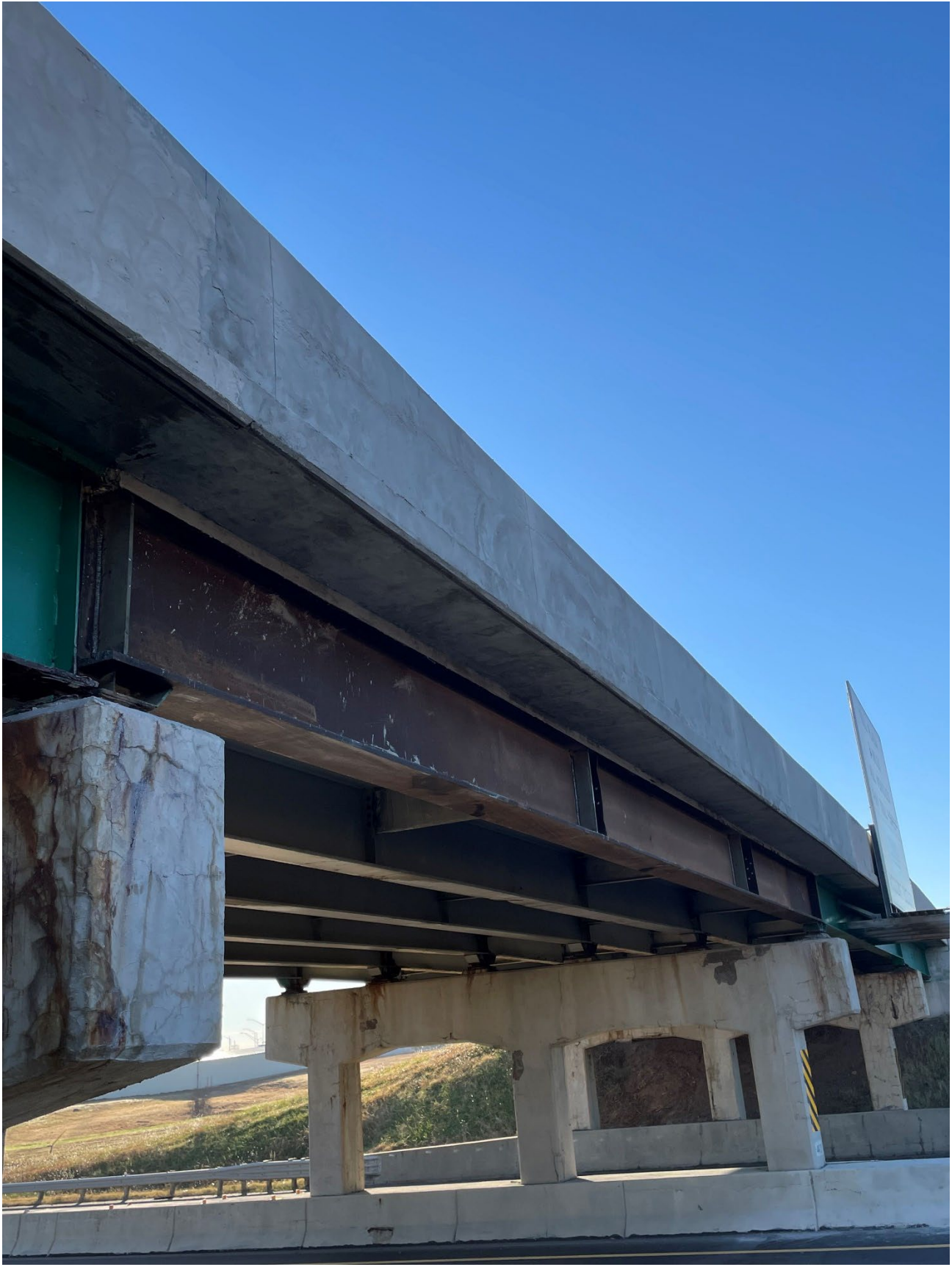
Crews completed emergency bridge repairs early Tuesday morning at the bridge to SH-99 in Stroud. The outside bridge beam was knocked down by an illegal, overheight semi-truck late Nov. 8. Repairs were made in four nights.
