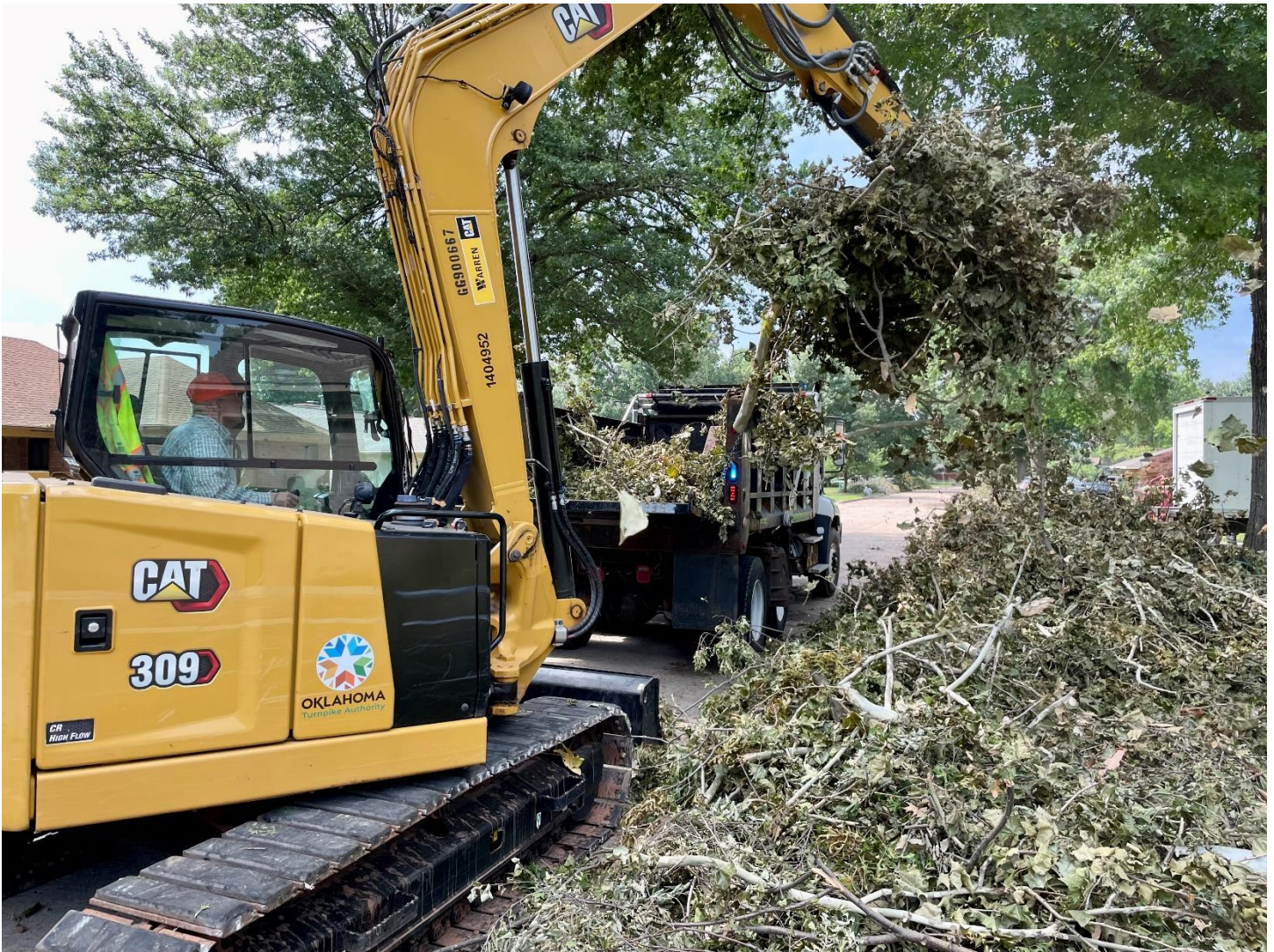
An Oklahoma Turnpike Authority maintenance crew helps remove debris from Tulsa neighborhood streets from a June 18 storm. Crews worked as part of the emergency response for more than three weeks to help clear debris blocking travel throughout Tulsa.
