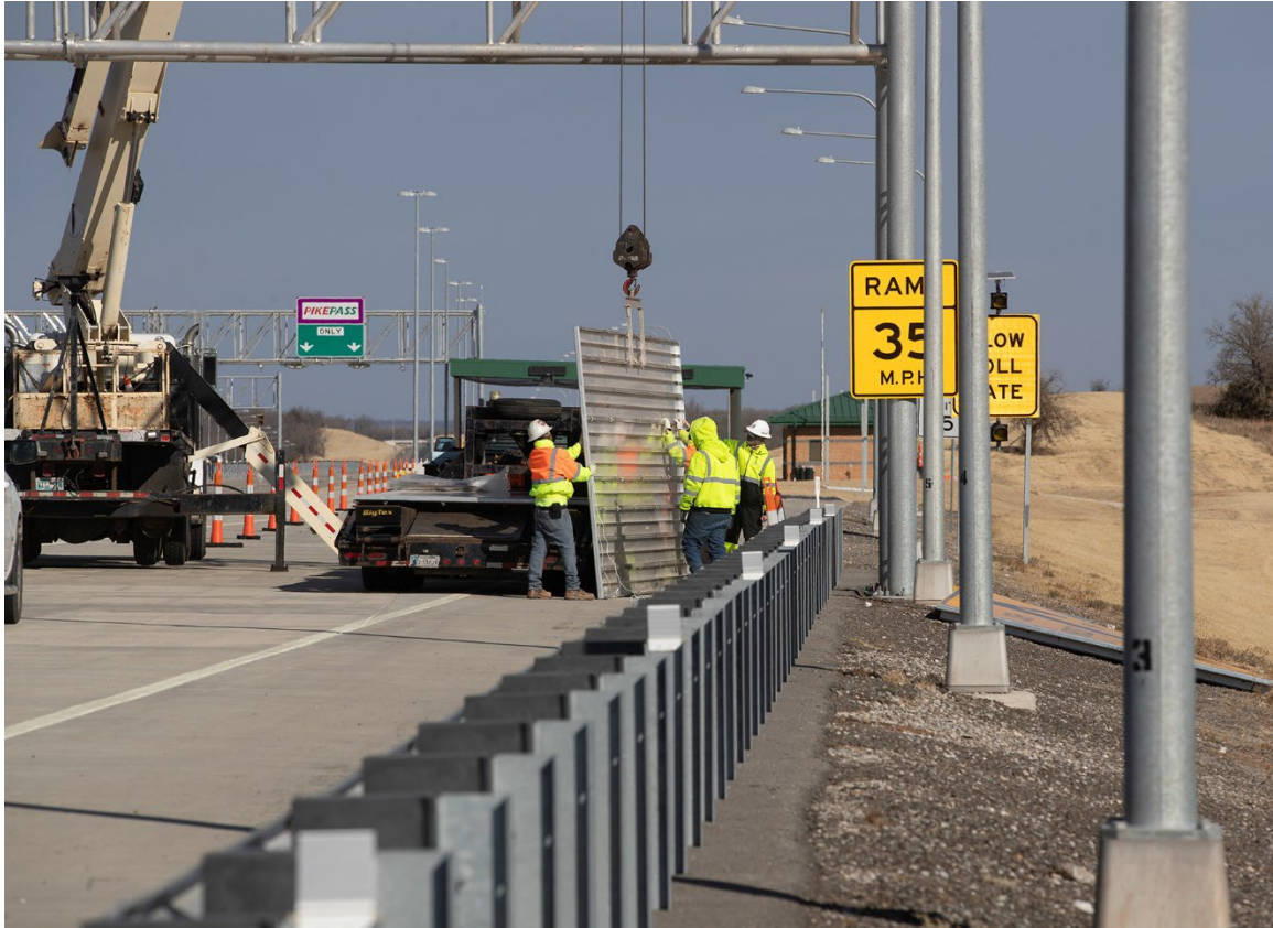
Oklahoma Turnpike Authority crews put new signage in place Tuesday morning as part of converting the Kickapoo Turnpike to PIKEPASS and PlatePay, eliminating toll booths and coin machines from the 21-mile turnpike in Eastern Oklahoma County.
