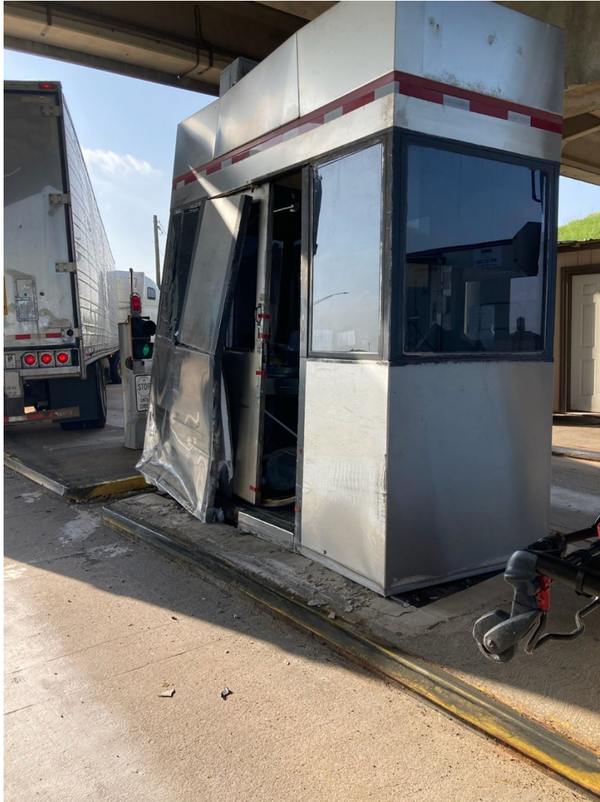
Damage from a semi-trailer truck colliding with an eastbound US-412/Cimarron Turnpike toll booth is shown Monday, May 9, 2022. The toll booth attendant working in the booth was injured and treated on scene.
