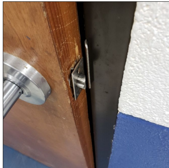
Broken Lock to Custodial Closet
