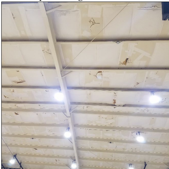
Gym Ceiling Deterioration
