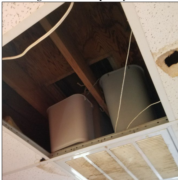
Roofing Leaks Inadequately Addressed
