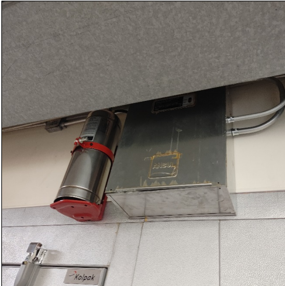
Fire Extinguisher too High for Quick Access
