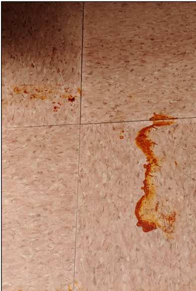
Stains on the Floor
