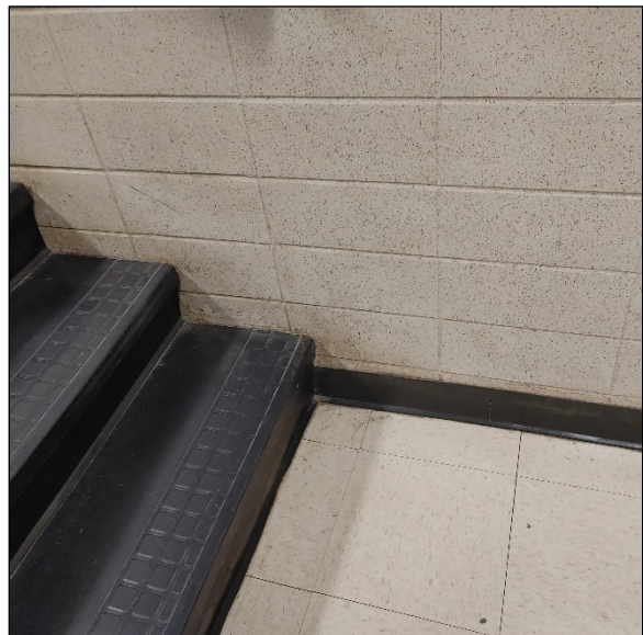
Stains on Wall
