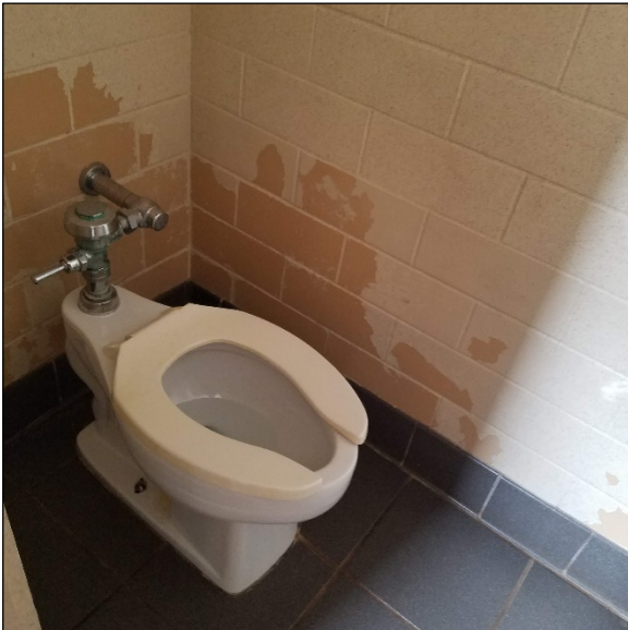
Paint Peeling on Walls
