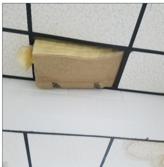
Exhibit 4-27 Ceiling Tile Missing, Broken and Stained
