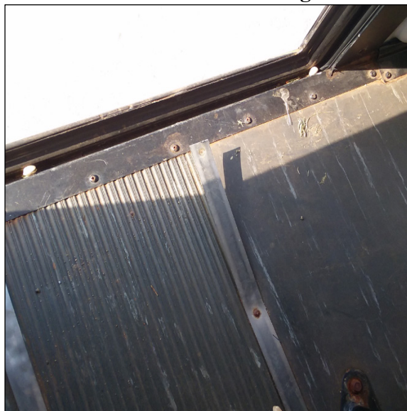
Broken Mat Lashing
