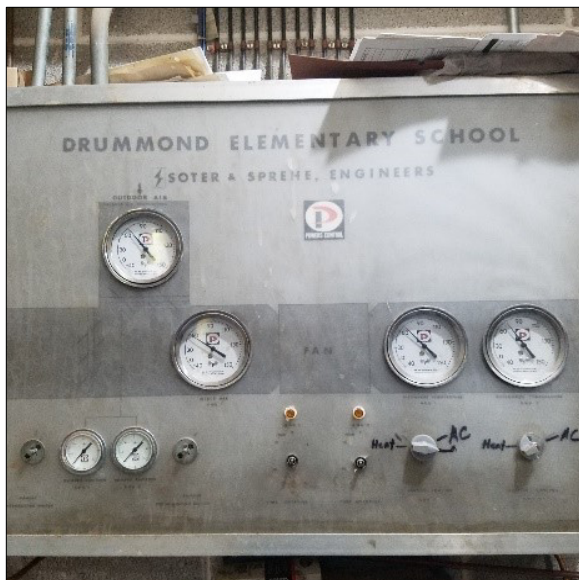
Exhibit 4-32 Outdated Multizone HVAC Control Panel
