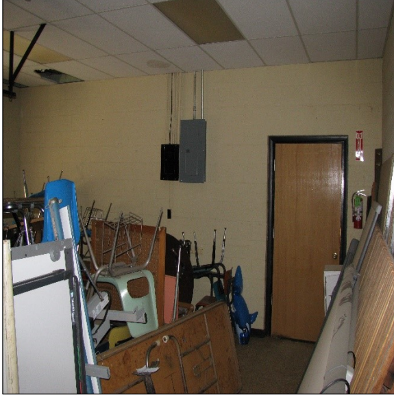
Electrical panels and Extinguisher Blocked
