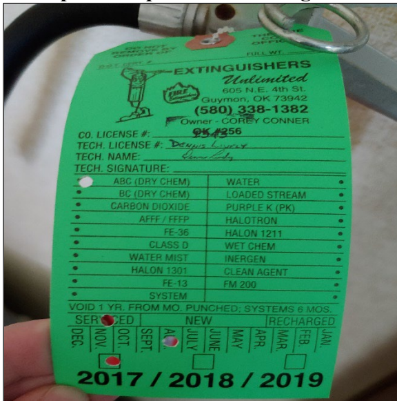
Expired Inspection on Extinguisher
