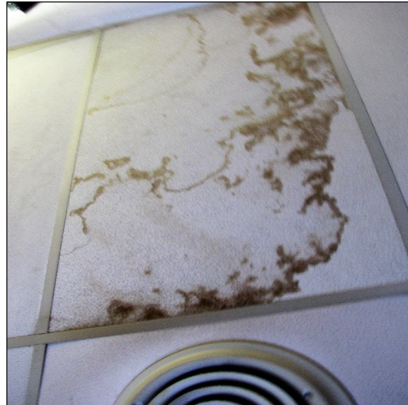
Stained Ceiling Tile Typical
