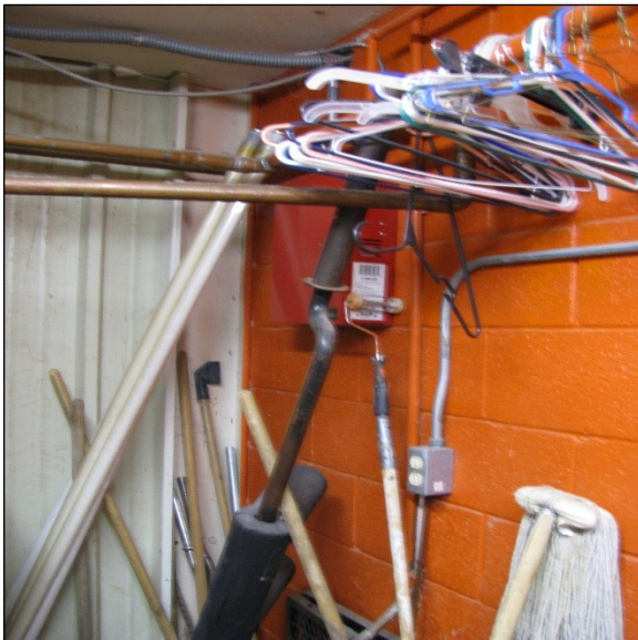
Blocked Fire Panel
