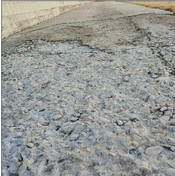
Crumbling Concrete Sidewalks*
