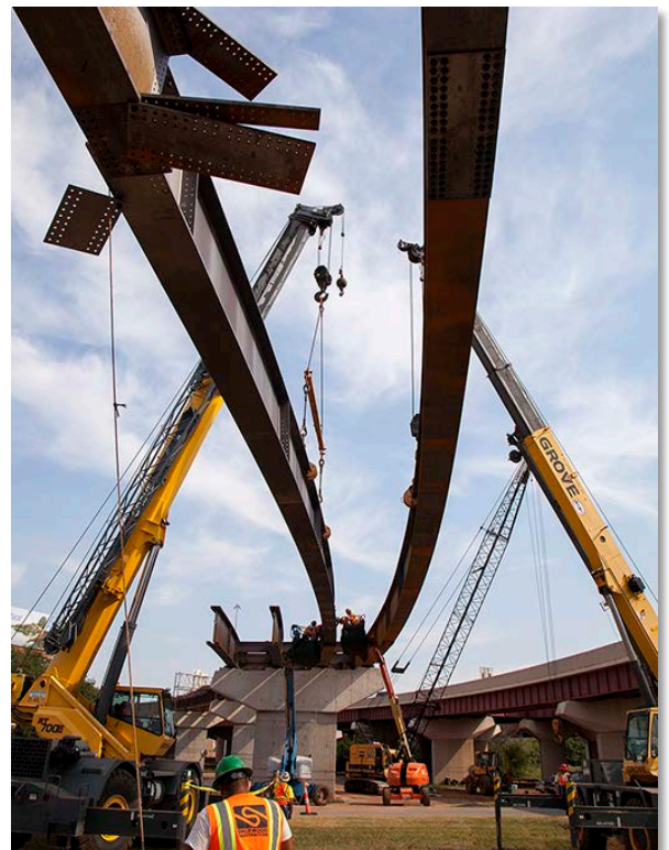
Figure 12: Crews hang beam for I-235 off-ramp to OKC Boulevard for the I-40 Crosstown Relocation in 2015
