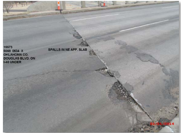
Figure 9: Douglas Boulevard Bridge - Deck repairs needed
