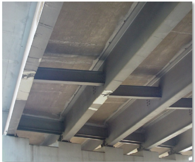
Figure 9: Anderson Road Bridge -Beam repairs needed
