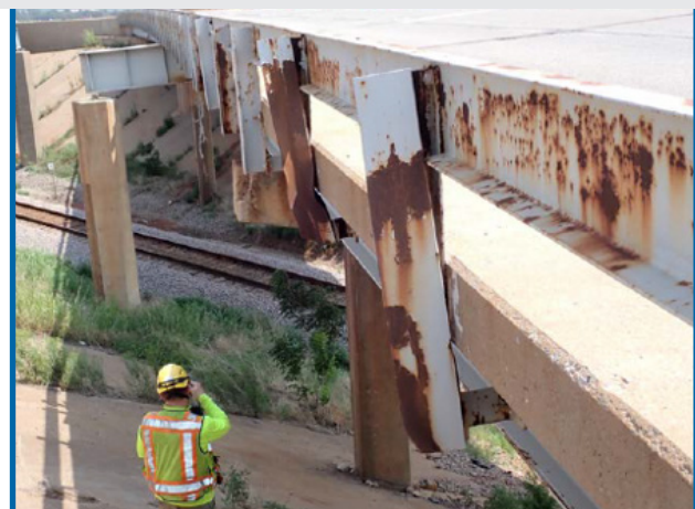
FIGURE 5. US-81 NB BRIDGE 16159: VIEW NORTH FROM THE SOUTH ABUTMENT SHOWING IMPACT-DAMAGED WEST RAILING POSTS, FAILED COATING, AND THE ADJACENT UPRR CORRIDOR.
