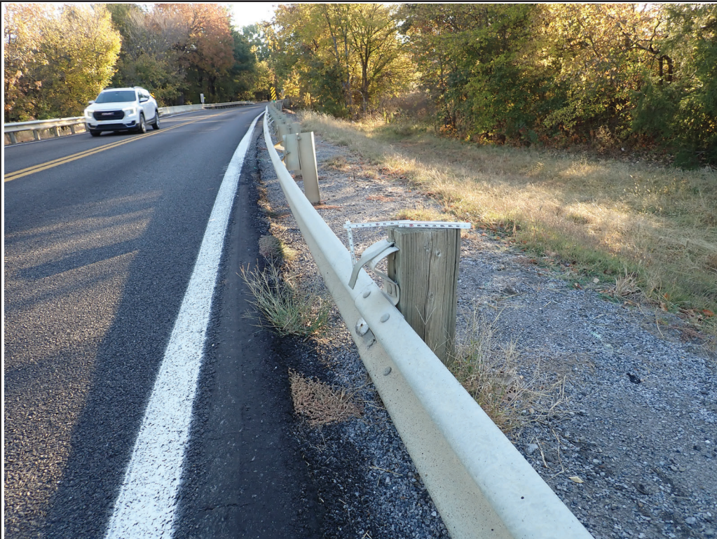
Photo 5 - Southwest approach guardrail; detached from the posts
