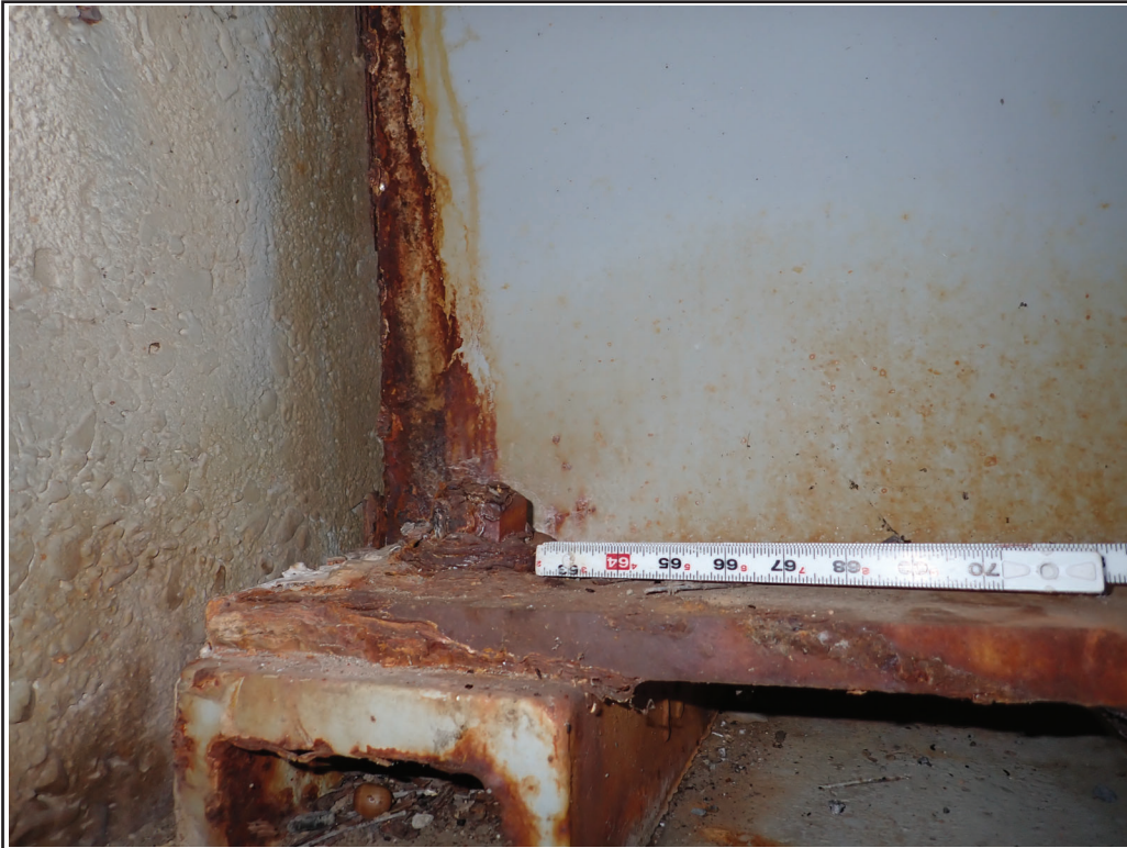
Photo 7 - East abutment, Bearing 6; laminar corrosion
