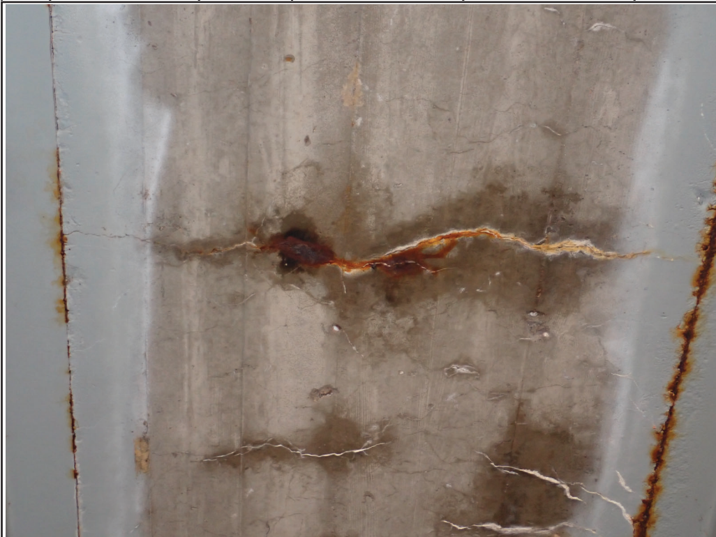
Photo 8 - Soffit, Bay 1; transverse cracking up to 1/32-in wide with efflorescence and corrosion staining
