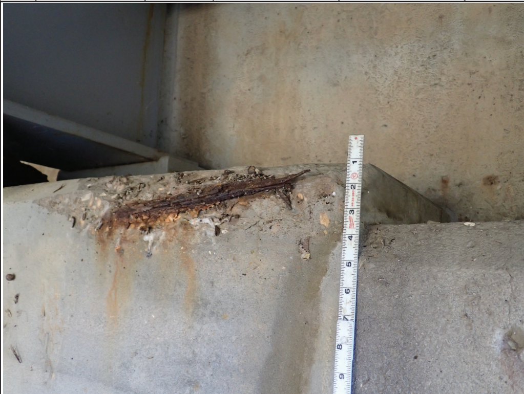
Photo 6 - East abutment, at Beam 2; spall 4-in H x 18-in L x 1 1/2-in D with exposed reinforcing
