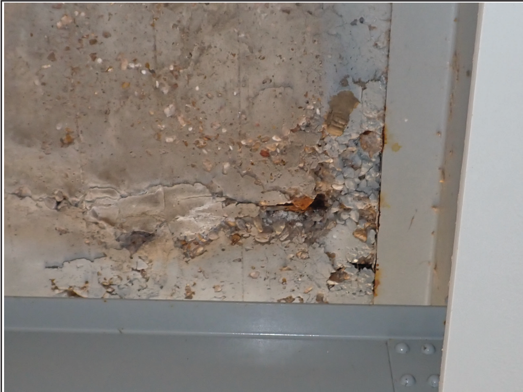
Photo 9 - Soffit, Bay 2; area of poor consolidation 24-in L x 30-in W x 3-in D with exposed reinforcing
