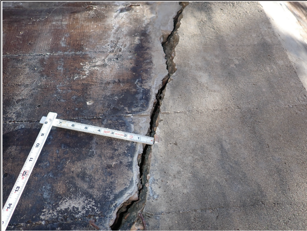
Photo 9 - Cell 5, east wall, near southeast wingwall connection; crack up to 3/4-in wide
