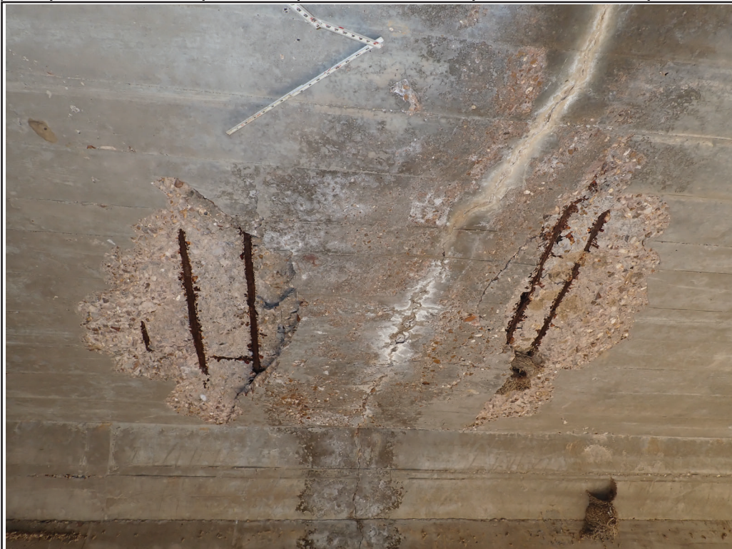
Photo 6 - Cell 4, top slab, near midspan; spalls up to 32-in L x 66-in W x 3-in D with exposed reinforcing
