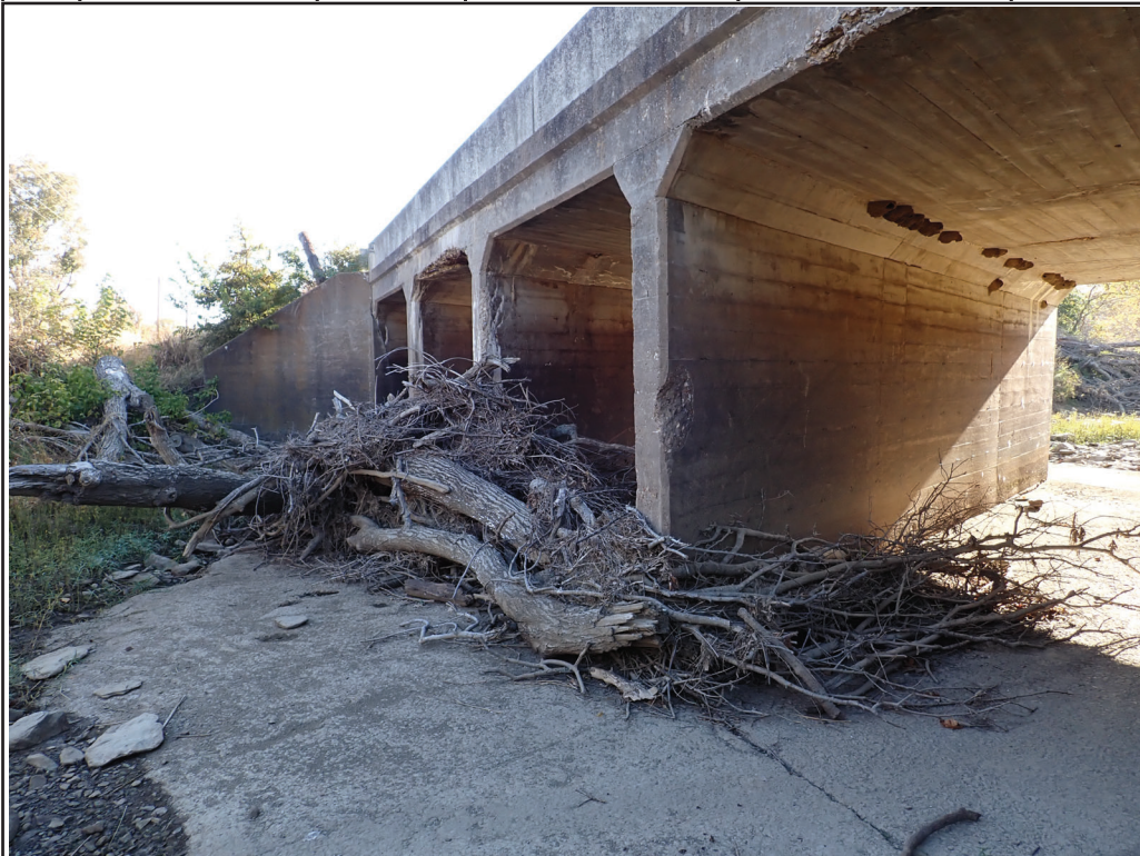
Photo 10 - Upstream end; timber debris accumulation up to 3-ft high
