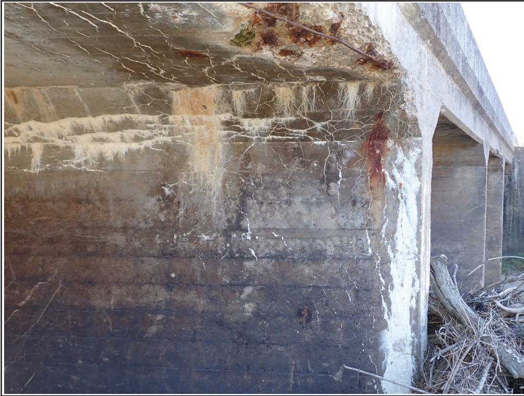
Photo 7 - Cell 4, west wall; hairline diagonal and longitudinal cracking with efflorescence buildup
