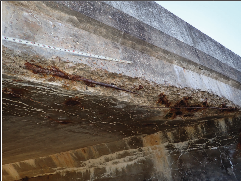
Photo 8 - Cell 4, north end; spall 24-in L x 84-in W x 3-in D exposed corroded reinforcing
