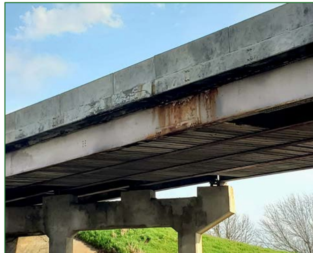
Figure 5. Existing Bridge Corrosion
