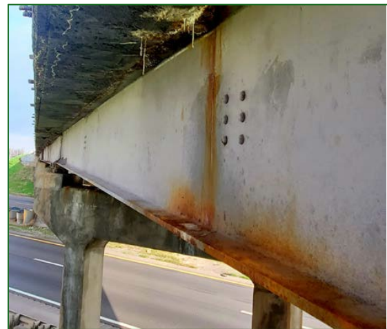
Figure 4. Existing Bridge Corrosion
