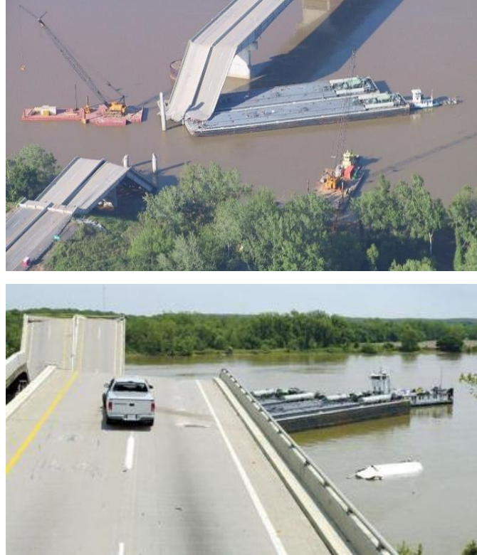
Figure 3: I-40 Bridge Collapse on May 26, 2002
