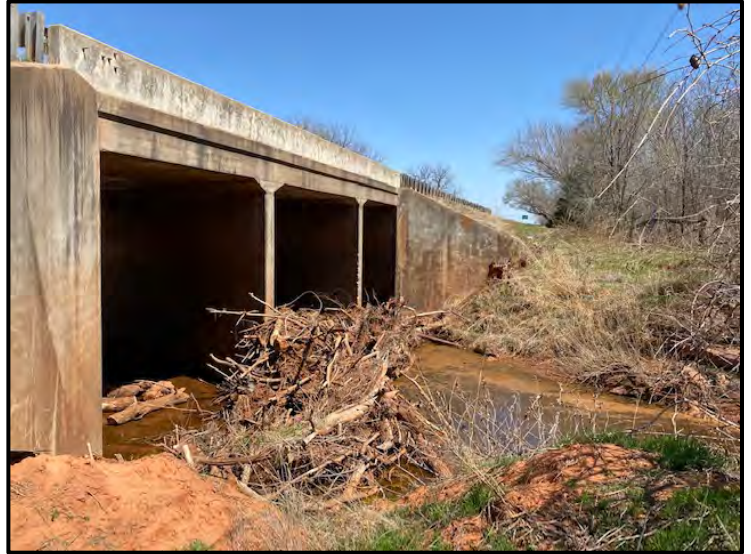
Photograph 27: Structure 8 (NBI: 12596) over R4SBA-01 (Spring Creek), migratory bird nests present.
