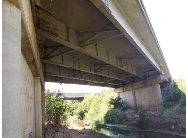
Photograph 16: Facing south toward debris deposit beneath west-bound I-40 bridge over FS-2.
