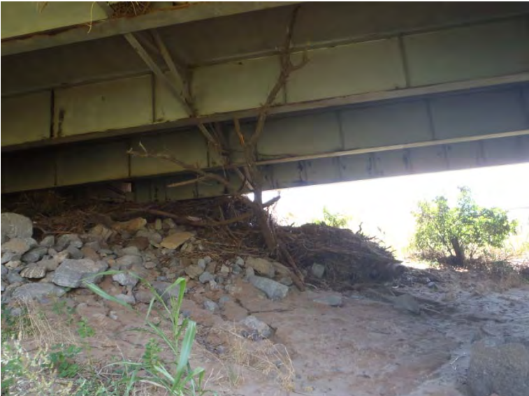
Photograph 15: Facing south toward debris deposit beneath west-bound I-40 bridge over FS-2.
