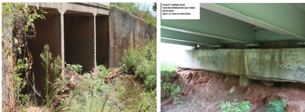
Figure 12: Deterioration of Structures
