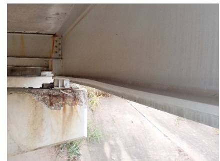
The bottom flange exhibits local deformation up to 1/4 inch due to impact damage on Span 2
