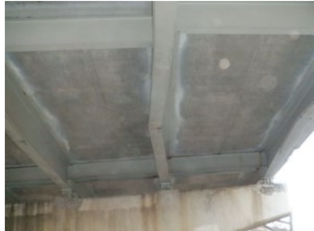
Bridge beam damage after the January 2023 bridge strike.
