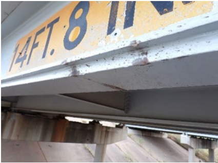
Signs of recent impact damage (scrapes and gouges) in the bottom flange
