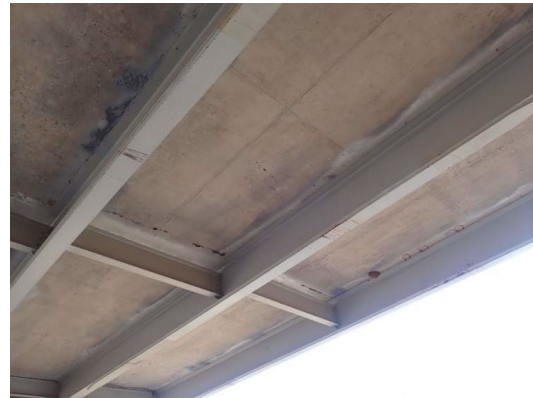
Signs of recent impact damage (scrapes) along the bottom flanges.
