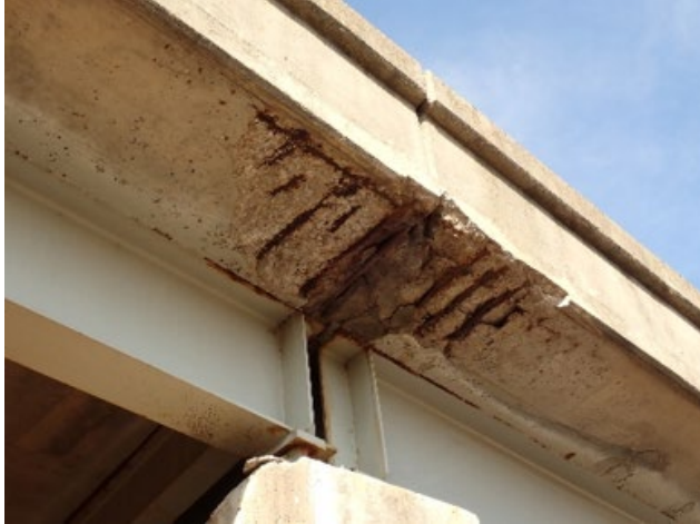
29-inch wide by 4-foot long by up to 2-inch deep spall with several exposed and corroding reinforcing steel bars and adjacent delaminations at pier 1
