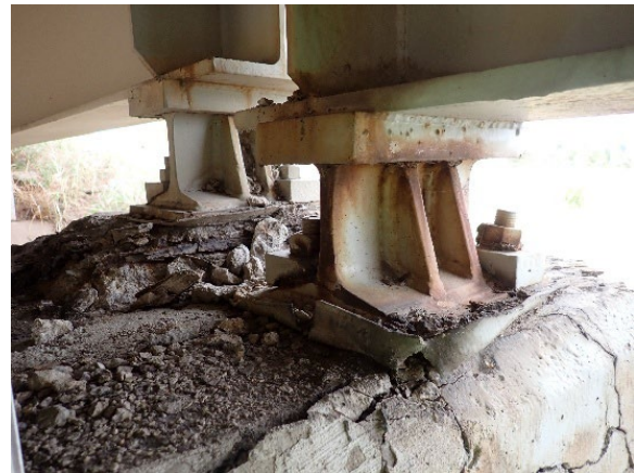
Wide cracking throughout pier 2 cap with spalls around and below bearings
