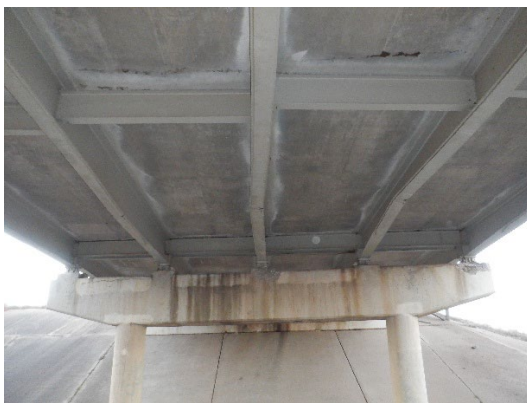
Bridge beam damage from the January 2023 bridge strike.
