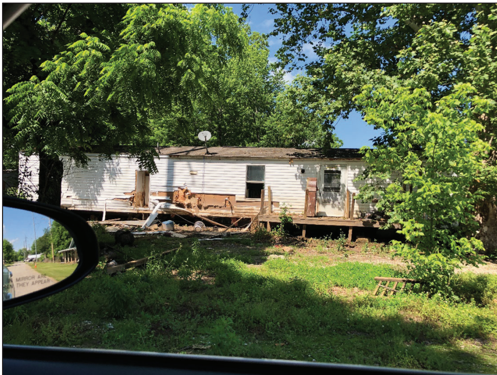
Photo 14: Abandoned home in disrepair in Webbers Falls.
