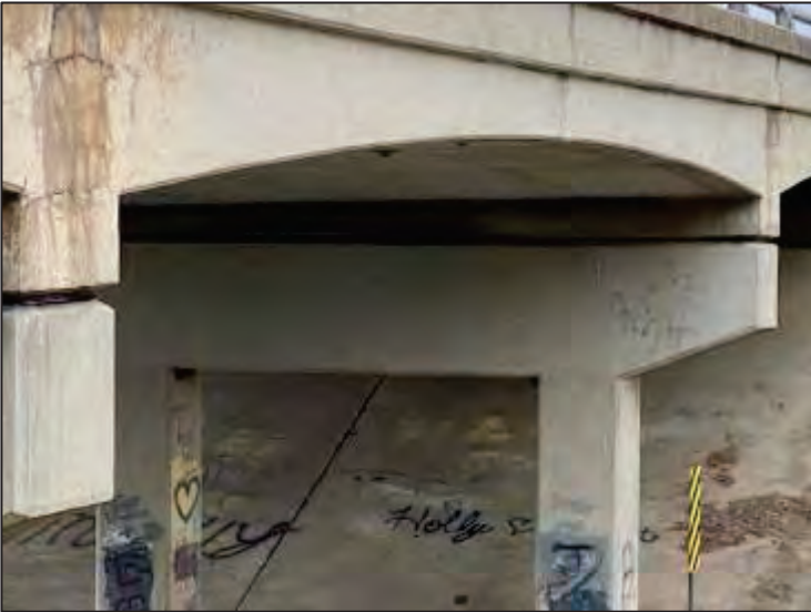
Photograph 33: NBI: 16945 (Structure 15) over SH-10, cliff swallow nests present.
