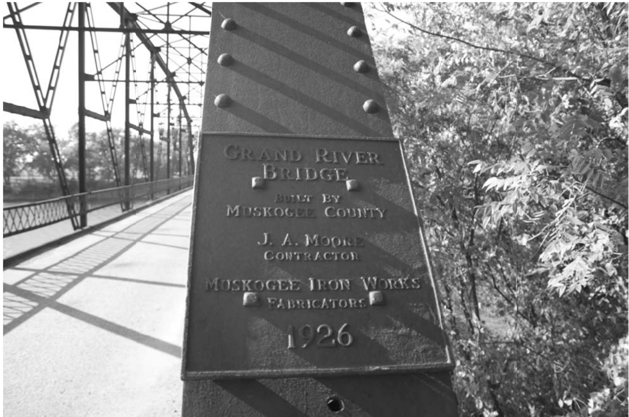
20. DETAIL VIEW OF BRIDGE STAMP READING “GRAND RIVER BRIDGE; BUILT BY MUSKOGEE COUNTY; J.A. MOORE CONTRACTOR; MUSKOGEE IRON WORKS FABRICATORS; 1926,” LOOKING NORTHWEST
