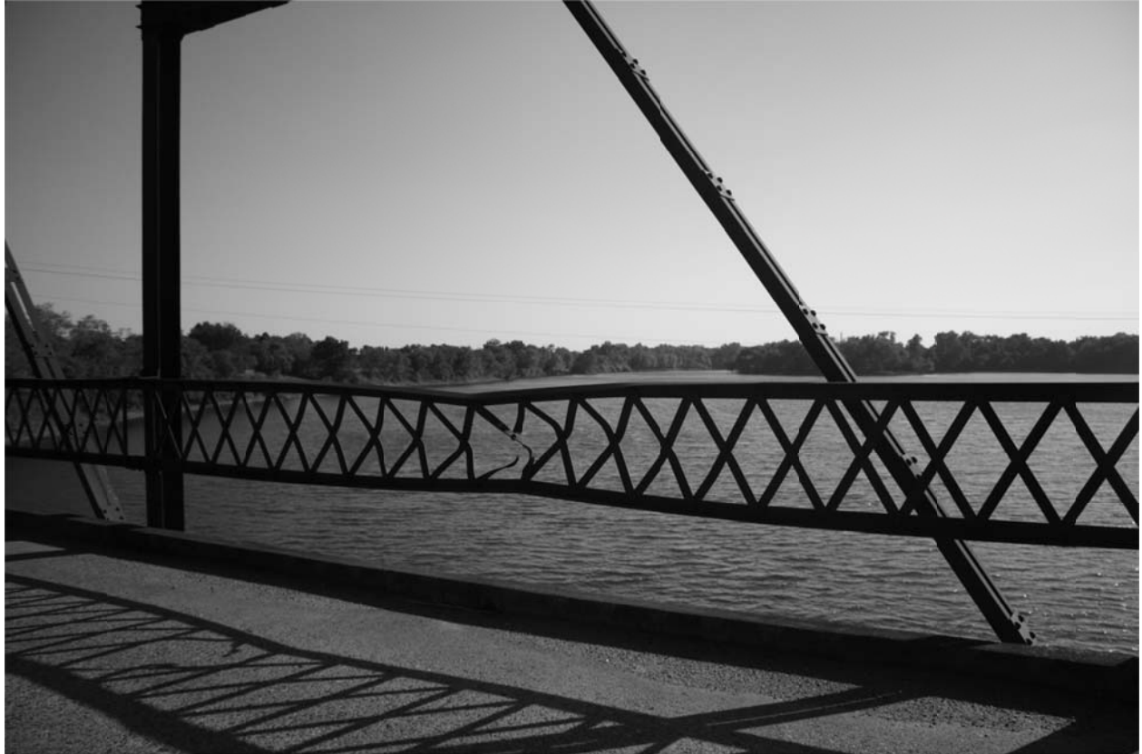
14. DETAIL VIEW OF LACING DAMAGE, LOOKING SOUTH
