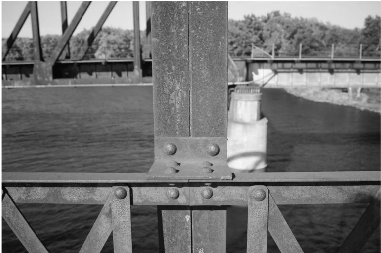
17. DETAIL VIEW OF GUSSET PLATE JOINING RAIL AND VERTICAL MEMBER, LOOKING NORTH
