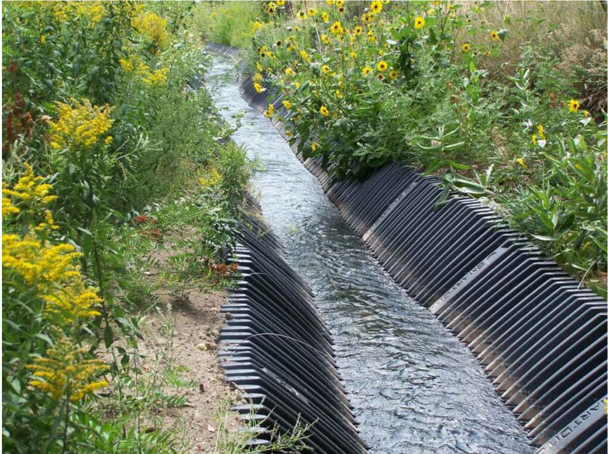
[Smart Ditch installed in ground]
