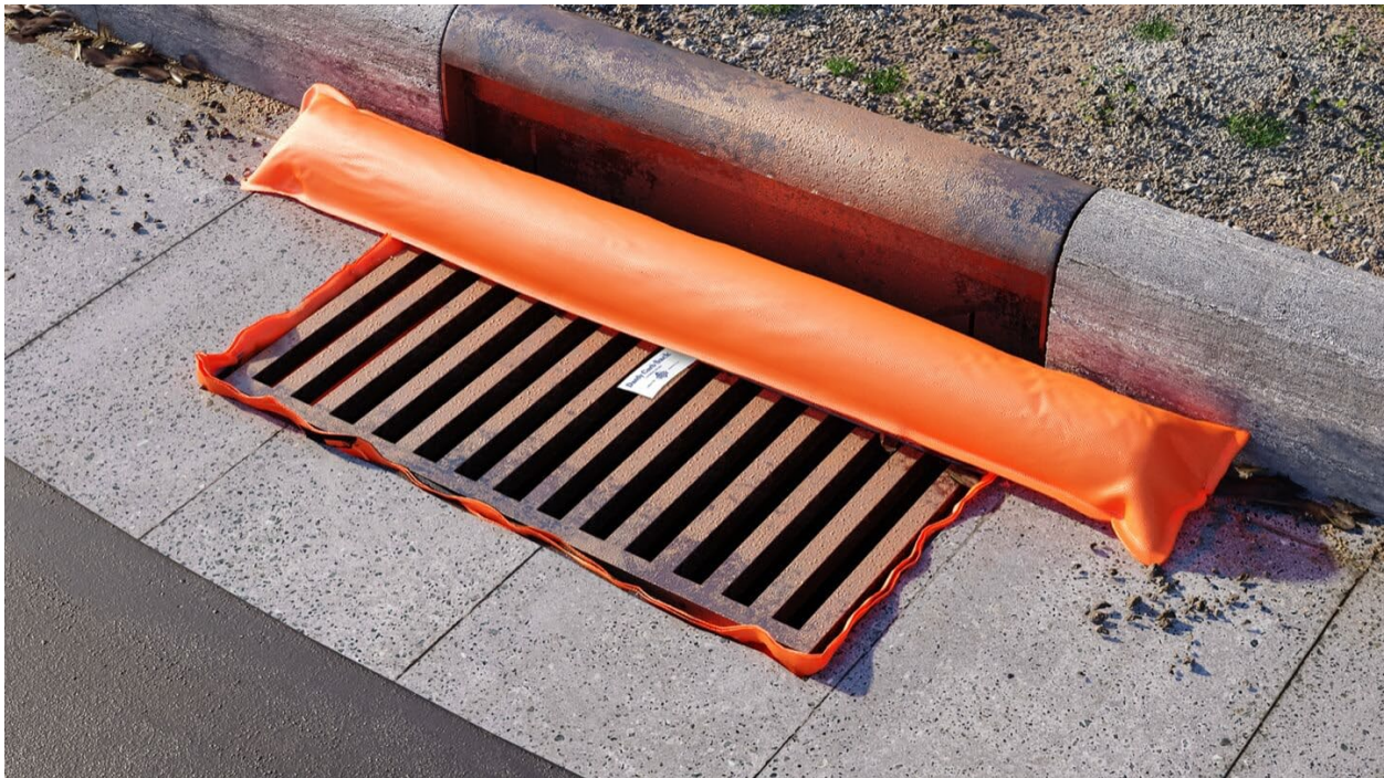
[Curb sediment bag installed on curb drain]
