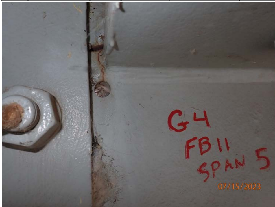
Photograph 48 - Looking north at the termination of the horizontal splice for girder 4, span 5 near floor beam 11. Note: 1-inch-long crack in lower web at horizontal splice termination has been arrested with a drilled hole.
