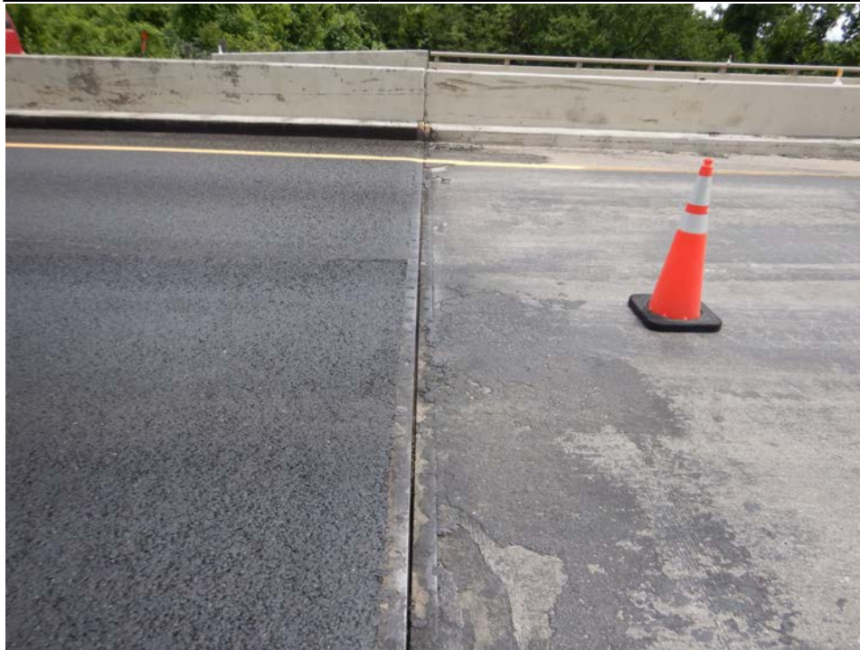
Photograph 39 - Looking south along the strip seal expansion joint in the westbound roadway at the east abutment. Note: joint is closed.
