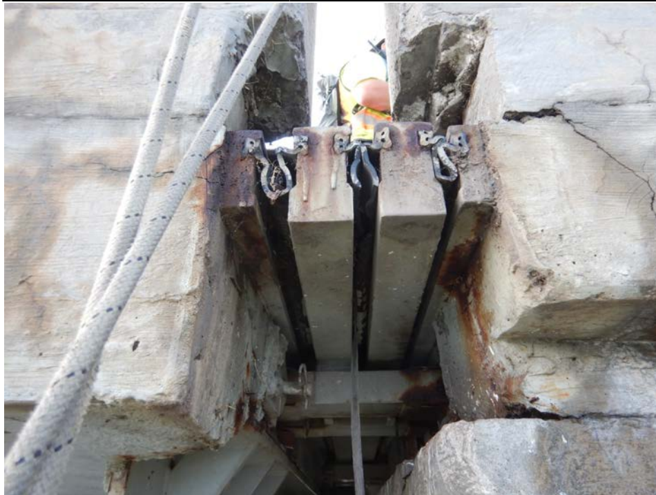
Photograph 28 - Looking south at the north end of the modular joint at pier 3. Note: elastomeric seals are split.
