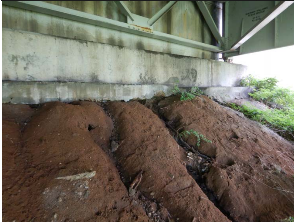
Photograph 80 - Looking southeast at the east embankment under the eastbound lanes. Note: erosion gullies from deck drainage leaking through the expansion joint is undermining the repair to encase the exposed piles.
