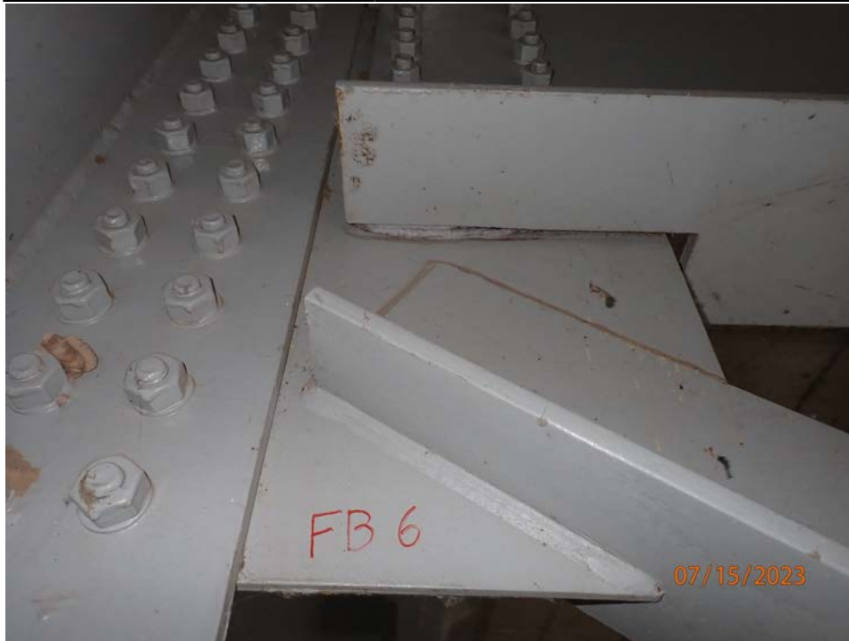
Photograph 69 - Looking east at floor beam 6, span 4 connection to girder 4. Note: 1/2-inch-thick painted over pack rust between floor beam and connection plate.
