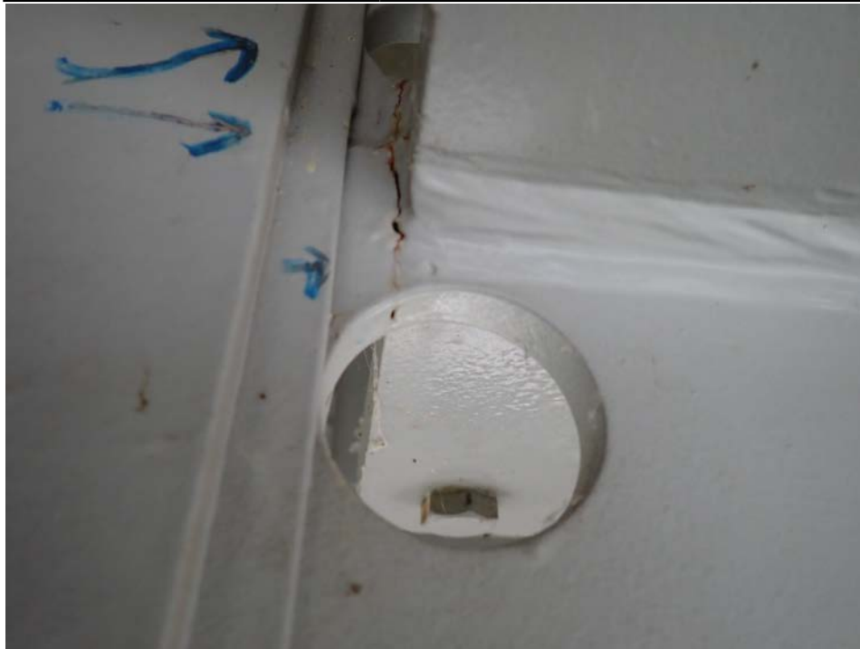
Photograph 42 - Looking north at the termination of the horizontal splice for girder 2, span 4 near floor beam 5. Note: cracks in upper and lower web of girder at horizontal splice termination have been arrested by drilled holes.
