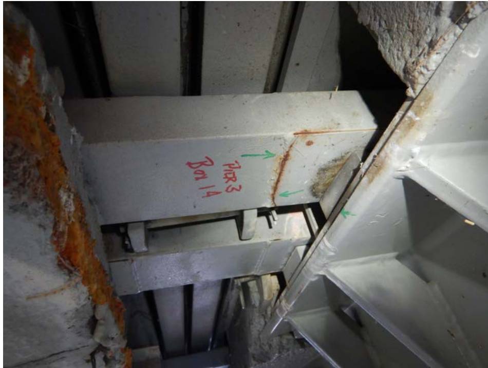
Photograph 25 - Looking northeast at the underside of the pier 3 modular joint at support box 14. Note: stainless steel plate welded to support bar 1 at the east bearing box has fractured near the west weld.
