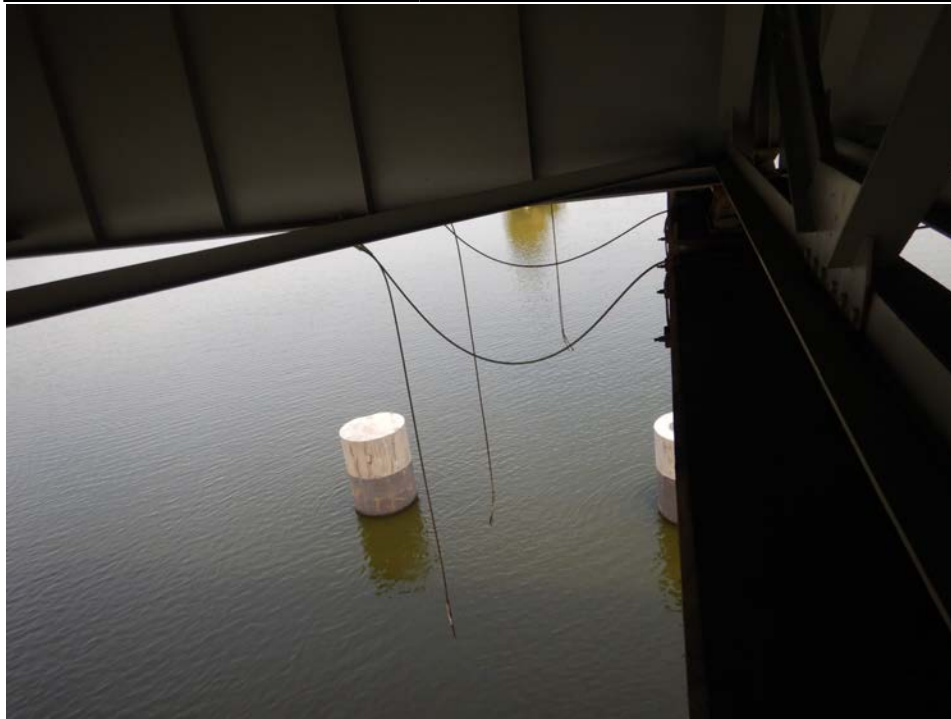
Photograph 85 - Looking north along pier 6 from girder 1. Note: seismic restraint cables are broken.
