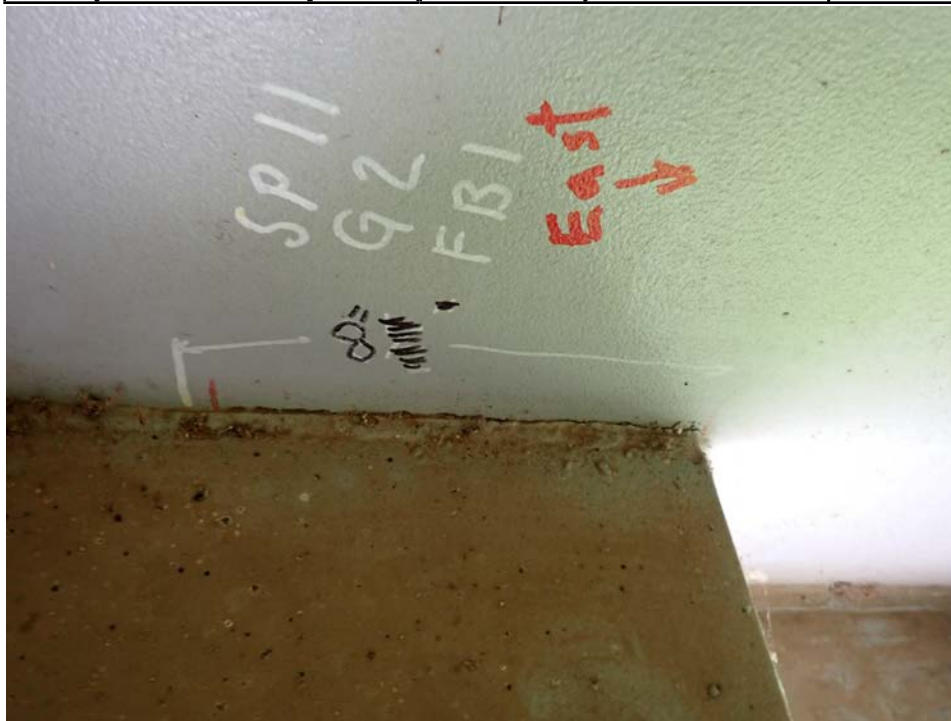
Photograph 75 - Looking north at girder 2, span 11 at floor beam 1. Note: cracked weld on gusset plate, 6 inches long, no change from previous inspection.
