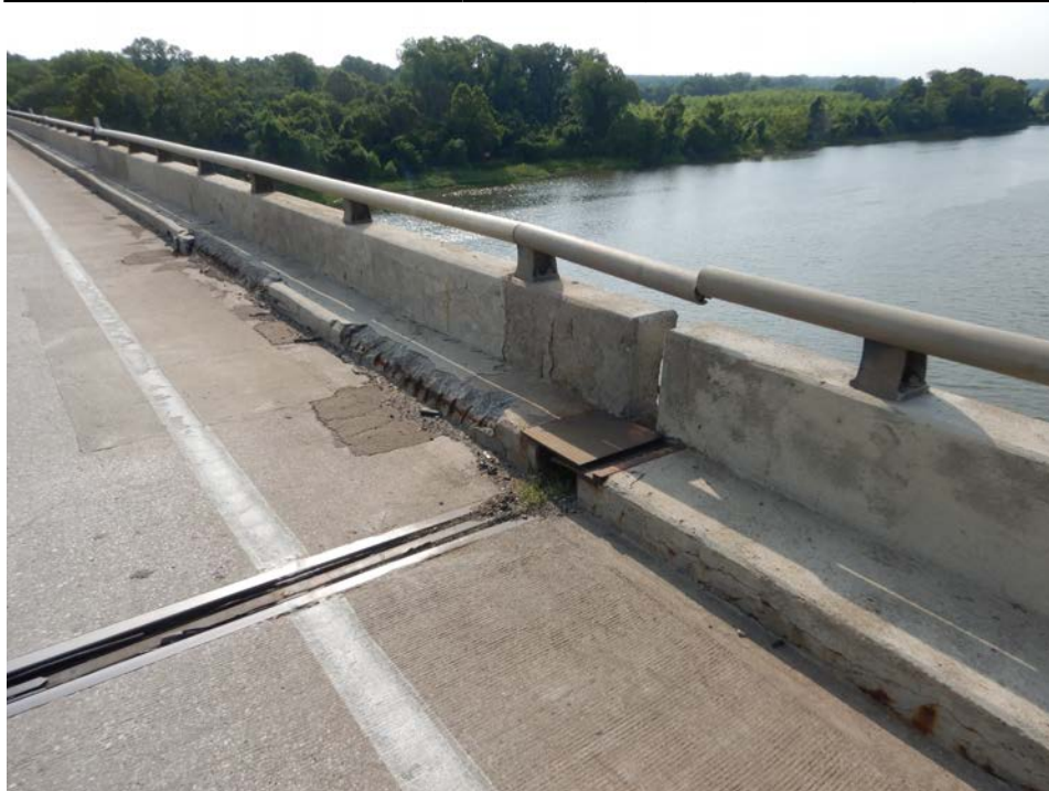
Photograph 8 - Looking southeast at the south bridge railing in over pier 6, span 7 near. Note: spalled curb and aluminum rail not spliced.
