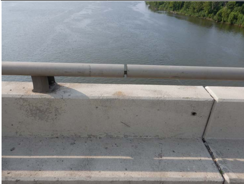
Photograph 9 - Looking south at the south bridge railing near floor beam 1, span 5. Note: rail is connected by a bar.
