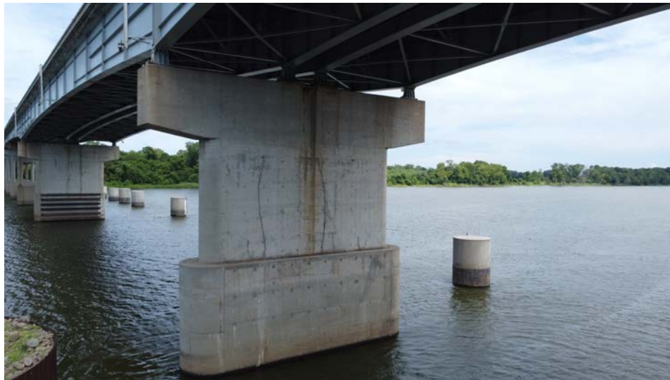
Photograph 87 - Looking southeast at pier 4. Note: sealed vertical and diagonal cracks in pier wall.
