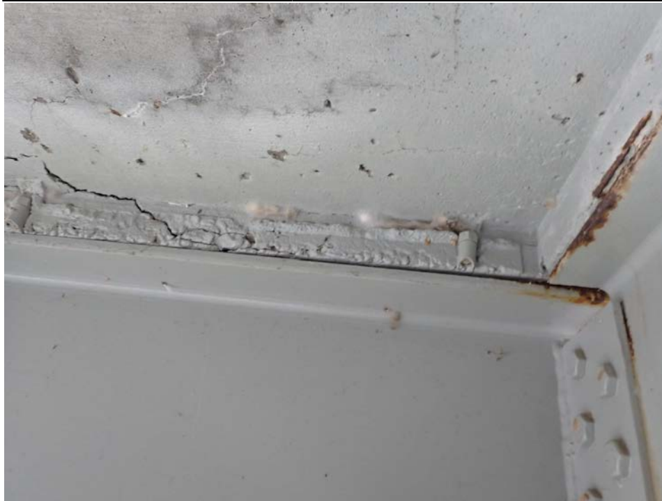
Photograph 17 - Looking north at stringer 3 near floor beam 11, span 5. Note: deck lifting above stringer (common at deck control joint locations).
