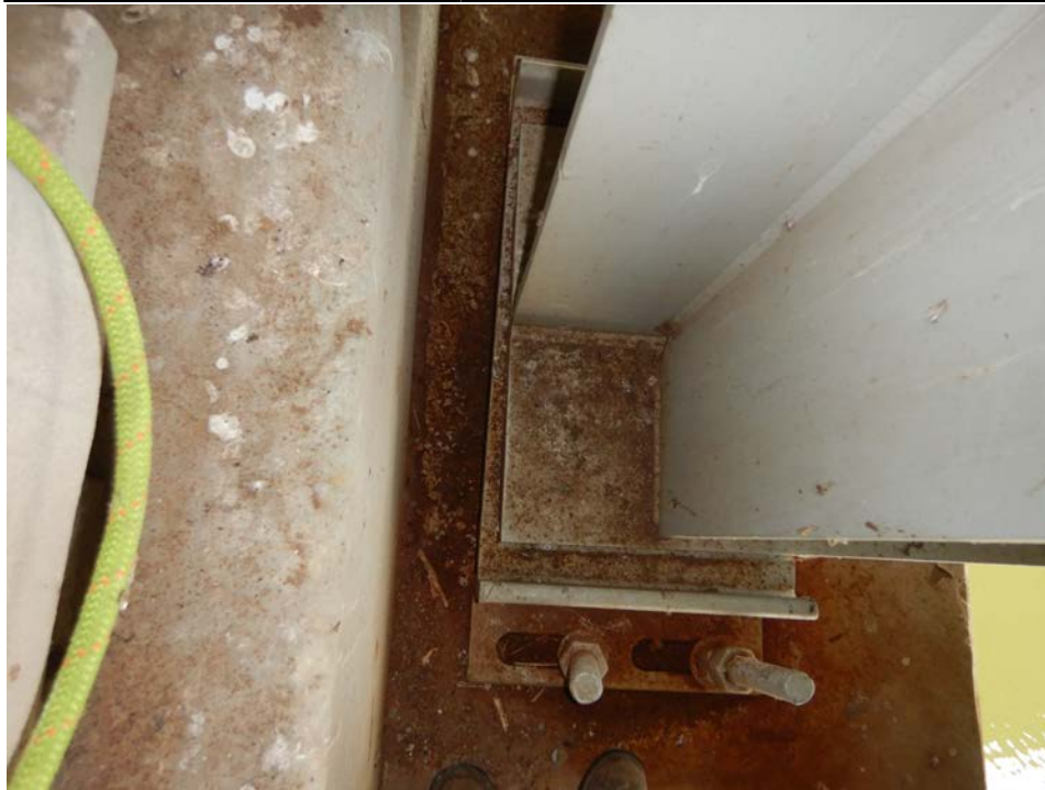
Photograph 91 - Looking down at the south edge of the girder 3, span 4 at the pier 3 bearing. Note: bearing assembly is not parallel with the girder (offset 5/16 inch over a 16 5/8-inch length).
