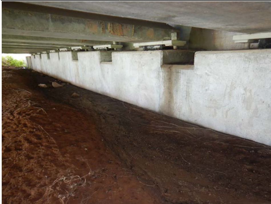
Photograph 82 - Looking southwest at the west abutment. Note: few horizontal and vertical cracks exist in the breastwall and back wall. Evidence of water leakage exists on the breastwall.
