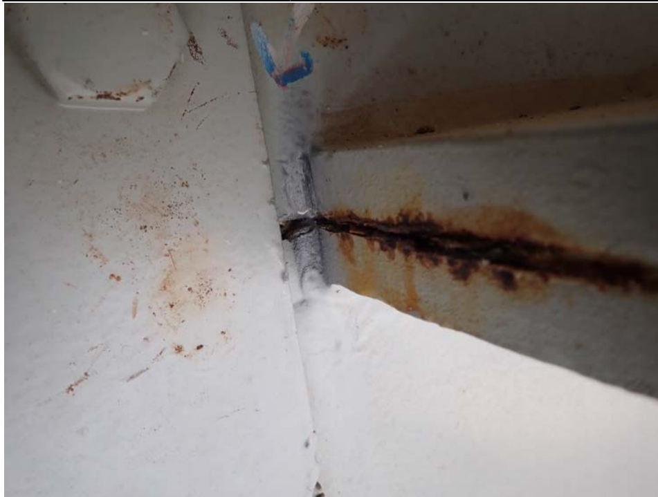
Photograph 51 - Looking south at the termination of the horizontal splice for girder 3, span 6 near floor beam 3. Note: paint crack in upper web at horizontal splice.
