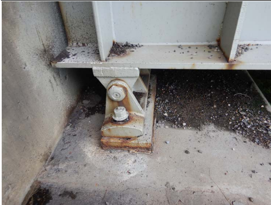
Photograph 93 - Looking south at the girder 4 expansion bearing at the east abutment. Note: bearing rotated 11 degrees east. Bearing has been reset 4 inches west in the past. Bottom flange is 1 1/2 inches from the backwall. All bearings at east abutment are similar.
