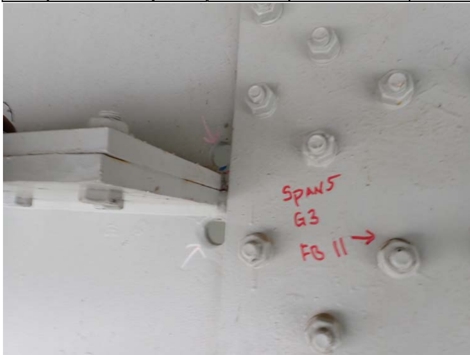
Photograph 46 - Looking southeast at the termination of the horizontal splice for girder 3, span 5 near floor beam 11. Note: 7/8-inch-long crack in upper web of girder at horizontal splice termination with drilled hole near crack termination.
