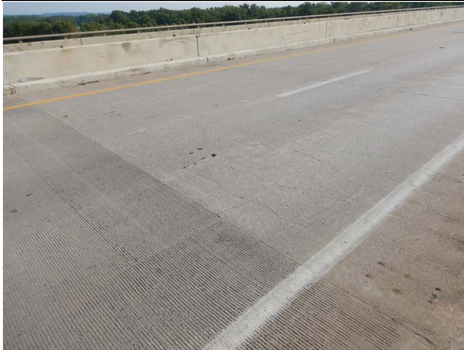
Photograph 14 - Looking northeast at the deck near floor beam 6, span 4. Note: transverse cracks in original portion of deck near the new deck section.
