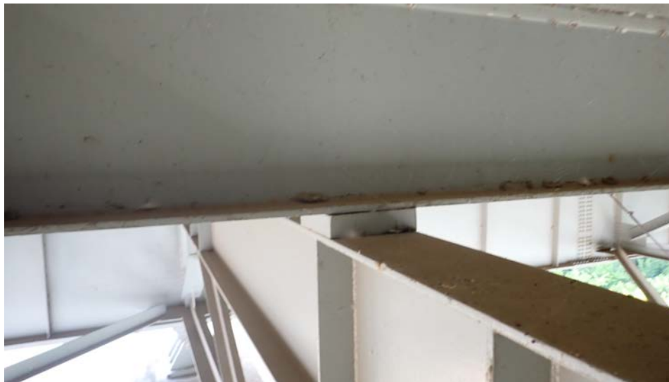
Photograph 64 - Looking northeast at stringer 3, span 10 over the floor beam 0. Note: all 4 anchor bolts are missing.
