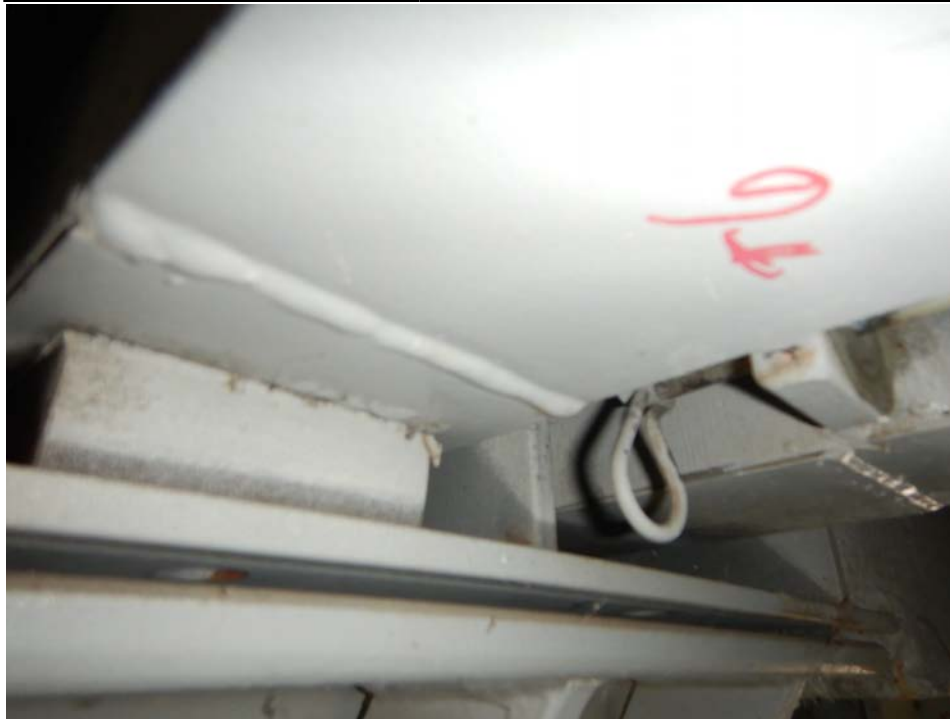
Photograph 23 - Looking southeast at the underside of the pier 3 modular joint at support box 6. Note: bearing block for support bar 1 is missing at the east support box.. Stainless steel sliding surface is painted.
