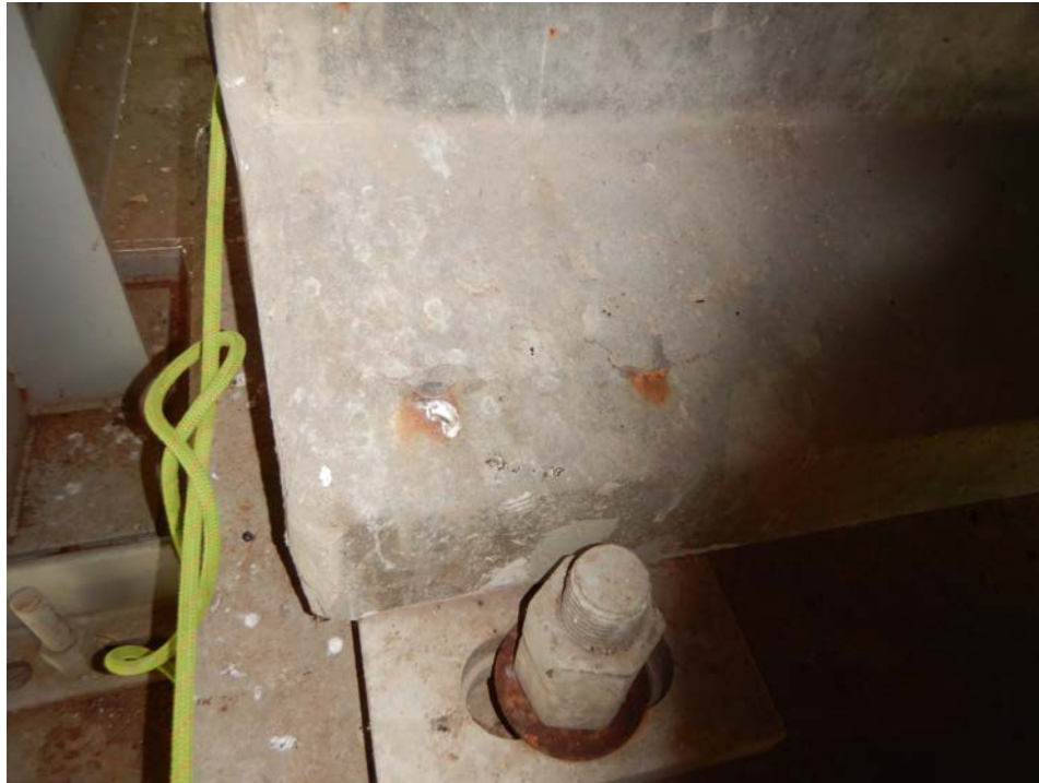
Photograph 63 - Looking south at the bottom flange of prestressed concrete beam 6, span 3 at pier 3. Note: ends of mild steel anchors for sole plate are exposed.
