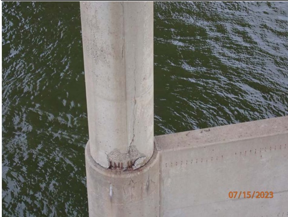
Photograph 84 - Looking east at pier 6 north column. Note: 5 square feet of spalling with exposed corroded reinforcement at the base of the column and a full height vertical crack of the column.
