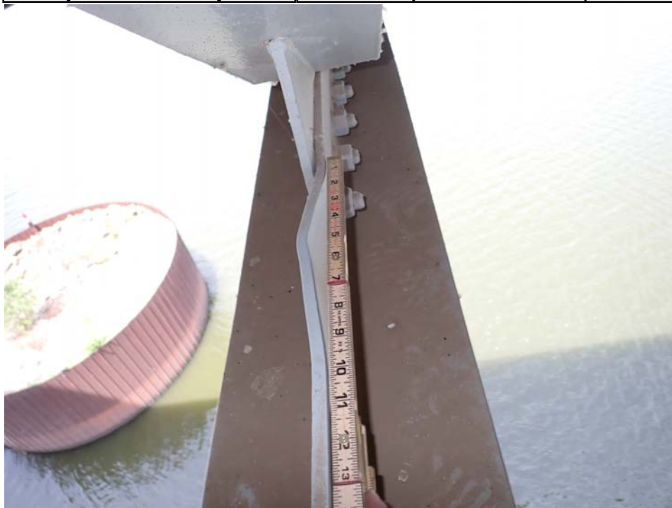
Photograph 68 - Looking north at the center girder bottom gusset plate for floor beam 2, span 6 between girders 3 and 4. Note: vertical leg of T-section is kinked west 11/16 inch over 10 inches.
