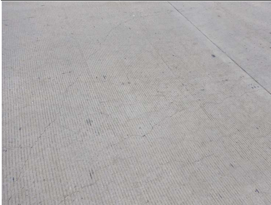
Photograph 13 - Looking south at the deck in the westbound lanes over pier 2. Note: diagonal and longitudinal cracks.
