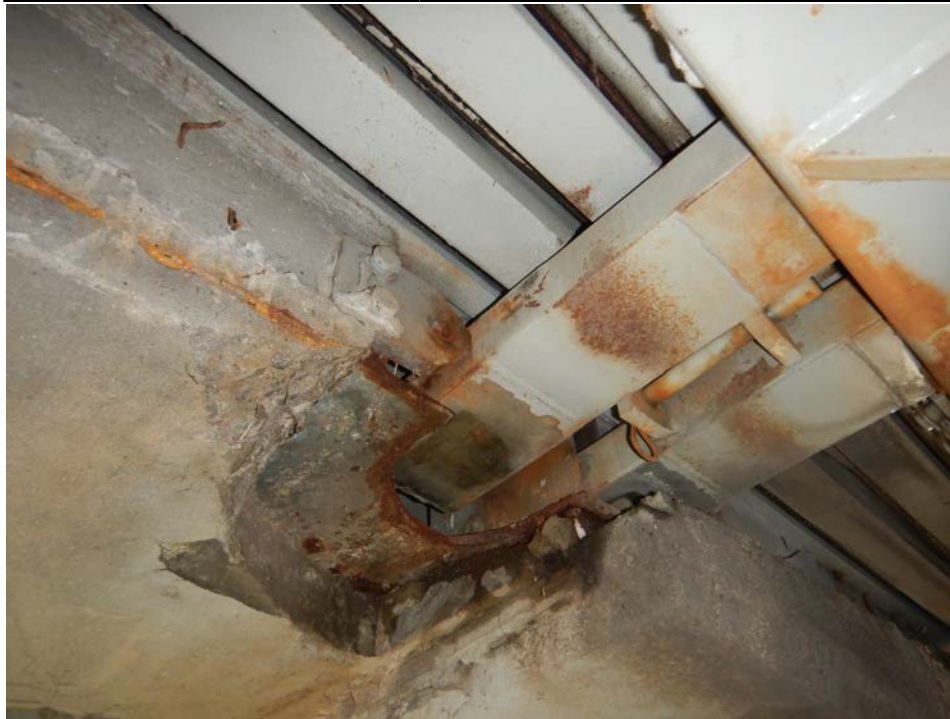
Photograph 27 - Looking northwest at the underside of the pier 3 modular joint at support box 16. Note: bottom plate of the west support box has fractured away and the west end of support bar 1 is unsupported.
