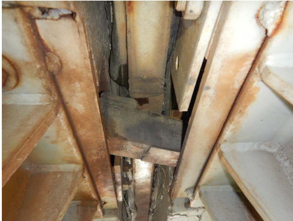
Photograph 29 - Looking south at the underside of the pier 6 modular joint at support box 2. Note: transverse separation beam fractured. Support bar has broken away from the transverse separation beam.
