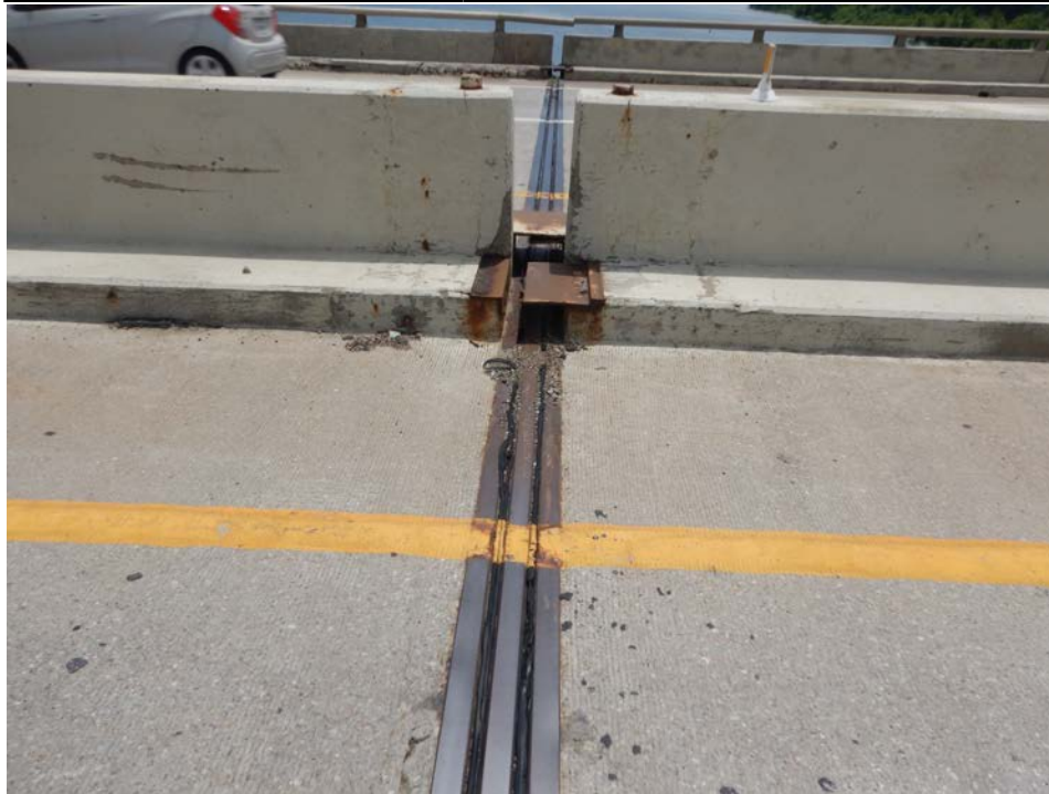
Photograph 41 - Looking south at the median at pier 6. Note: sliding plate for joint is missing.
