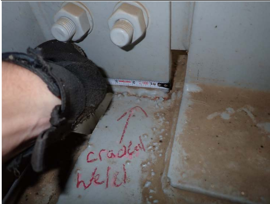
Photograph 57 - Looking west at the connection stiffener for girder 3, span 6 at floor beam 3. Note: 3-inch-long crack in the weld to the lateral bracing gusset plate.
