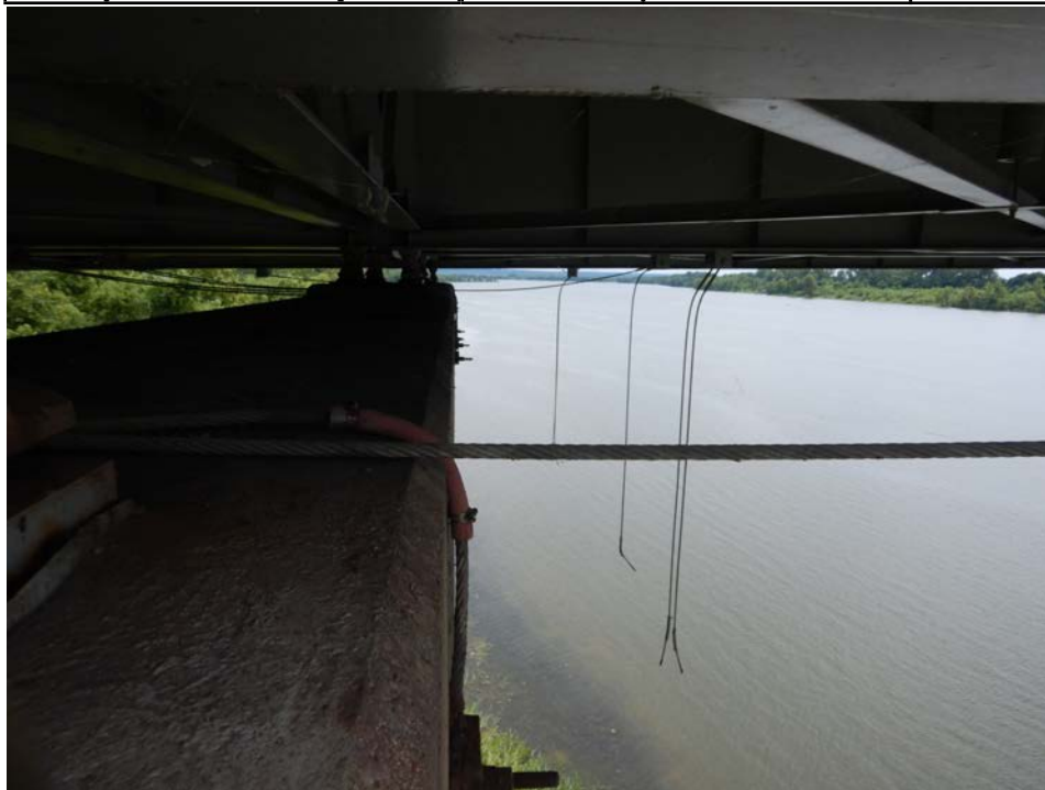
Photograph 86 - Looking south along pier 10 from girder 1. Note: both seismic restraint cables are broken at girders 1 and 3, and one is broken at girder 2.
