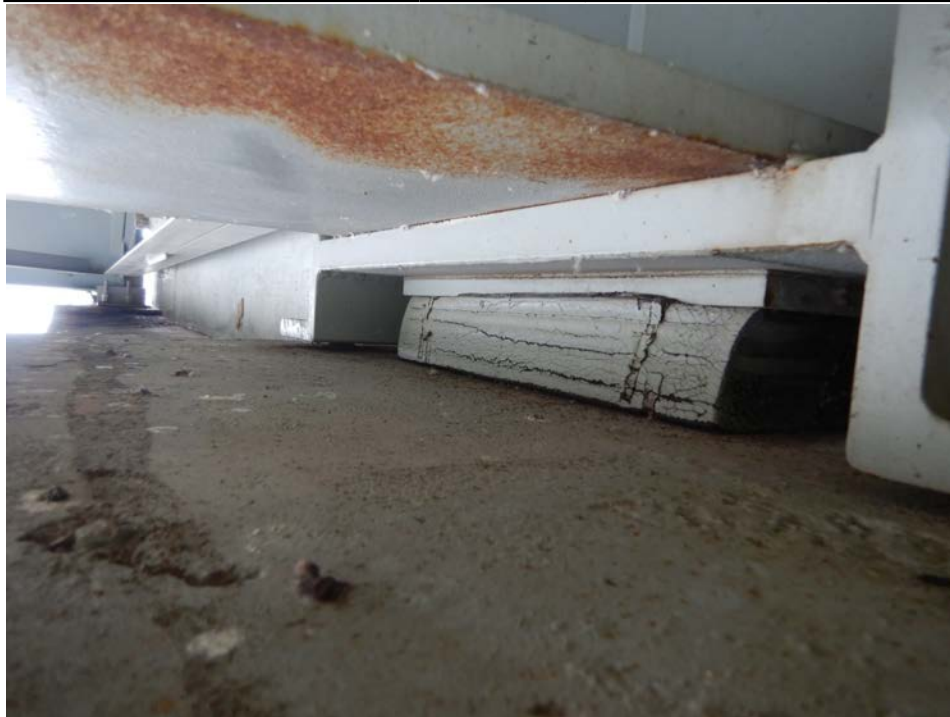
Photograph 90 - Looking southwest at the elastomeric expansion bearing for girder 2, span 4 at pier 3. Note: elastomeric bearing is bulging over the edge of the sole plate. Bearing is sheared in expansion 3/4 inch and the bottom east edge has lifted from the pier seat.
