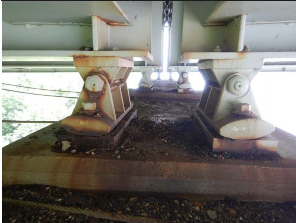
Photograph 92 - Looking south at the girder 3 expansion bearings at pier 10. Note: bearings are rocked slightly in expansion at 90F. Pack rust exists between the rocker and masonry plate.
