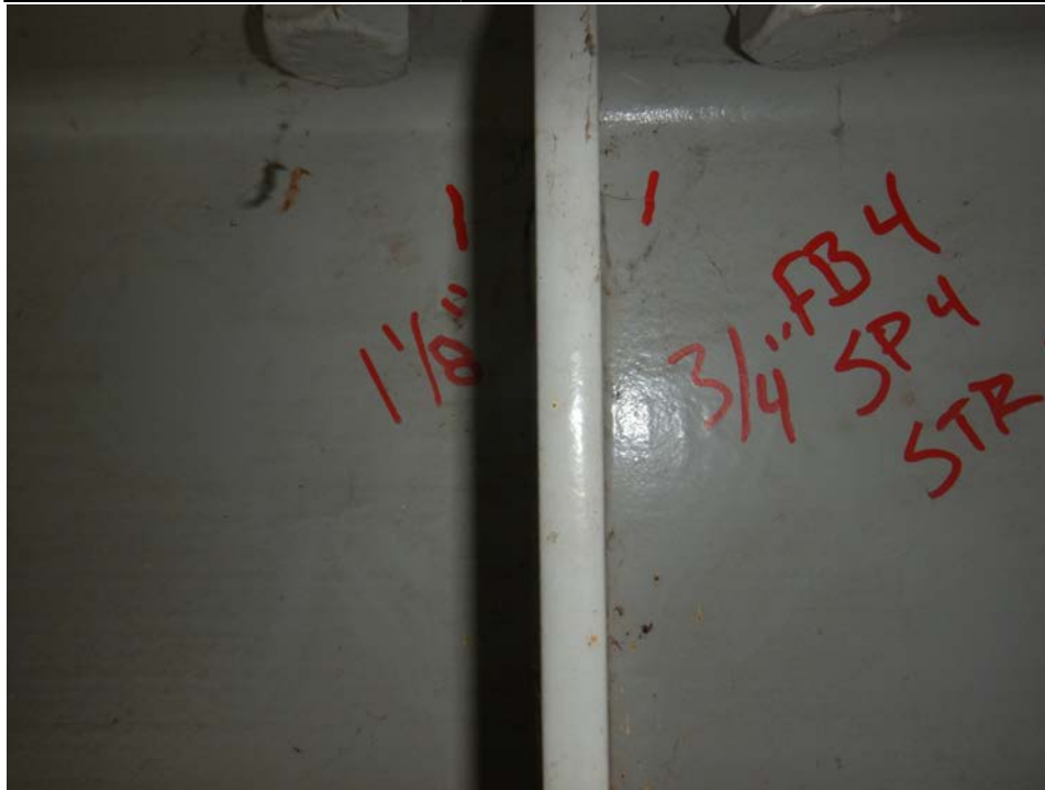
Photograph 67 - Looking west at floor beam 4 at stringer 2 in span 4 . Note: horizontal crack extends 3/4 inch north and 1 1/8 inches south of the stiffener.
