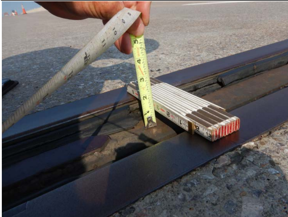
Photograph 31 - Looking northwest along the modular expansion joint in the south eastbound lanes at pier 6. Note: repair of the transverse separation beam has failed and beam has dropped 1 inch.
