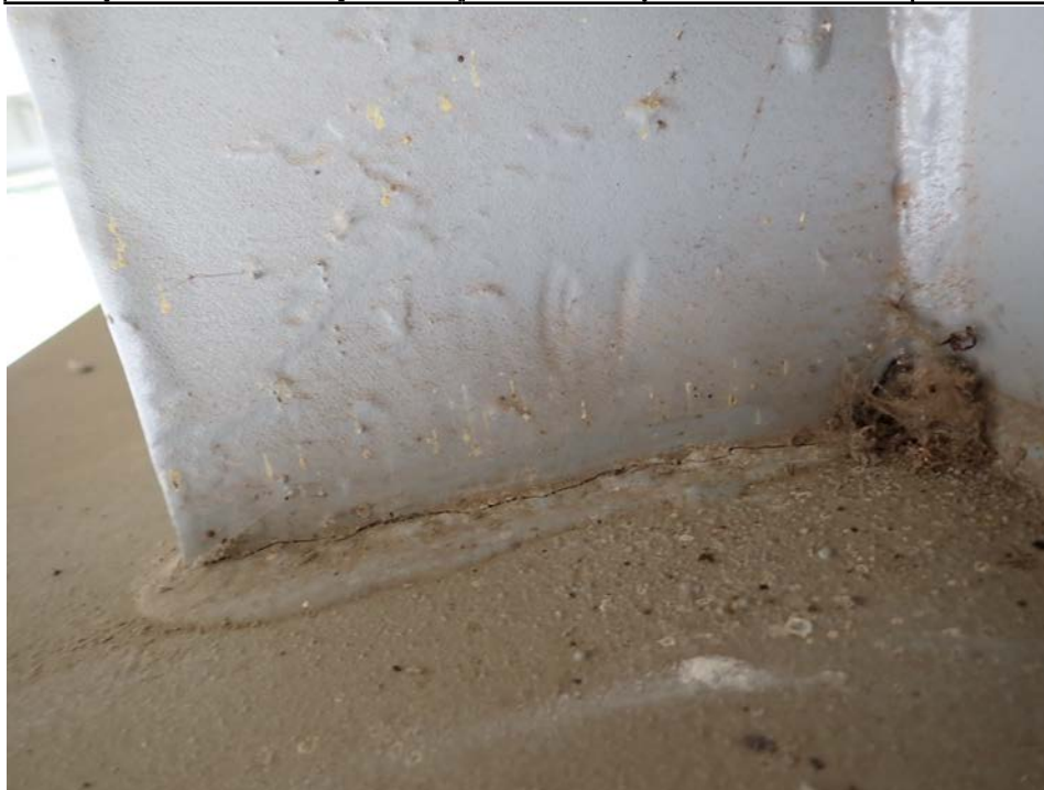
Photograph 58 - Looking east at the connection stiffener for girder 3, span 6 at floor beam 4. Note: paint crack at the interface with the girder bottom flange.
