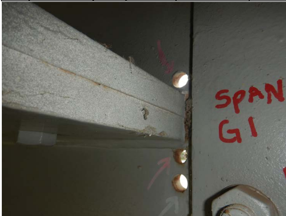
Photograph 44 - Looking south at the termination of the horizontal splice for girder 1, span 5 near floor beam 11. Note: 3/4-inch-long and 1 1/4-inch-long cracks in upper and lower web of girder at horizontal splice termination have been arrested by drilled holes.
