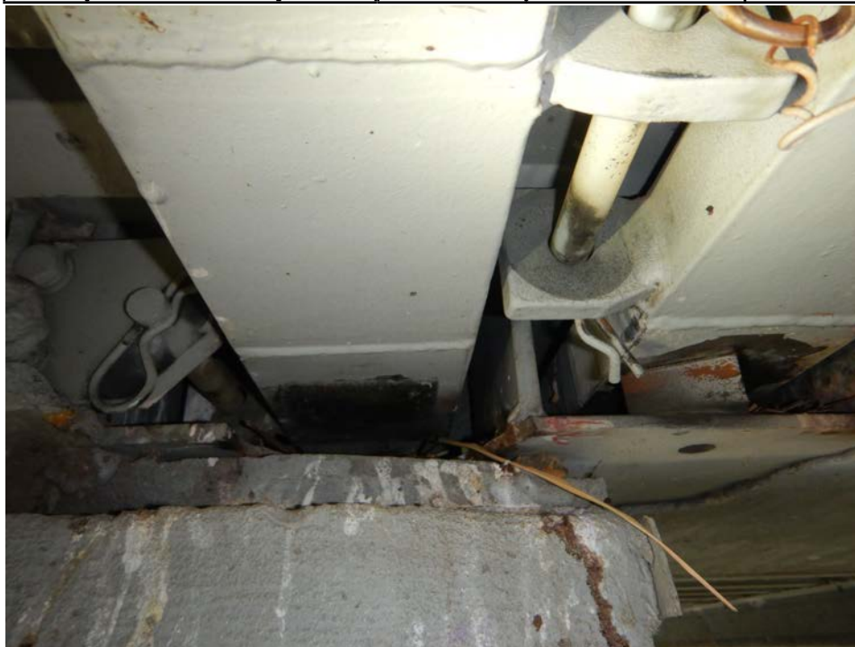
Photograph 20 - Looking west at the underside of the pier 3 modular joint at support box 3. Note: bottom plate of support box has fractured and west end of support bar 1 is unsupported. Bearing block for support bar 2 is dislodged. Stainless steel sliding surface is painted.
