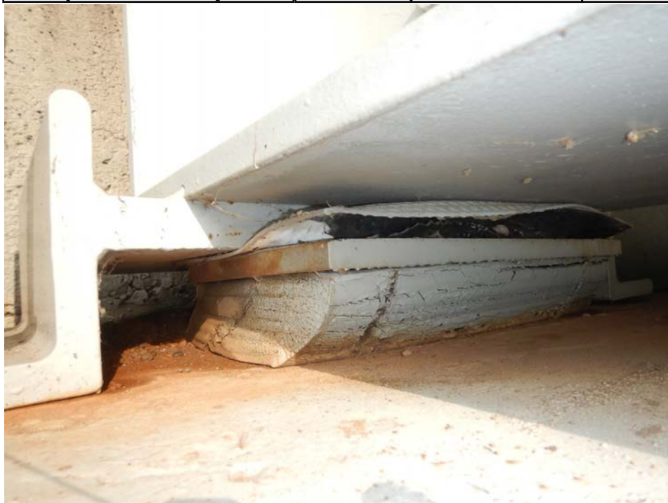
Photograph 88 - Looking northwest at the elastomeric expansion bearing for girder 1, span 4 at pier 3. Note: bearing split at northeast corner and debonded from sole plate at southeast corner. PTFE pad distorted and stainless steel surface painted.
