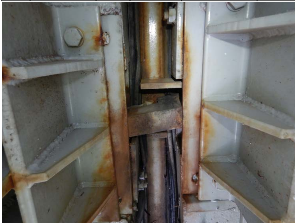
Photograph 32 - Looking south at the underside of the pier 6 modular joint at support box 3. Note: support bar has broken away from the transverse separation beam.
