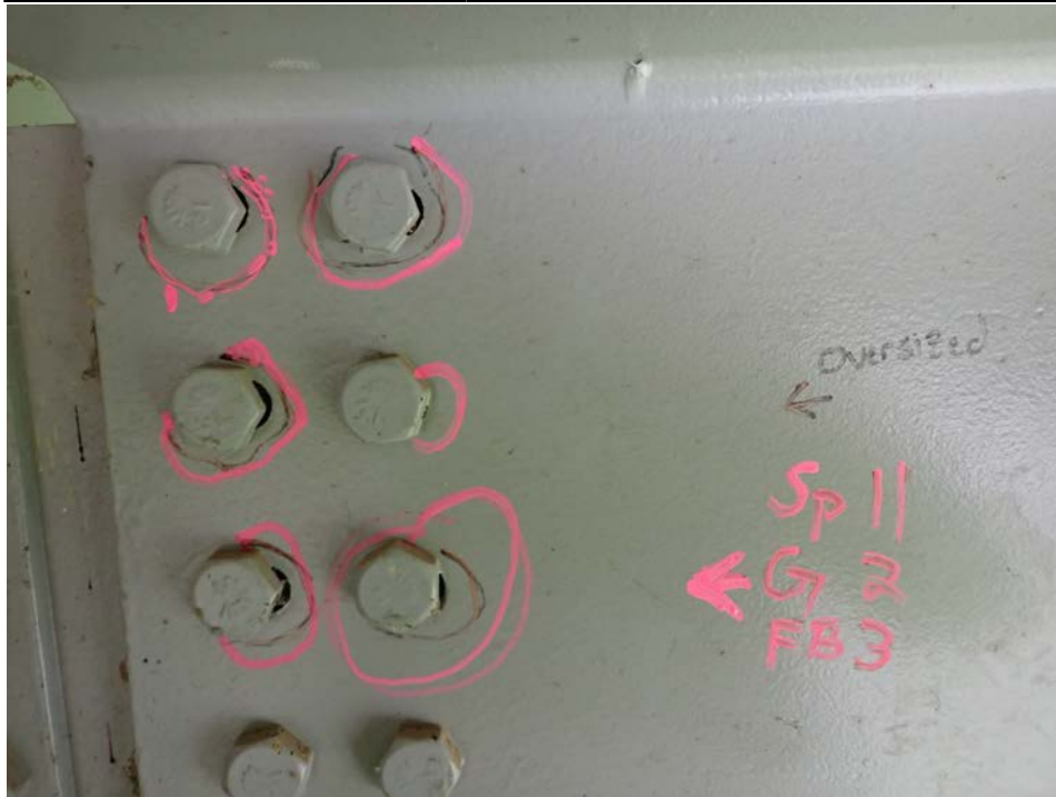
Photograph 71 - Looking east at floor beam 3, span 11 connection to girder 2. Note: top 6 bolt holes are oversized.
