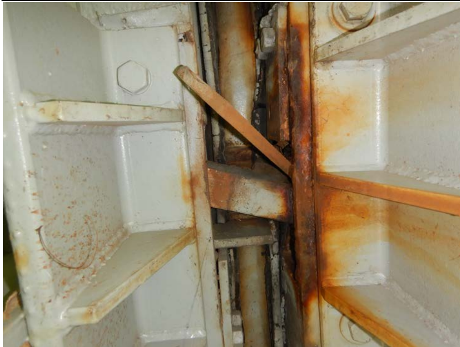
Photograph 35 - Looking up at the underside of the pier 10 modular joint at support box 4. Note: support beam is no longer attached to the transverse support beam and has slid east. South equidistant bar has broken and is wedged in place.
