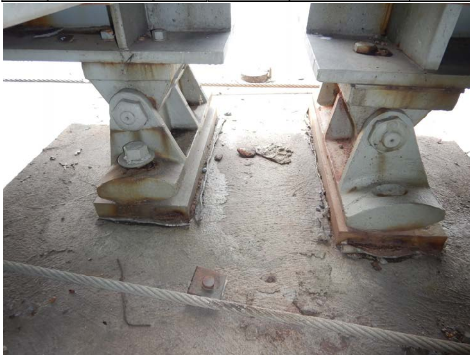
Photograph 94 - Looking south at the girder 1 expansion bearings at pier 6. Note: span 6 rocker rotated 14 degrees in expansion with anchor bolts missing. Span 7 rockers rotated 7 degrees in contraction at 85F. Brags are 8 inches tall to center of pin.
