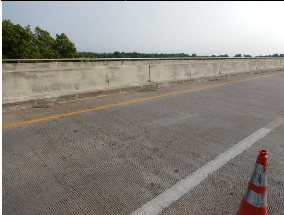
Photograph 5 - Looking northeast at the median bridge railing near mid span of span 1. Note: vertical cracks along the length of the bridge rail.
