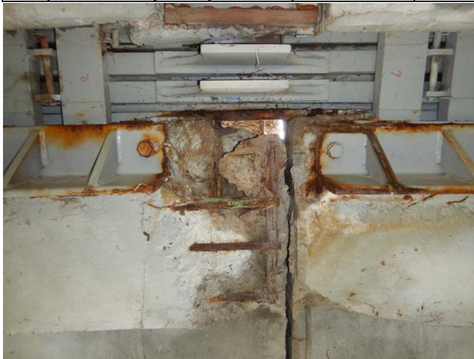
Photograph 16 - Looking east at the underside of the deck under the median at pier 3. Note: spalling with exposed reinforcing steel.
