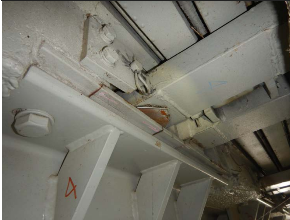
Photograph 21 - Looking southeast at the underside of the pier 3 modular joint at support box 4. Note: the bottom plate of support box has fractured and support bar 2 is unsupported.
