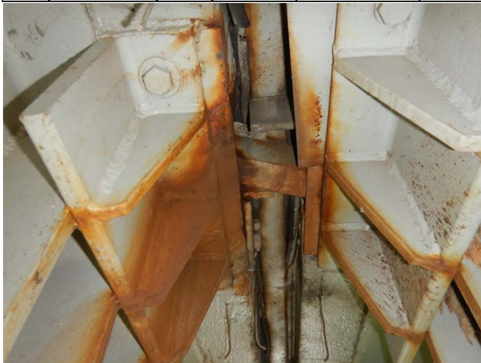
Photograph 34 - Looking south at the underside of the pier 10 modular joint at support box 3. Note: support beam is no longer attached to the transverse support beam and has slid east.
