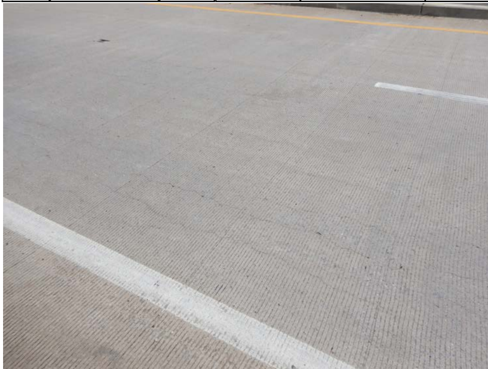
Photograph 12 - Looking southeast at the deck in the westbound lanes near mid span of span 1. Note: longitudinal cracks (typical in new section of approach beams).
