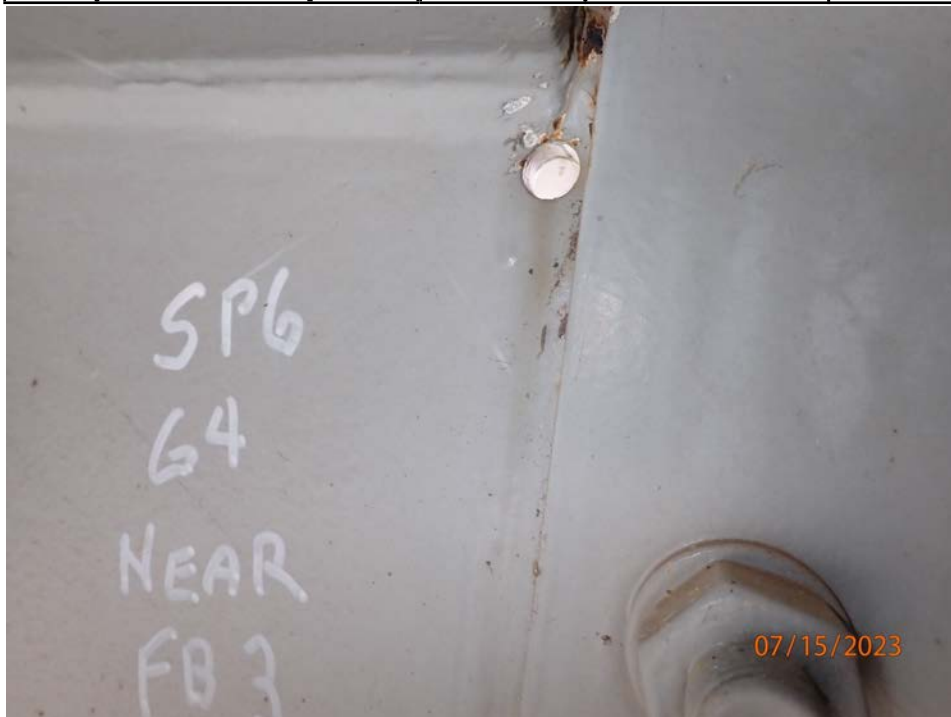
Photograph 52 - Looking north at the horizontal splice plate at girder 4 west of floor beam 3 at span 6. Note: lower web contains a 1 1/4-inch-long crack arrested with a drilled hole.
