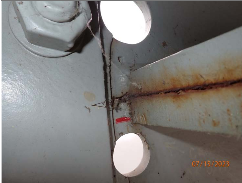
Photograph 43 - Looking north at the termination of the horizontal splice for girder 4, span 4 near floor beam 5. Note: 7/16-inch-long vertical crack in lower web between paint mark and drilled hole. Edge of fill plate for splice plate is cut by drilled holes.
