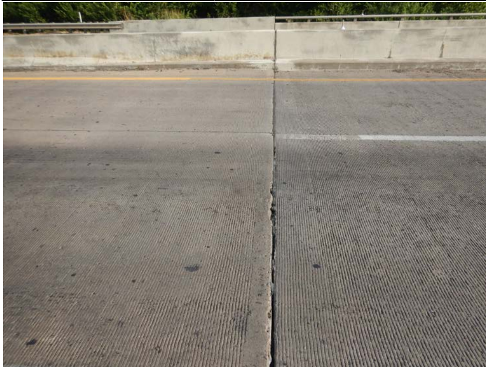
Photograph 38 - Looking north along the poured seal fixed joint at the west abutment. Note: seal is missing in south eastbound lane.
