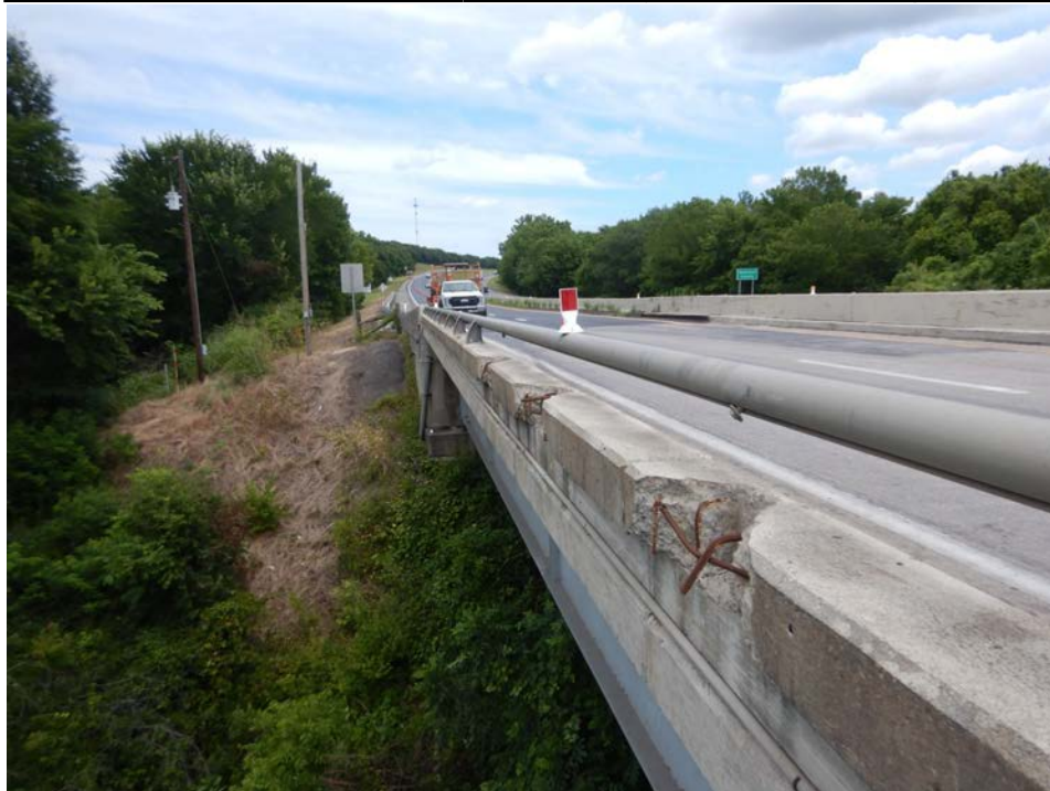
Photograph 4 - Looking southeast at the north bridge railing near mid span of span 13. Note: three spalls in the concrete railing where rail posts used to exist.
