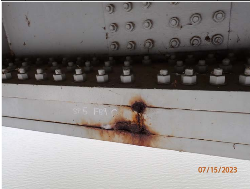
Photograph 55 - Looking northwest at the bottom flange bolted field splice for girder 4, span 5 at floor beam 9. Note: pack rust with minor section loss to the splice plates.
