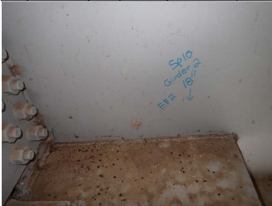
Photograph 73 - Looking north at girder 2, span 10 at floor beam 2. Note: 18-inch long crack in weld connecting gusset plate to the web.
