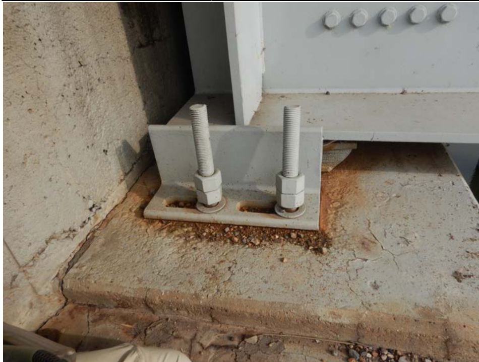
Photograph 89 - Looking north at the elastomeric expansion bearing for girder 1, span 4 at pier 3. Note: bearing assembly is near full expansion. Bearing assembly is in contact with the bearing seat with evidence of recent expansion observed.
