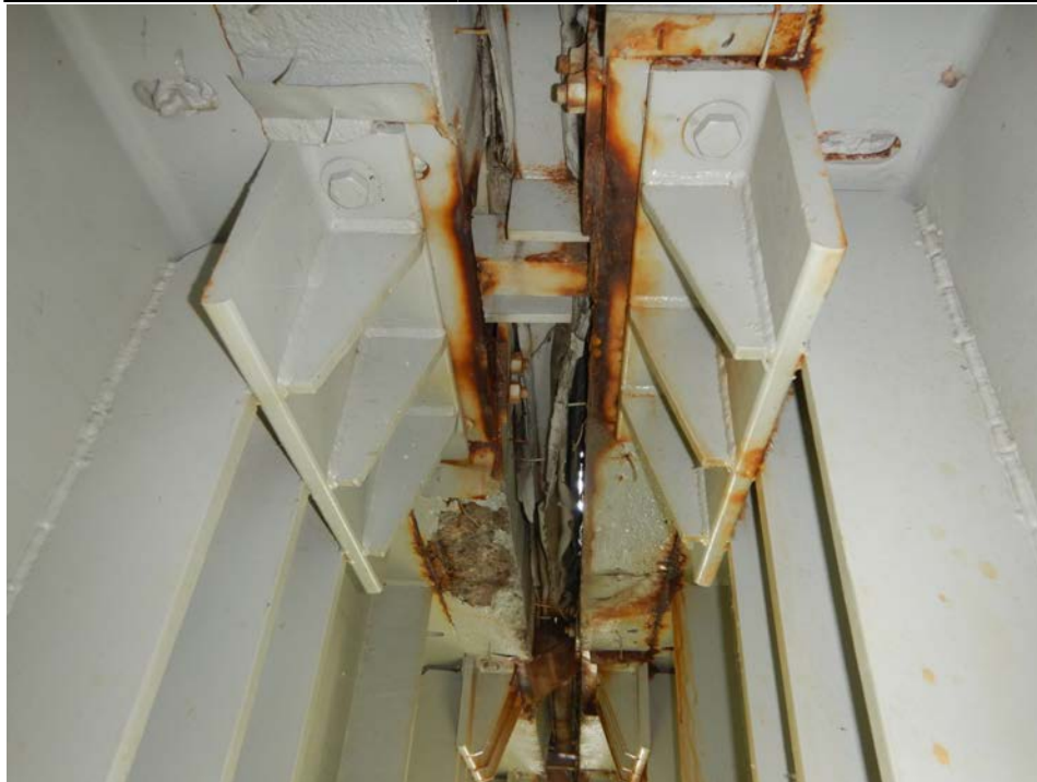
Photograph 37 - Looking north at the underside of the pier 6 modular joint between support boxes 9 and 10. Note: equidistant bar broken away at support box 10. Joint seal deteriorated and light visible through joint.
