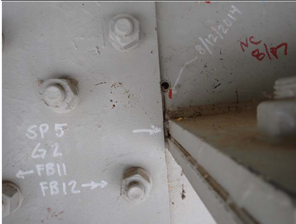
Photograph 45 - Looking north at the termination of the horizontal splice for girder 2, span 5 near floor beam 11. Note: 2-inch-long crack in upper web of girder at horizontal splice termination has been arrested by drilled hole.
