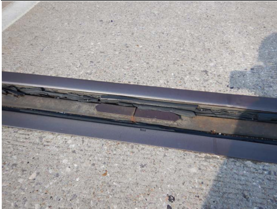
Photograph 30 - Looking west at the modular expansion joint in the south eastbound lane at pier 6. Note: repair of the transverse separation beam has failed and beam has dropped 1 inch.
