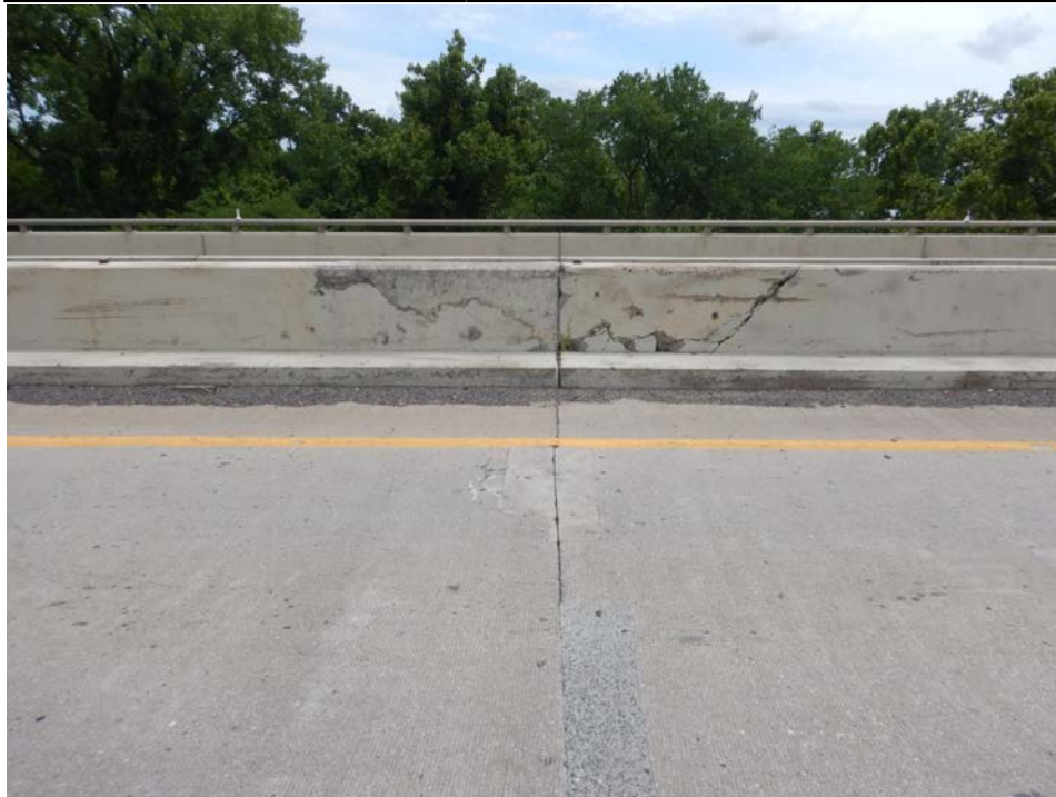
Photograph 6 - Looking south at the median railing near pier 12 . Note: spalling due to impact damage.
