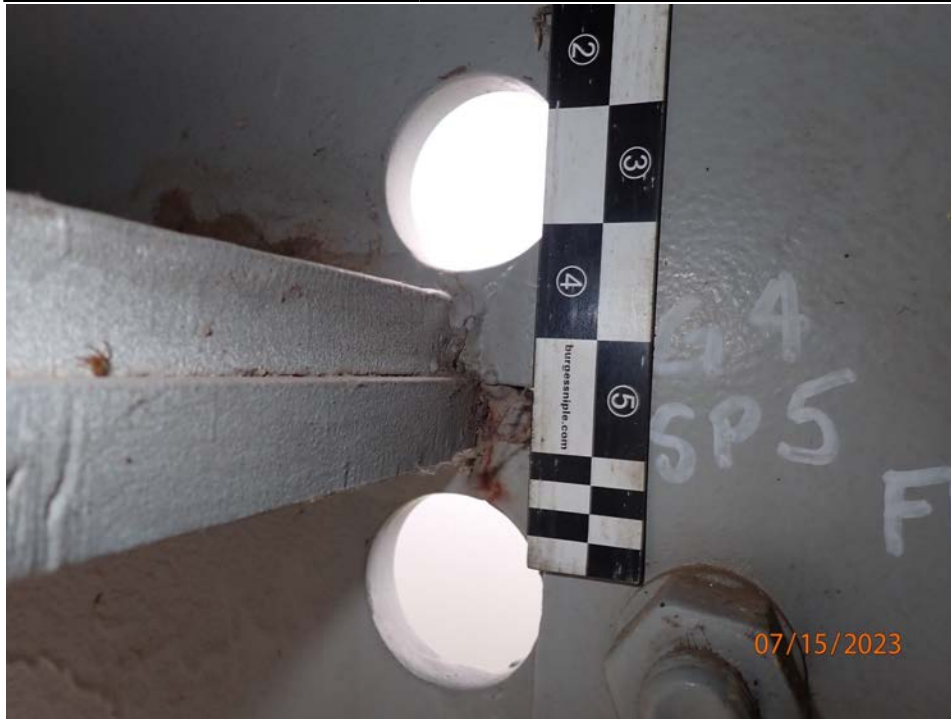
Photograph 47 - Looking north at the termination of the horizontal splice for girder 4, span 5 near floor beam 3. Note: 1 1/8-inch-long crack in upper web and 1-inch-long crack in lower web at horizontal splice termination has been arrested with drilled holes.
