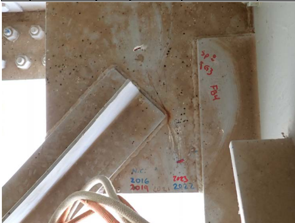
Photograph 72 - Looking southwest at the lateral bracing gusset plate connection to girder 3, span 8 at floor beam 4. Note: 8 1/2-inch-long crack running tangent to the corner of the bracing and one 3 1/2-inch-long crack along the floor beam bottom flange.
