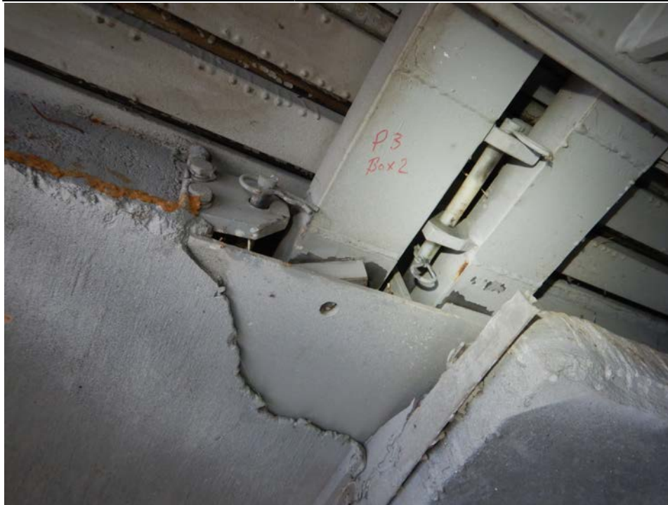
Photograph 19 - Looking northwest at the underside of the pier 3 modular joint at support box 2. Note: bottom plate of the support box is unsupported along the end of span 3. Equidistant spring between support bars is missing (typical).
