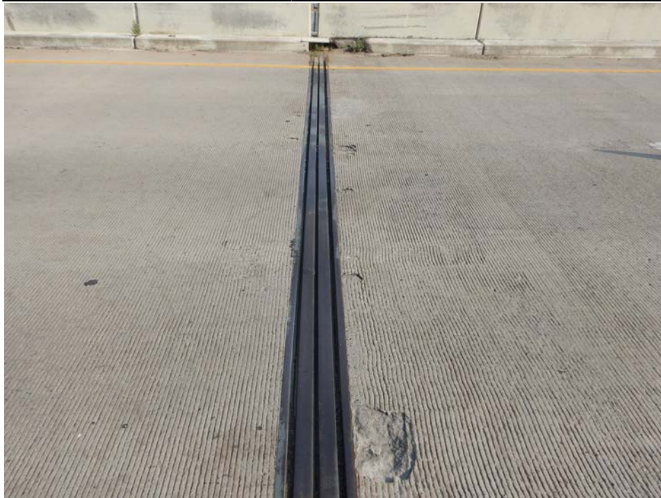
Photograph 40 - Looking north along the modular expansion joint in the eastbound lanes at pier 3. Note: spalls in the deck likely correspond with support boxes.
