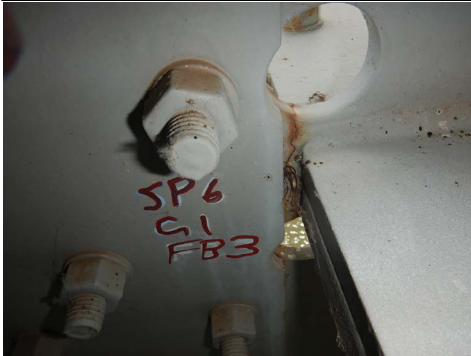
Photograph 49 - Looking south at the termination of the horizontal splice for girder 1, span 6 near floor beam 3. Note: cracks in upper and lower web at splice termination are arrested in drilled holes.
