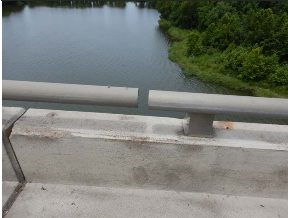
Photograph 7 - Looking north at the north bridge railing over floor beam 4, span 9. Note: splice for rail is missing.
