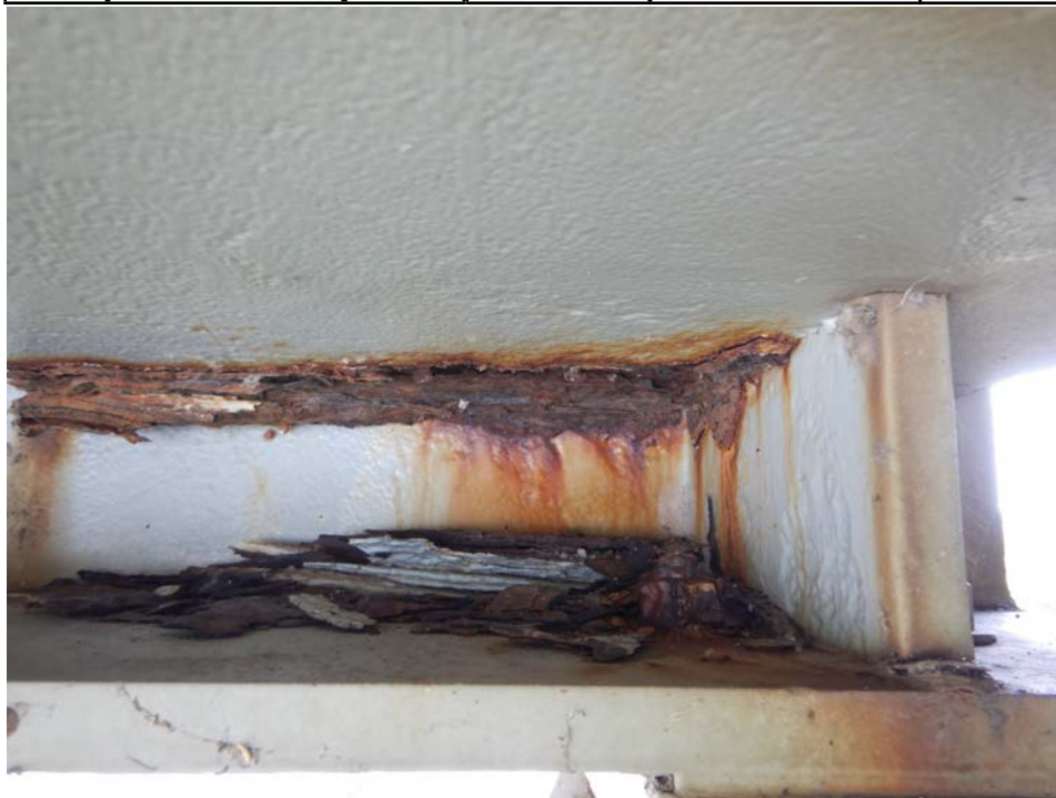
Photograph 56 - Looking north below the lateral bracing gusset plate connection to girder 4 at pier 6. Note: laminating corrosion and section loss exists in the girder web.
