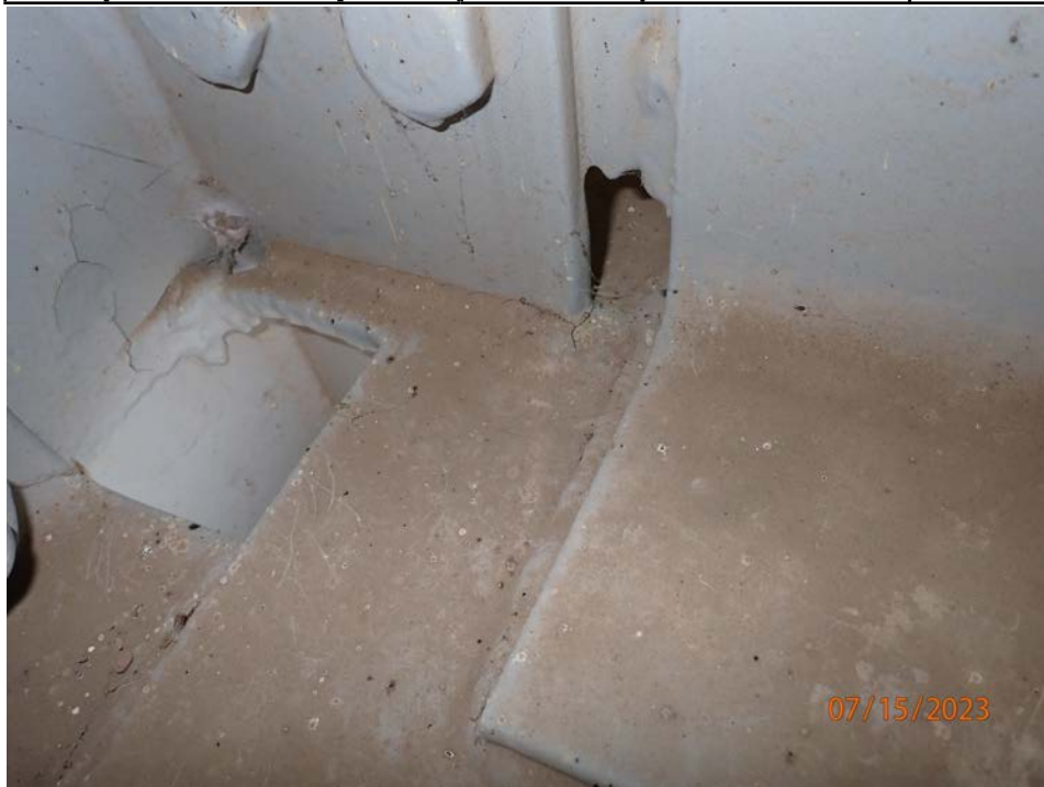
Photograph 60 - Looking east at the connection stiffener at girder 4, span 8 at floor beam 2. Note: 3 1/2-inch-long paint crack at the weld to the lateral bracing gusset plate.
