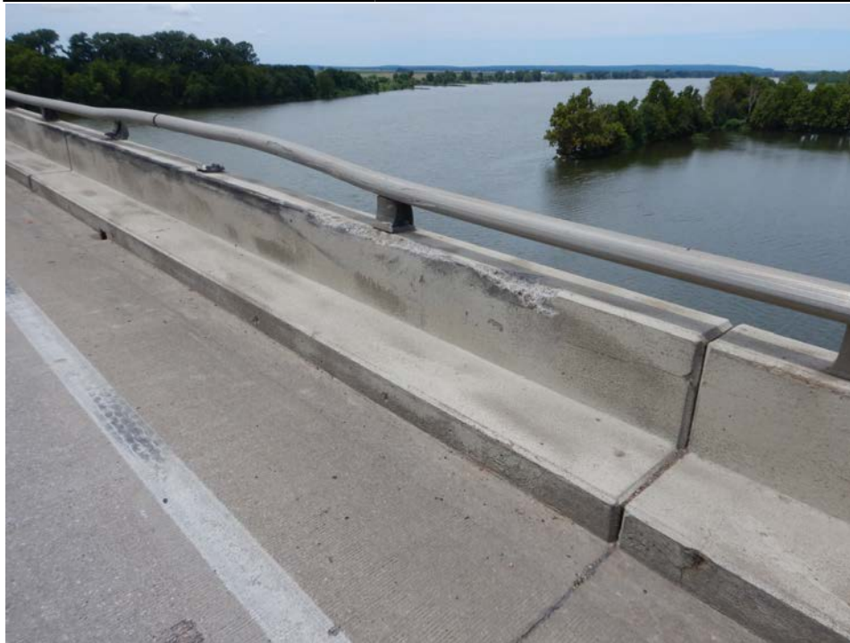
Photograph 3 - Looking northwest at the north bridge railing, span 8. Note: steel rail bent and two posts detached. Spalls in the concrete has not exposed reinforcing steel.
