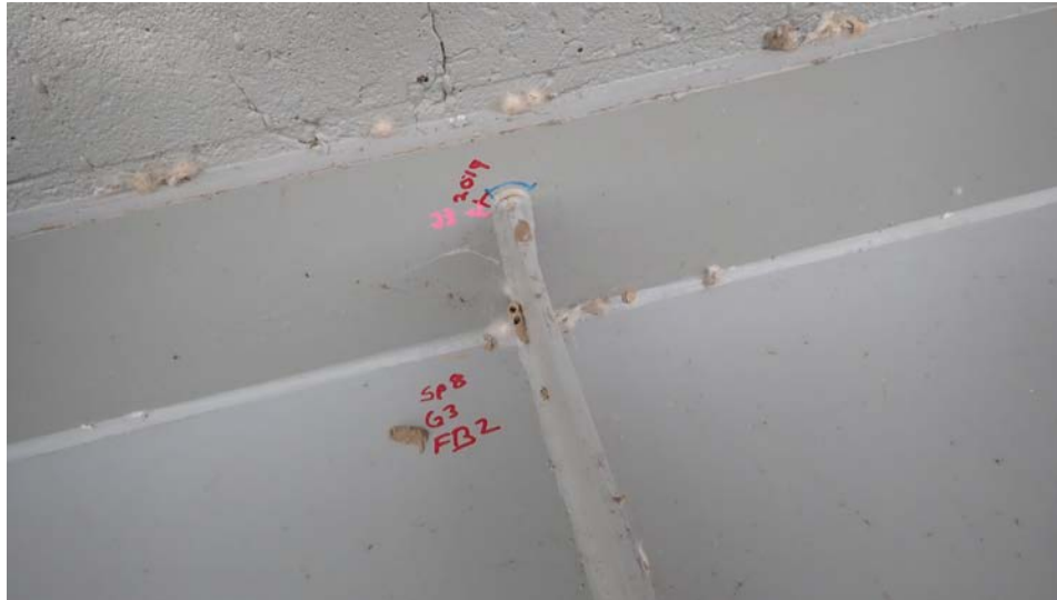
Photograph 59 - Looking south at the vertical stiffener for girder 3, span 8 at floor beam 2. Note: 1 3/4-inch-long paint crack in the weld to the top flange.
