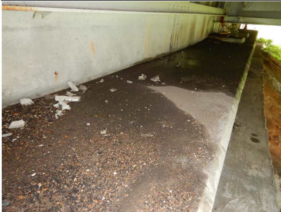
Photograph 81 - Looking south along the east abutment seat from girder 4. Note: ponding and debris exist on the bearing seat.
