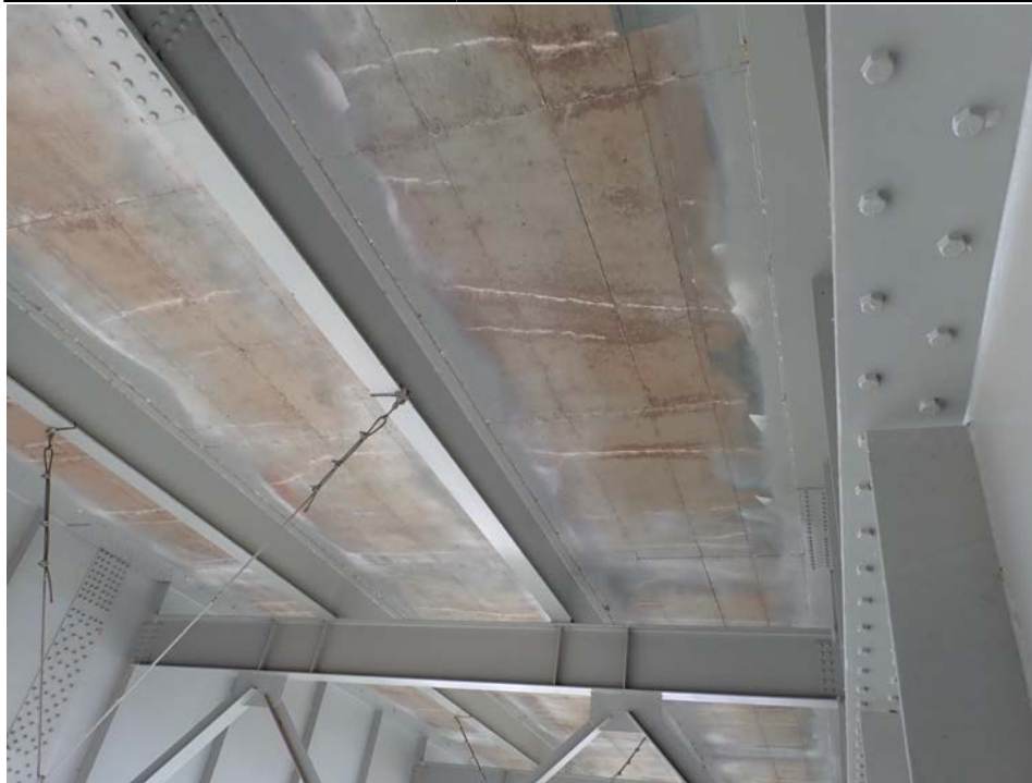
Photograph 15 - Looking northeast at the deck soffit between girders 3 and 4 near 1/3 span in span 6. Note: transverse cracking with efflorescence spaced at 3 to 6 feet.
