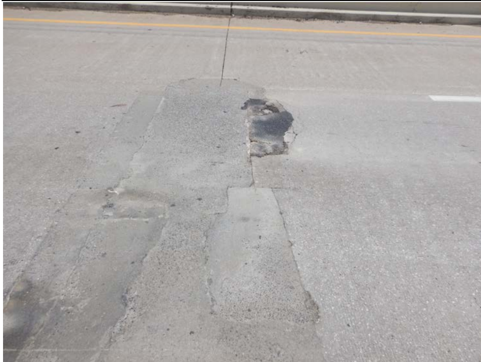
Photograph 10 - Looking south at the deck in the westbound lanes over floor beam 1, span 8. Note: patches with adjacent spalls forming along the deck control joint.
