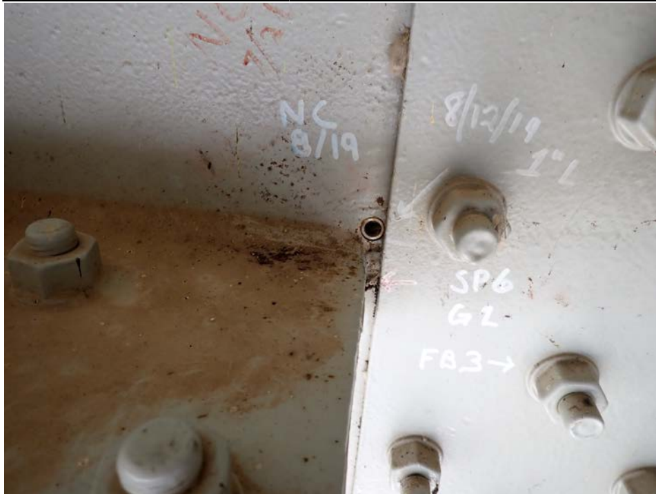
Photograph 50 - Looking north at the termination of the horizontal splice for girder 2, span 6 near floor beam 3. Note: 1-inch-long crack in upper web at horizontal splice termination has been arrested with drilled holes.
