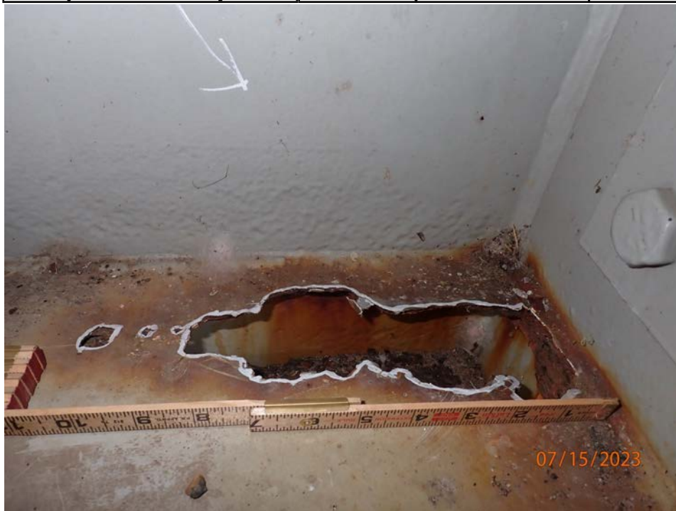
Photograph 78 - Looking north at lateral bracing gusset plate at girder 4, span 6 at pier 6. Note: 8 1/2-inch by 2 3/4-inch corrosion hole through the gusset plate.
