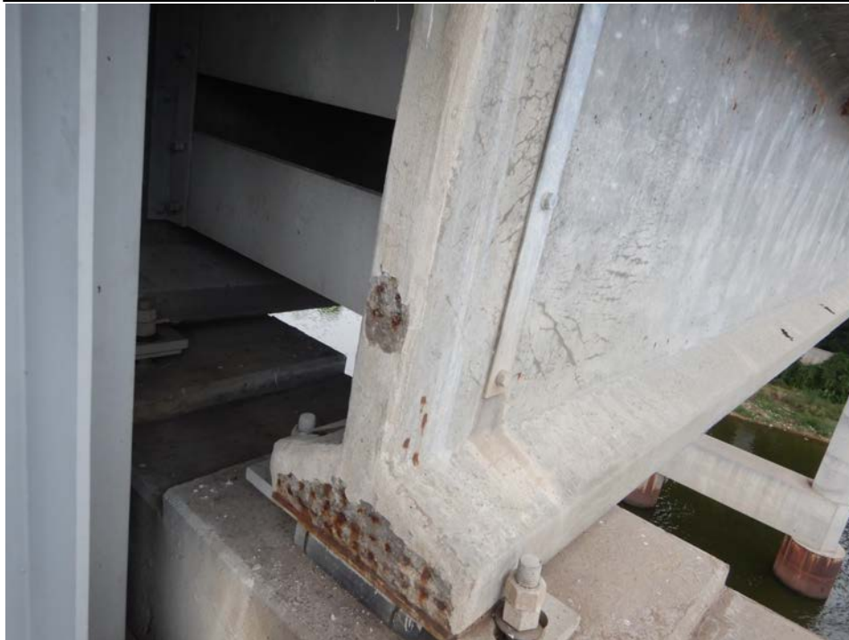
Photograph 62 - Looking southwest at prestressed beam 12, span 3 at pier 3. Note: strands exposed in the end of the beam (26 in bottom flange and 4 in web), corrosion stains and cracks with discolored concrete in web.
