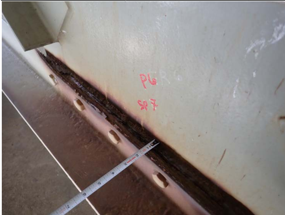
Photograph 70 - Looking northeast at floor beam 0, span 7 between girders 3 and 4. Note: 1-inch thick pack rust between lower strut and lower center gusset plate.
