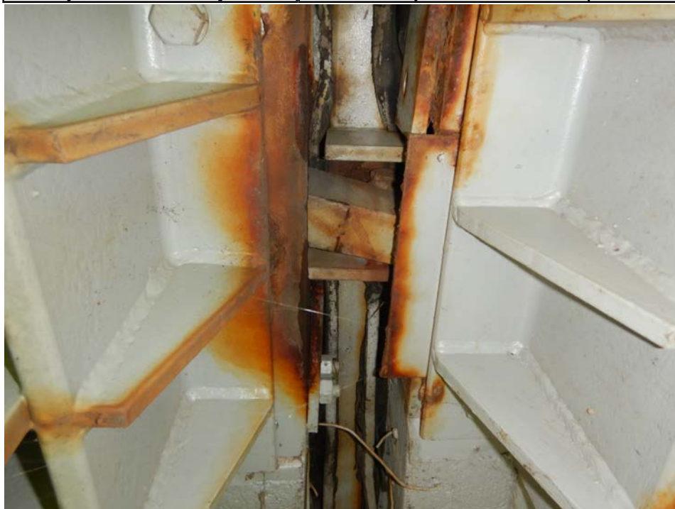
Photograph 36 - Looking north at the underside of the pier 10 modular joint at support box 5. Note: support beam is no longer attached to the transverse support beam and has slid east.
