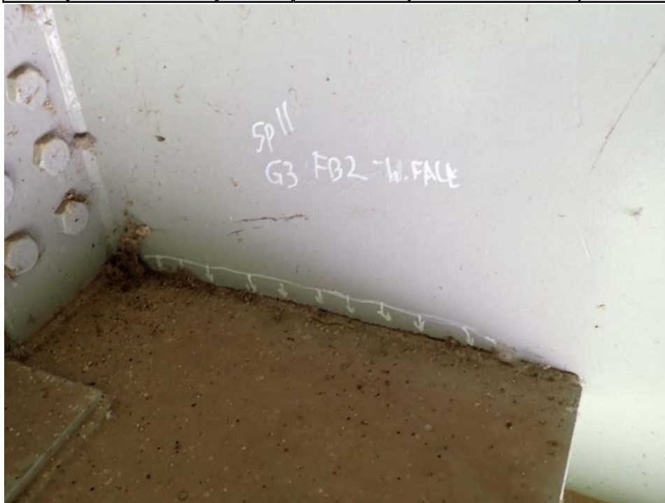
Photograph 76 - Looking south at lower lateral gusset plate weld at girder 3, span 11 at floor beam 2. Note: undercut weld.
