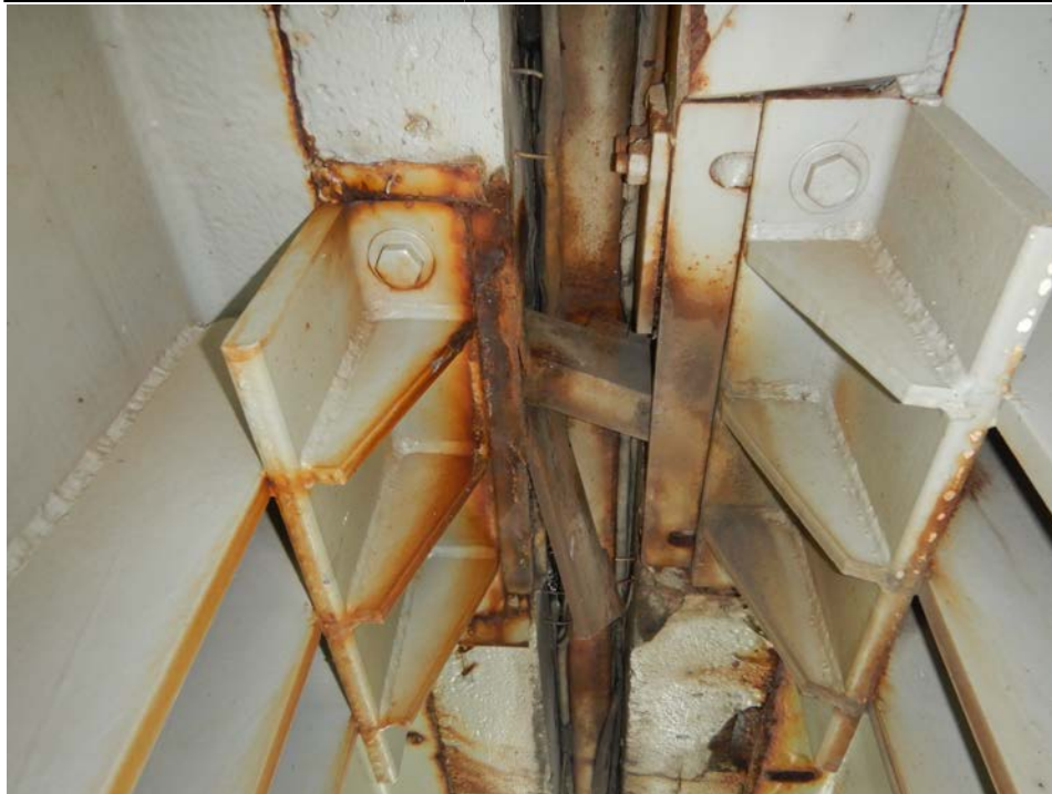
Photograph 33 - Looking north at the underside of the pier 6 modular joint at support box 13. Note: support bar has broken away from the transverse separation beam. One equidistant bar is missing and the other is loose.
