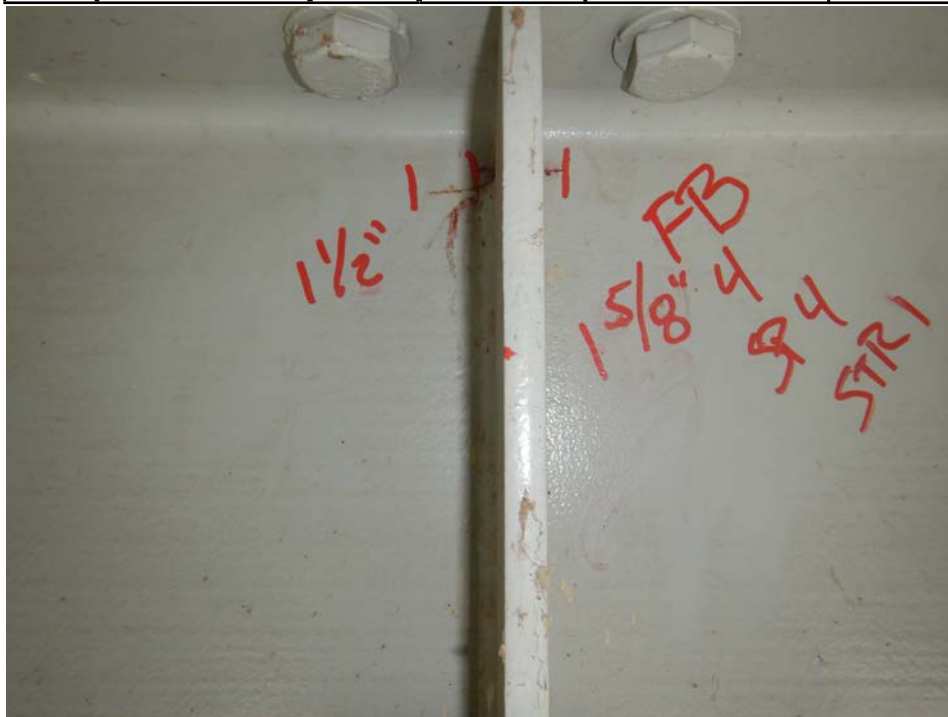
Photograph 66 - Looking west at floor beam 4 at stringer 1 in span 4. Note: 1 5/8-inch-long horizontal crack exists approximately 1/4 inch above the weld termination of the stiffener and extending north and south of the stiffener. 1 1/2-inch-long horizontal crack exists at the toe of the weld termination of the stiffener connection south.
