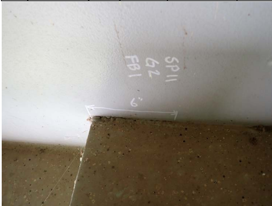
Photograph 74 - Looking north at girder 2, span 11 at floor beam 1. Note: 6-inch-long cracked weld in gusset plate weld.
