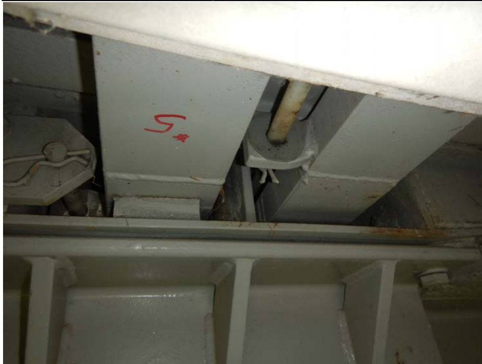
Photograph 22 - Looking east at the underside of the pier 3 modular joint at support box 5. Note: bearing block for support bar 1 is missing at the east support box. Stainless steel sliding surface is painted (typ.).
