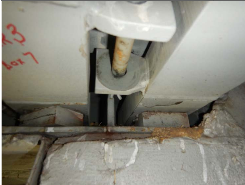
Photograph 24 - Looking west at the underside of the pier 3 modular joint at support box 7. Note: bottom plate of bearing support box is fractured adjacent to vertical plate.
