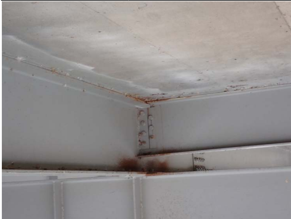
Photograph 18 - Looking northeast at stringer 4 over floor beam 4, span 7. Note: evidence of deck pumping.
