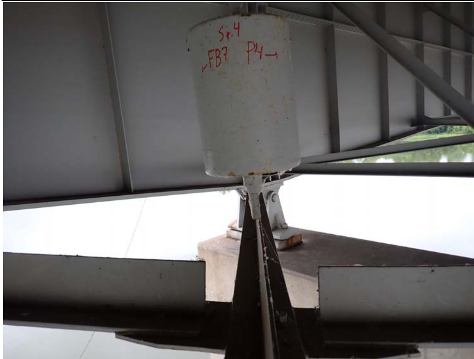
Photograph 77 - Looking northeast at the dampening canister between floor beam 7 and pier in span 4, 4. Note: canister lower anchor has broken and is no longer effective.
