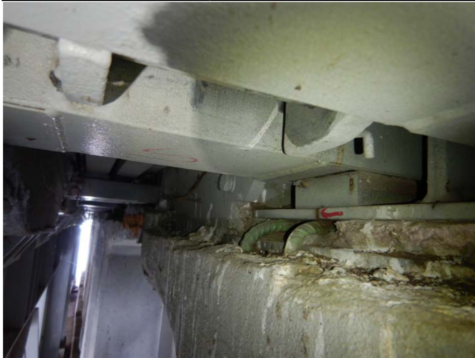
Photograph 26 - Looking southwest at the underside of the pier 3 modular joint at support box 15. Note: bottom plate of the west support box is fractured beneath the bearing block for support bar 1. Composite reinforcing extending up from beam 10 is exposed with no concrete under support box.
