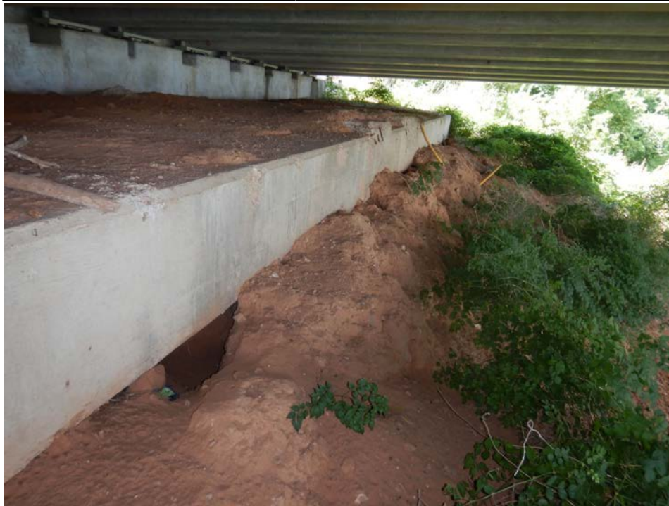
Photograph 83 - Looking north along the remnants of the original west abutment. Note: erosion exposing the underside of the breastwall.
