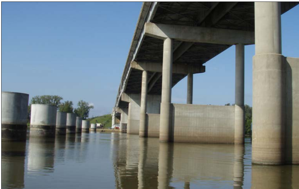
Figure 2.4-2: View of the 12-Foot Drilled Shaft Protection on the Downstream Side of the Bridge
