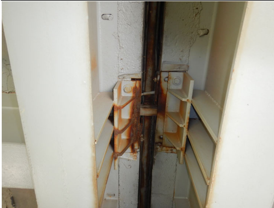
Photograph 19 - Looking north at support assembly 12 at the pier 6 modular joint. Note: no change to the missing control bars.
