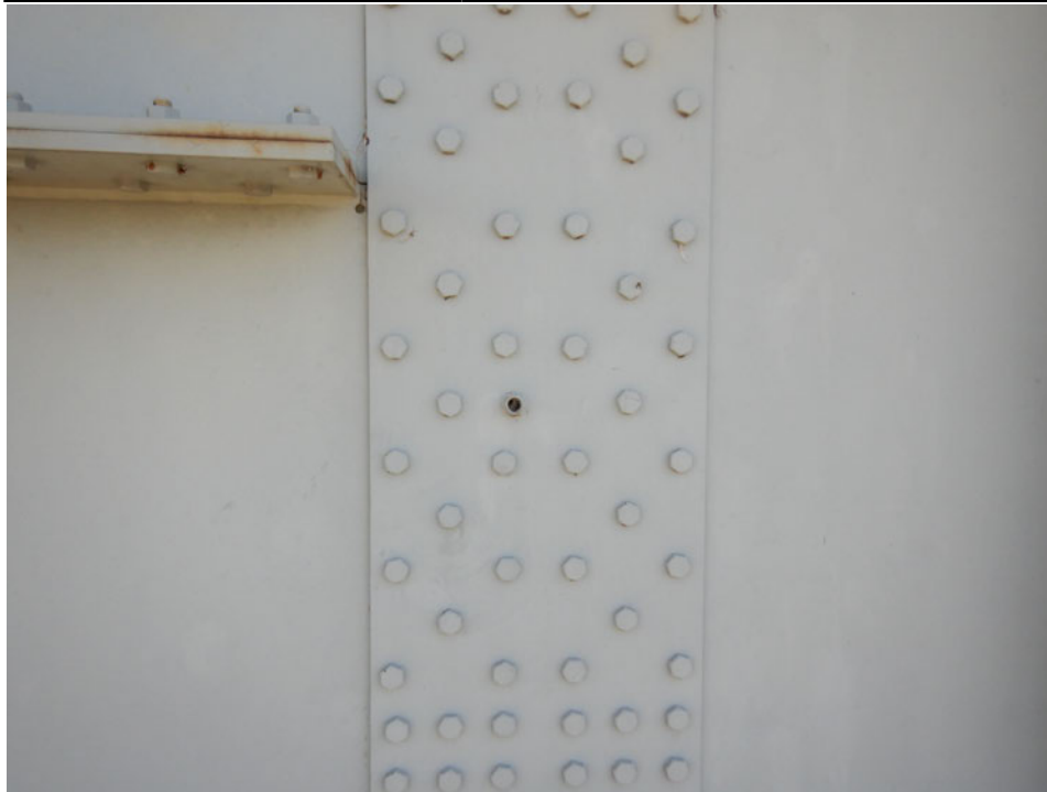
Photograph 35 - Looking south at the exterior face of the field splice for girder 4, span 5 near floor beam 11. Note: missing bolt in web splice.
