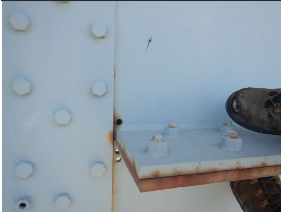
Photograph 27 - Looking north at the exterior face of girder 1, span 5 at floor beam 11. Note: upper web contains a 3/4-inch-long crack stopping short of the arrestor hole. Crack in bottom web is 1 1/4-inches-long and is arrested by two 1/2-inch-diameter drilled holes.
