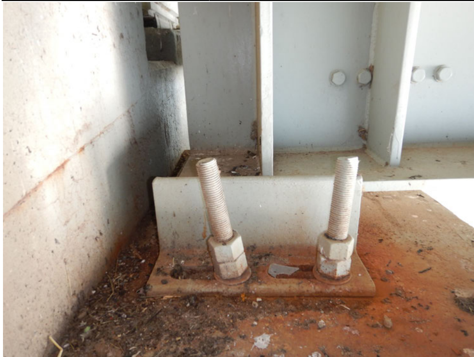
Photograph 47 - Looking north at girder 3 bearing for span 4 at pier 3. Note: elastomeric bearing pad exhibits no overhang. Anchor bolts are bent and in the fully extended position.
