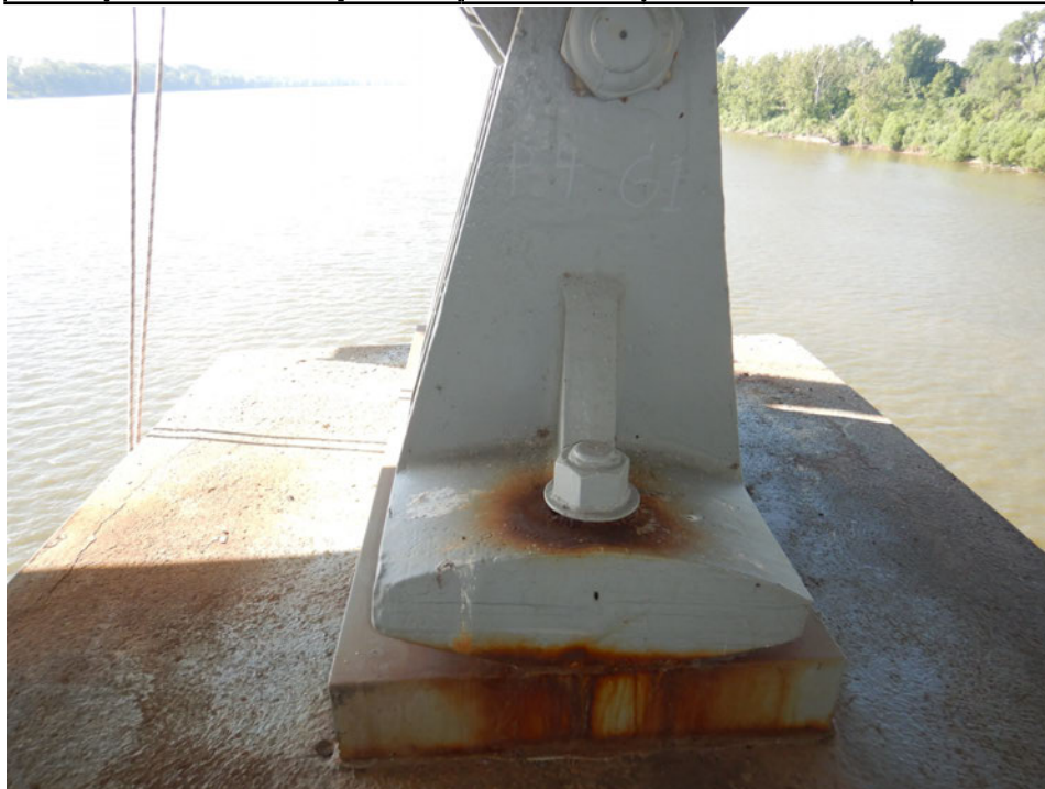
Photograph 48 - Looking south at the girder 1 bearing at pier 4. Note: all bearings at pier 4 are expanded up to 4 degrees at 90F.
