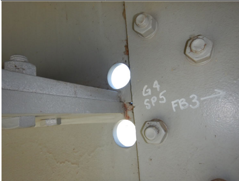
Photograph 32 - Looking north at girder 4, span 5 horizontal splice near floor beam 3. Note: crack present with arresting holes in pace. Crack has not jumped the arresting holes.
