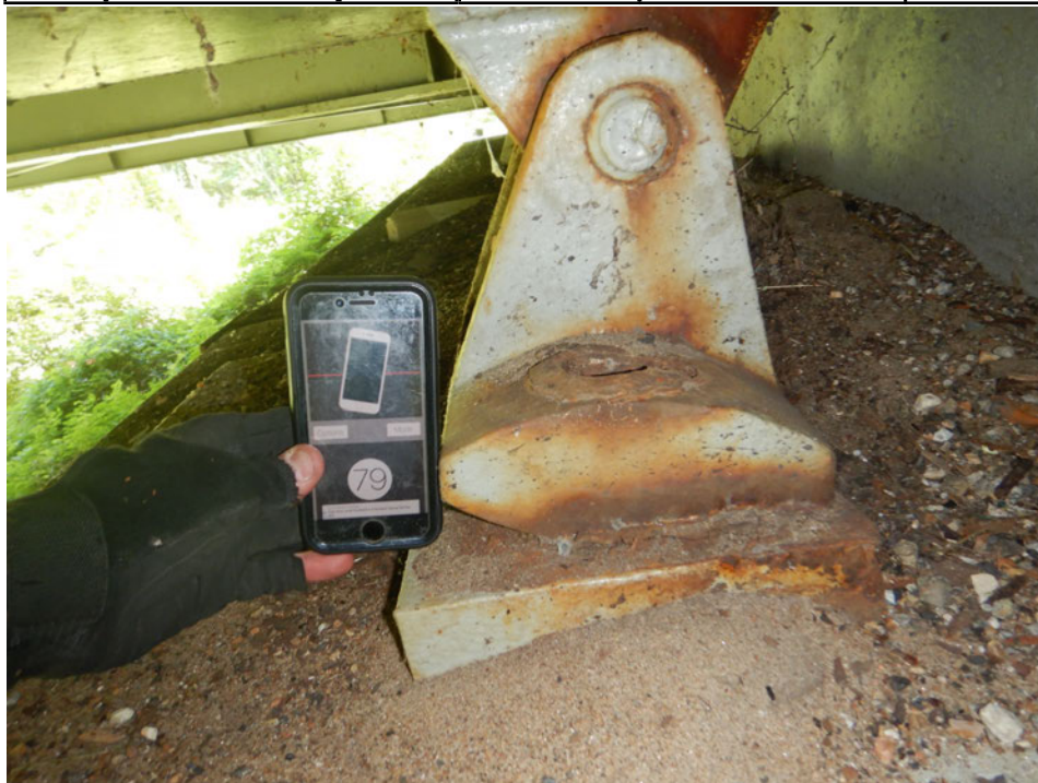
Photograph 50 - Looking north at the girder 2 rocker bearing at the east abutment. Note: bearings are 11 degrees in expansion at 90 degrees F.
