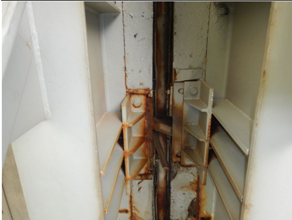
Photograph 20 - Looking north at support assembly 13 at the pier 6 modular joint. Note: one control bar is dislodged and one control bar is missing the transverse separation beam is bent and fractured.
