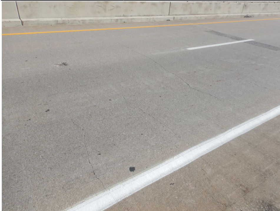
Photograph 8 - Looking northeast at the span 5 wearing surface. Note: transverse cracking spaced approximately 4 feet apart.
