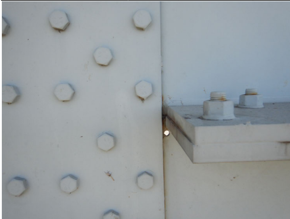
Photograph 42 - Looking south at the end of the longitudinal stiffener of girder 4, span 6 near floor beam 3. Note: 1 1/4-inch-long crack arrested in drilled holes.
