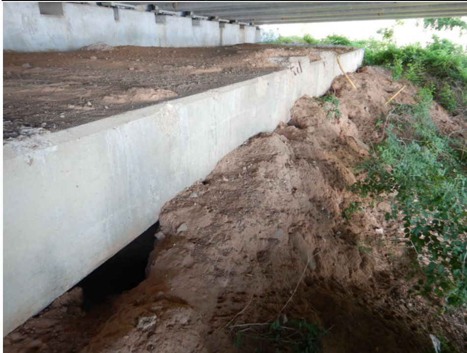
Photograph 53 - Looking north at the west abutment breastwall. Note: multiple erosion holes undermine the abutment up to 3 feet under beams 3, 5, and 7.
