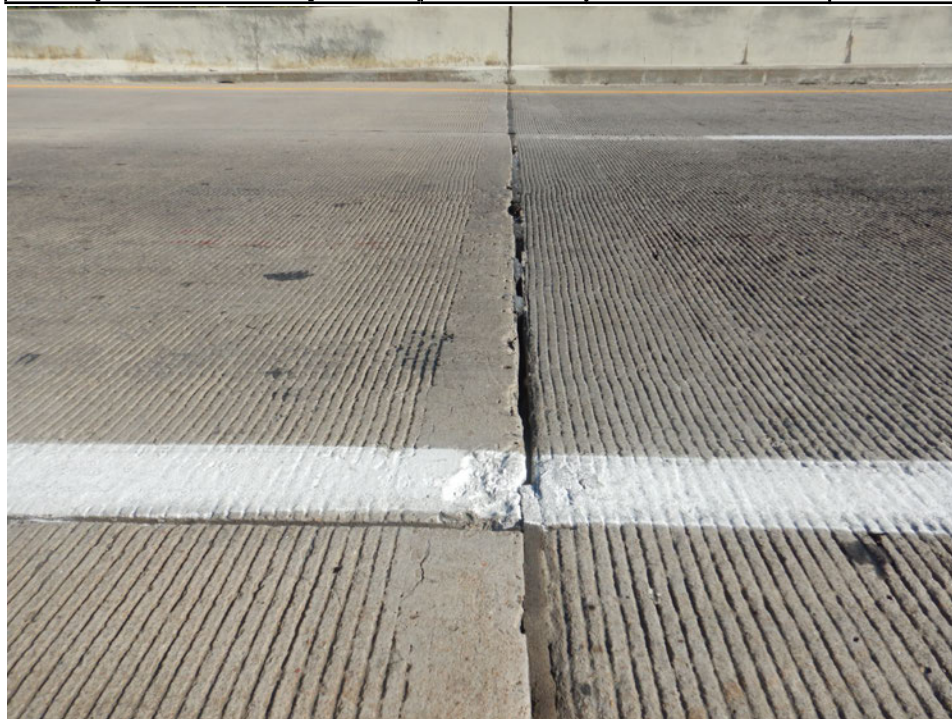
Photograph 4 - Looking north at the west abutment pourable joint. Note: 10 feet of joint seal is missing.
