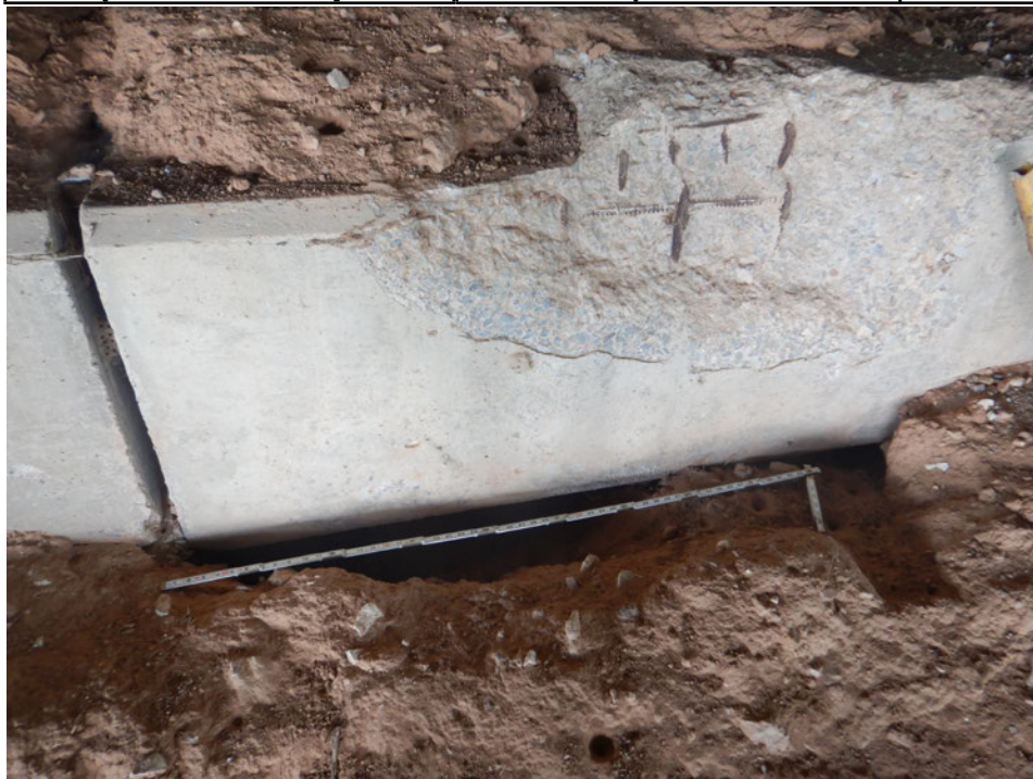
Photograph 56 - Looking west at the west abutment under beam 7. Note: 2-foot-deep erosion hole with 18 inches of penetration, and a 3-foot-wide x 2 1/2-foot-tall x 3/4-inch-deep spall with exposed reinforcement at the top corner of the breastwall.
