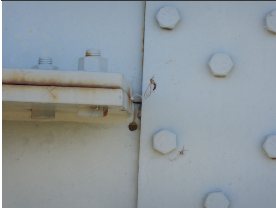
Photograph 34 - Looking south at end of the longitudinal stiffener for girder 4, span 5 near floor beam 11. Note: no change to crack in lower web arrested with a drilled hole.
