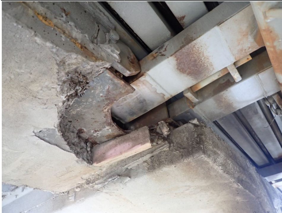
Photograph 17 - Looking northwest at support joint assembly 16 at the pier 3 modular joint. Note: west bottom plate of the support box and the 3-inch-thick unreinforced concrete pour below the support box have fractured and are no longer supporting the south support bar.
