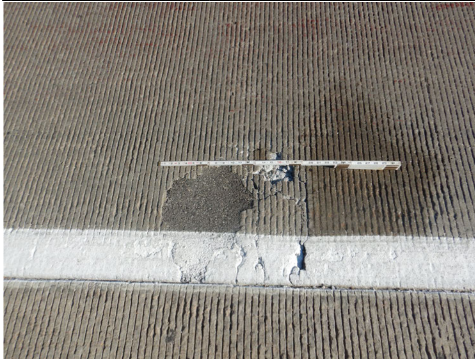
Photograph 3 - Looking north at the west approach slab. Note: 20-inch-diameter asphalt filled patch.
