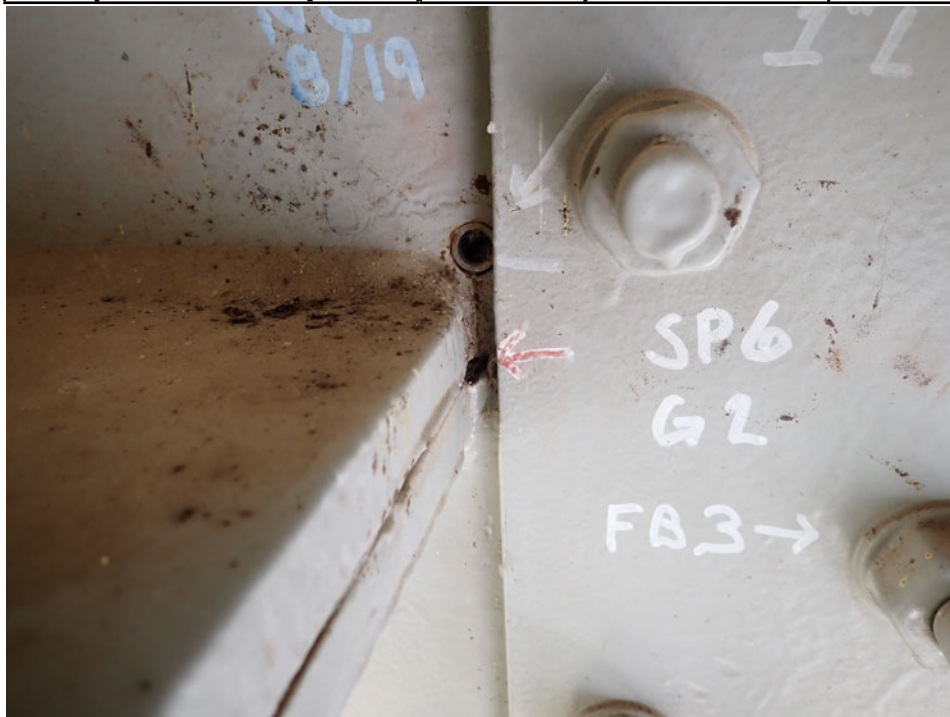
Photograph 38 - Looking north at end of the longitudinal stiffener of girder 2, span 6 near floor beam 3. Note: no change to crack in upper web retrofitted with a crack arrest bushing.
