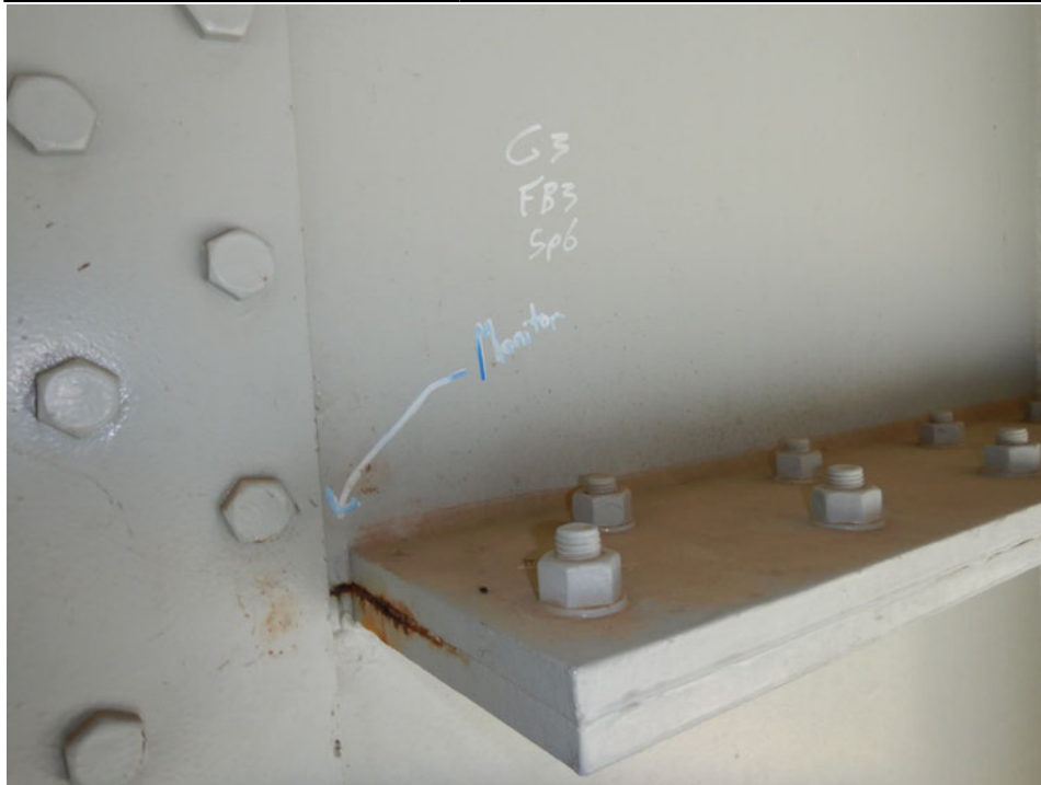
Photograph 39 - Looking south at the interior face of girder 3, span 6 near floor beam 3. Note: no change to paint crack at end of horizontal web splice.
