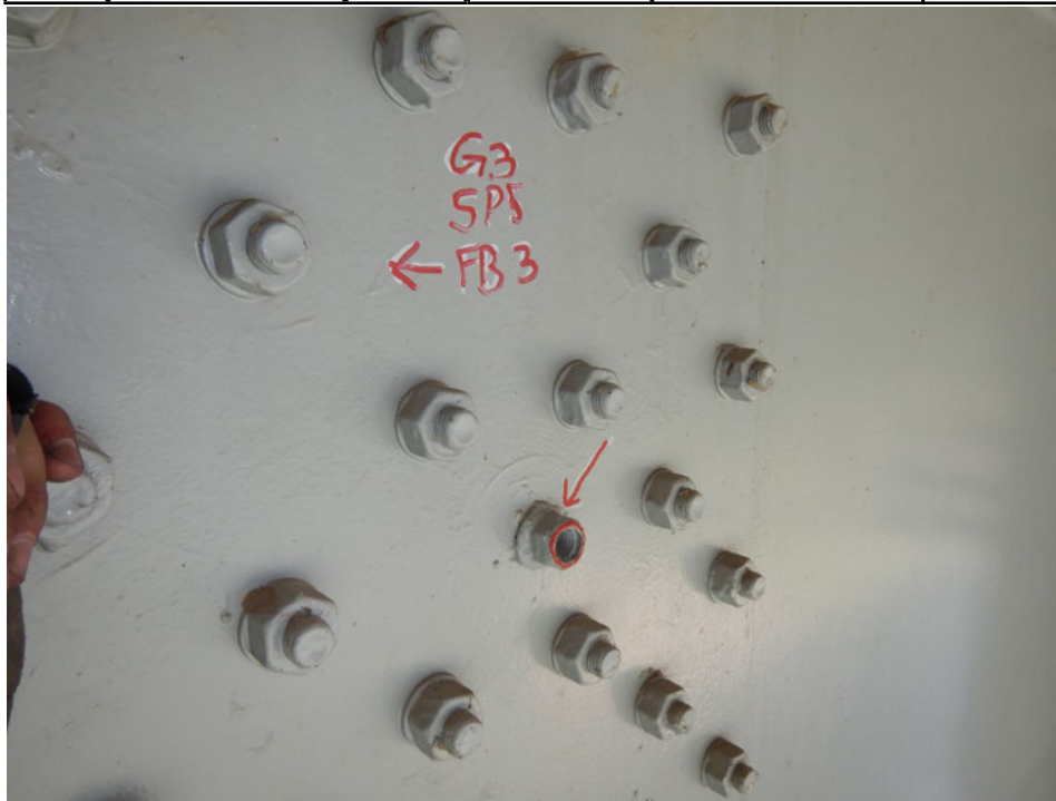
Photograph 30 - Looking south at girder 3, span 5 horizontal splice near floor beam 3. Note: missing bolt in the web of the girder.
