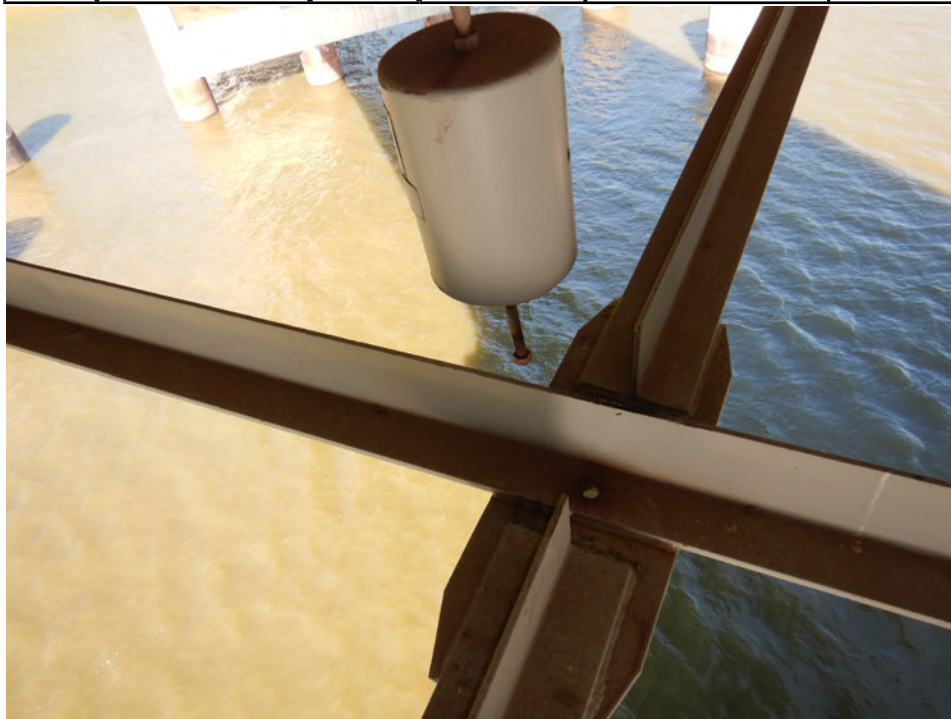
Photograph 24 - Looking northwest at lower lateral bracing dampener in span 4 between girders 1 and 2 and between floor beams 7 and 8. Note: dampener not connected to lower lateral bracing.
