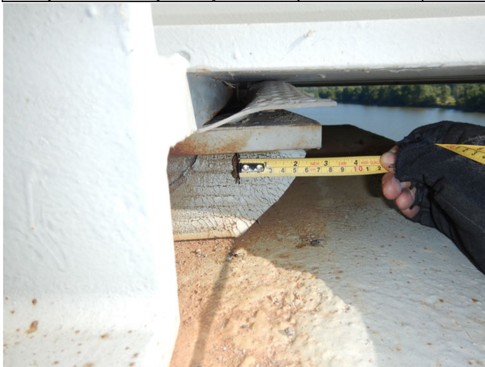
Photograph 46 - Looking north at girder 1 bearing for span 4 at pier 3. Note: elastomeric bearing pad exhibits an overhang to the east of up to 2 1/2 inches with the anchors bolts in the full extended position. Anchor bolts also exhibit some bending, may be due to the alignment of the bearing.
