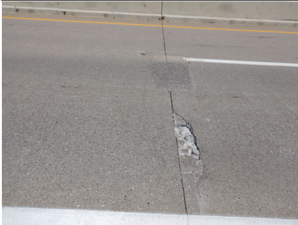
Photograph 11 - Looking north at the span 10 deck top at the deck control joint. Note: 1-foot-long x 2-foot-wide x 2 1/2-inch-deep spall in south wheel line of south eastbound lane.
