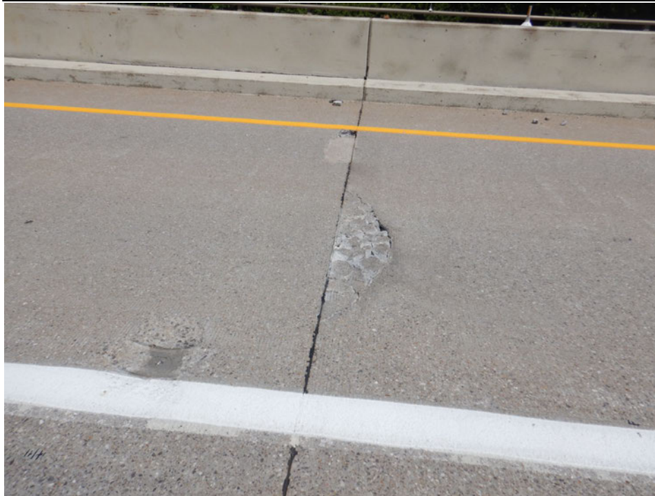
Photograph 13 - Looking north at the span 13 deck top at the deck control joint. Note: spall in the northern eastbound lane.
