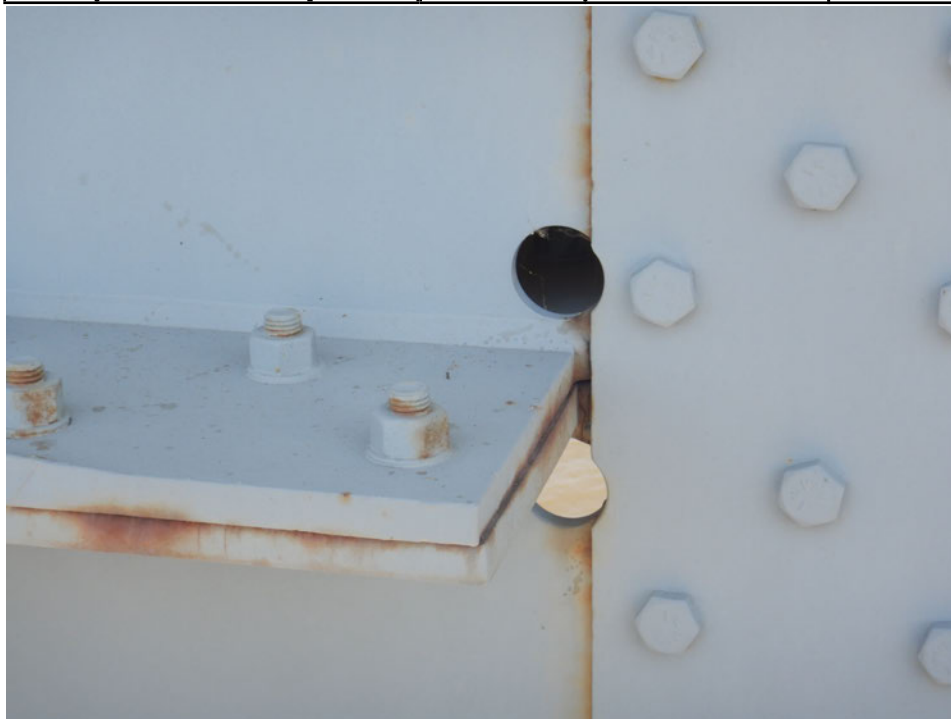
Photograph 36 - Looking north at the exterior face of girder 1, span 6 at floor beam 3. Note: two vertical cracks at the end of the longitudinal splice plates arrested in 2-inch-diameter holes.
