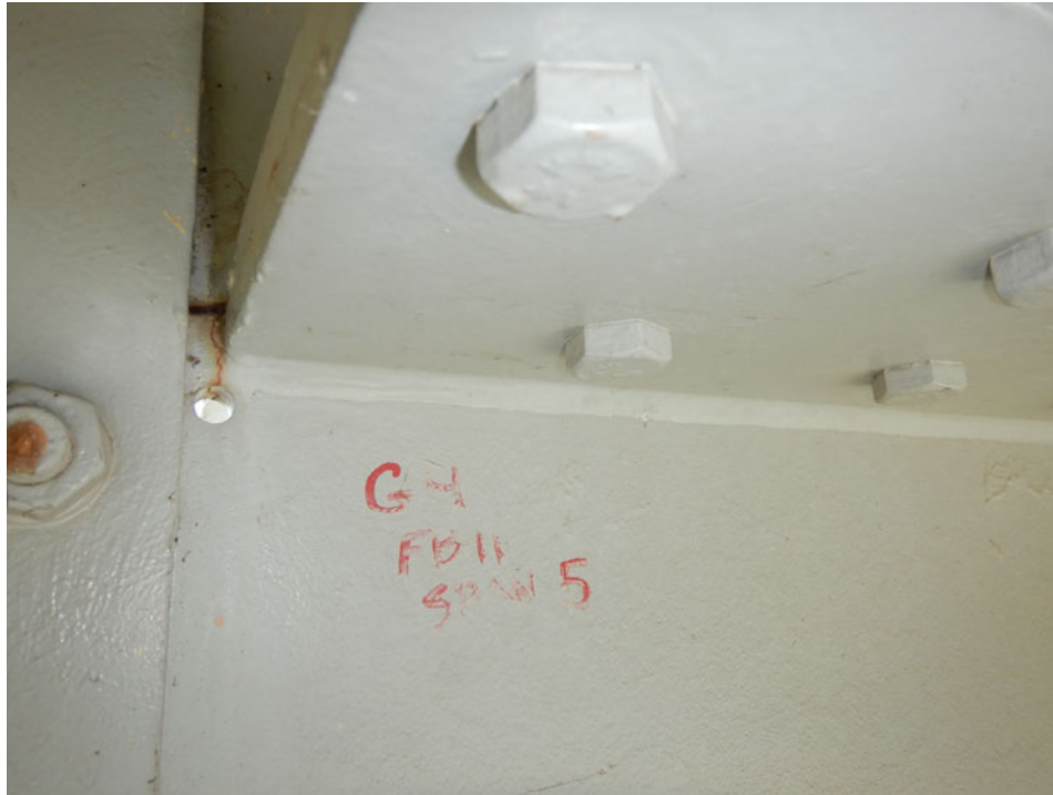
Photograph 33 - Looking north at the interior face of girder 4, span 5 near floor beam 11. Note: no change to crack with arrest hole at end of horizontal web splice.
