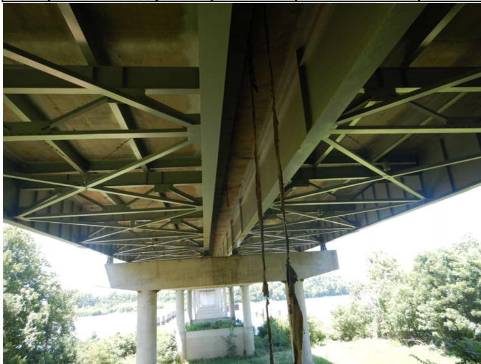
Photograph 44 - Looking west at the underside of framing in span 13. Note: no significant deficiencies.
