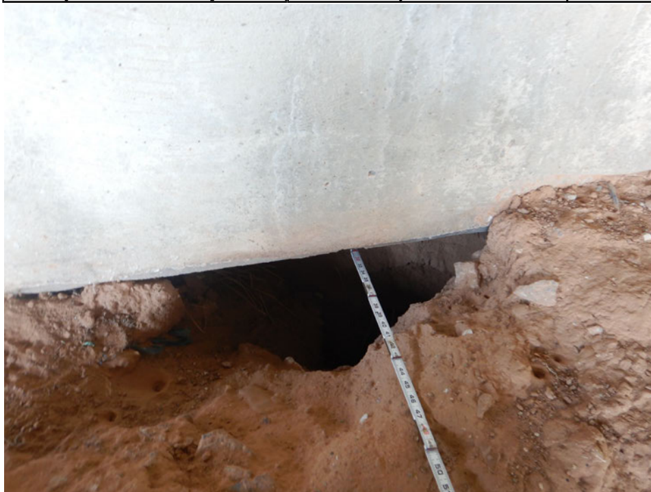
Photograph 54 - Looking west at the west abutment under beam 3. Note: 26-inch-deep erosion hole with 3 feet of penetration.
