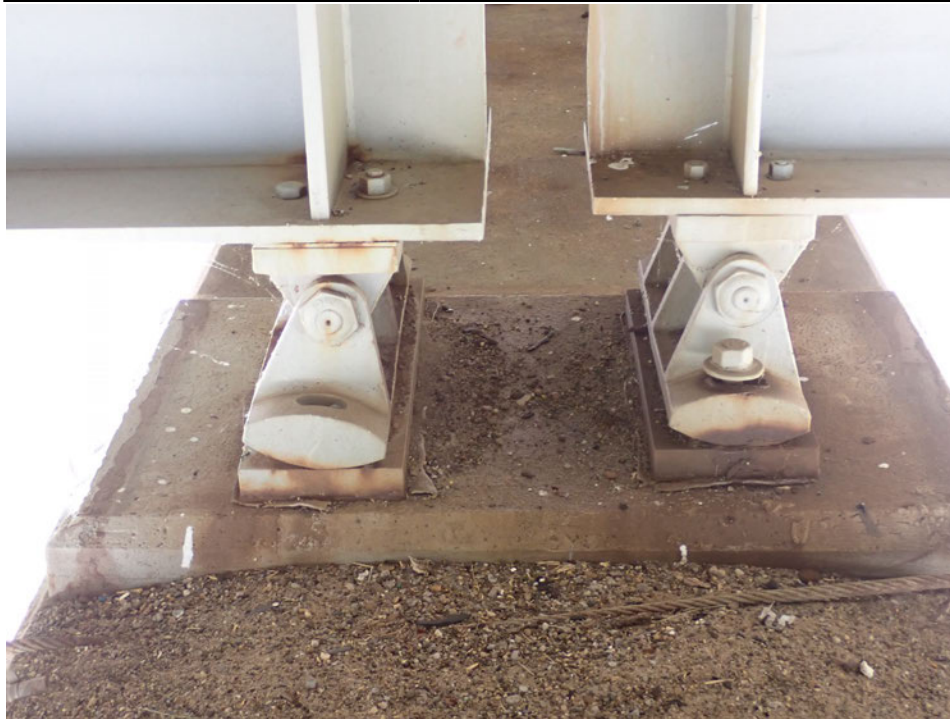
Photograph 49 - Looking north at the girder 3 bearing at pier 6. Note: span 6 bearing is rotated.
