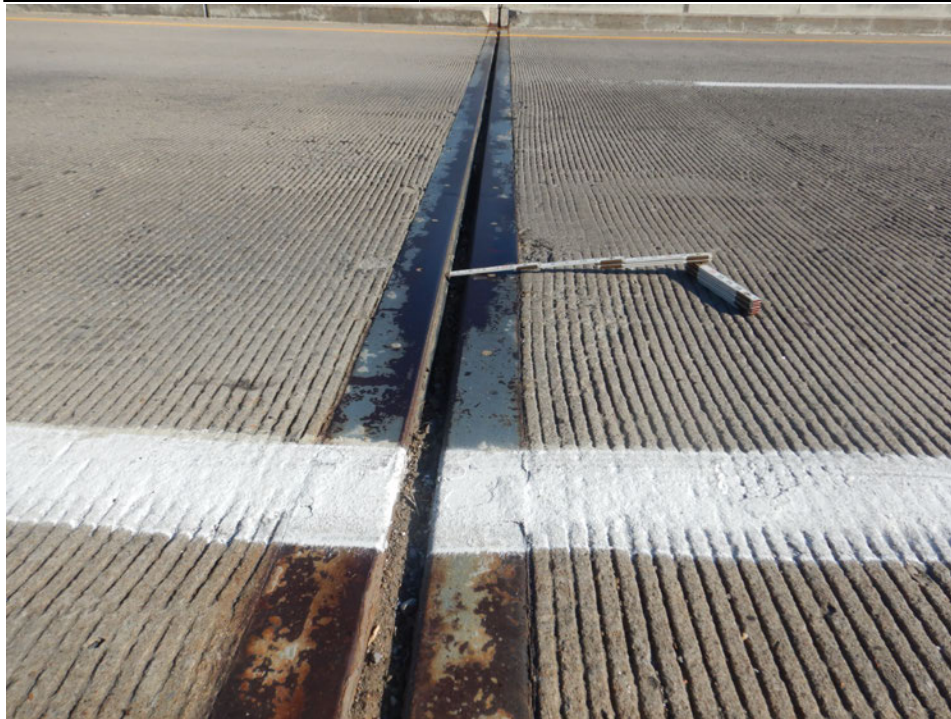
Photograph 5 - Looking north at the pier 1 expansion joint. Note: joint is filled with soil and open 1 1/2 inches.
