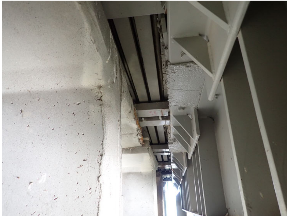
Photograph 15 - Looking north at the underside of the pier 3 joint. Note: typical condition of joint with no equidistant bars.
