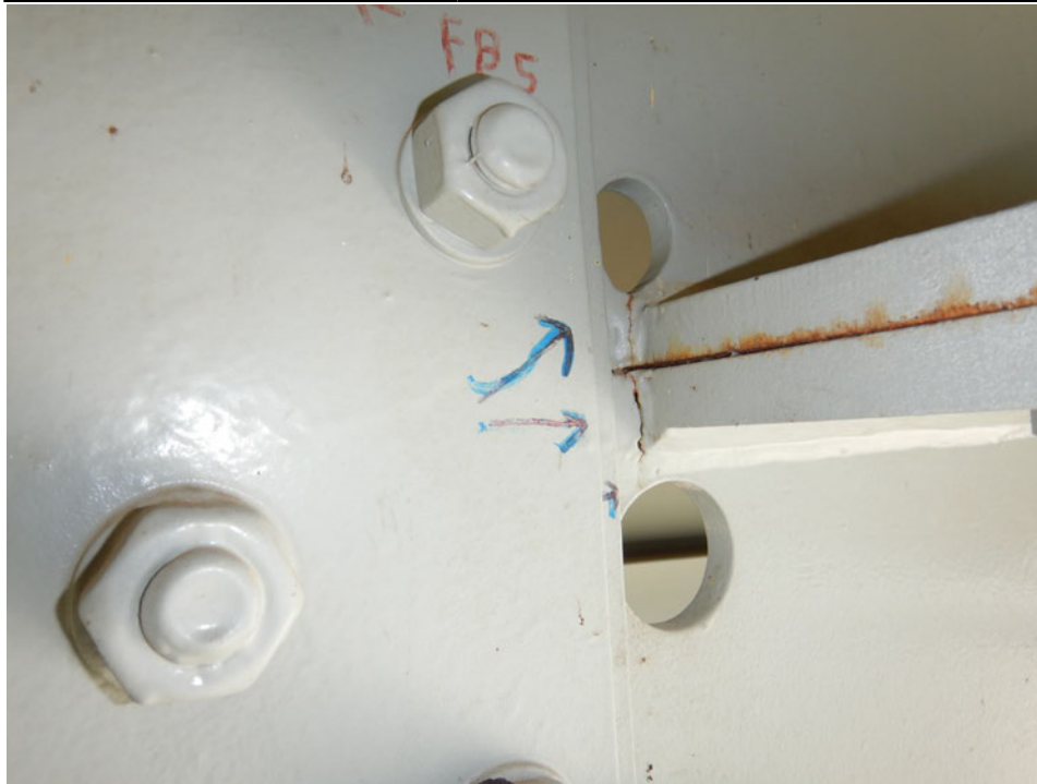
Photograph 23 - Looking northeast at girder 2, span 4 at end of horizontal splice near floor beam 5. Note: no change to crack at end of horizontal splice.
