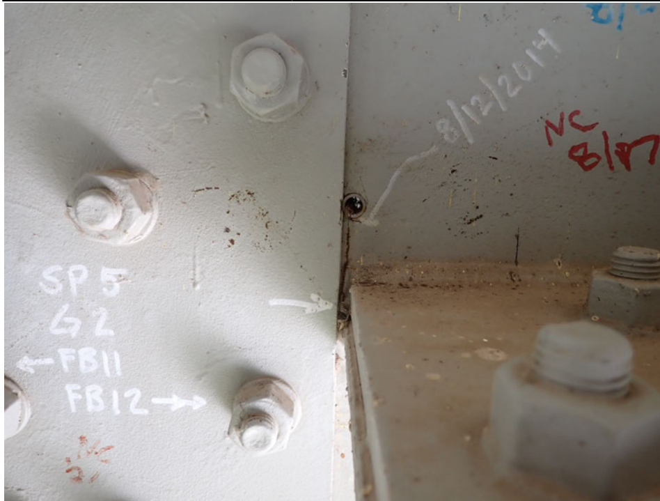
Photograph 29 - Looking north at girder 2, span 5 near floor beam 11. Note: no change to 2-inch-long crack retrofitted with crack arrested bushing in the upper web.
