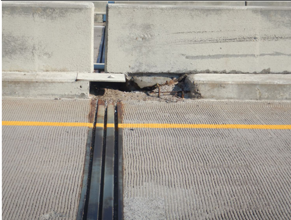
Photograph 6 - Looking north at the median curb at pier 3. Note: end 2 feet of curb is spalled with exposed reinforcement.
