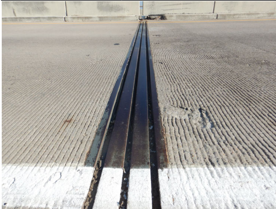
Photograph 7 - Looking north at the pier 3 modular joint. Note: west transverse bar is lifted 1/4-inch.
