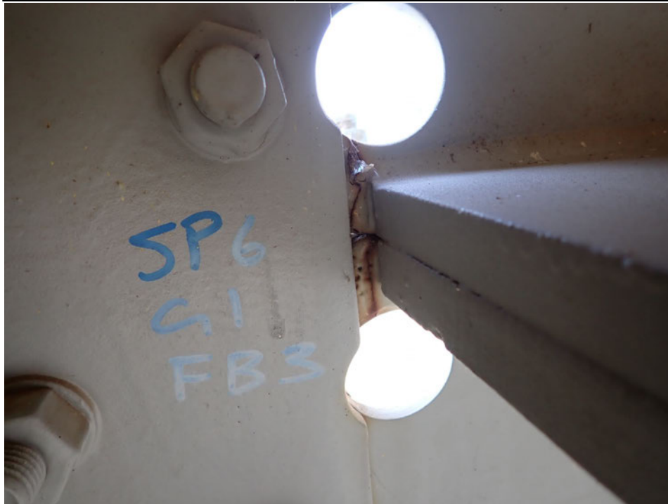
Photograph 37 - Looking south at the end of the longitudinal stiffener for girder 1, span 6 near floor beam 3. Note: no change to two cracks arrested by 2-inch-diameter arrestor holes.
