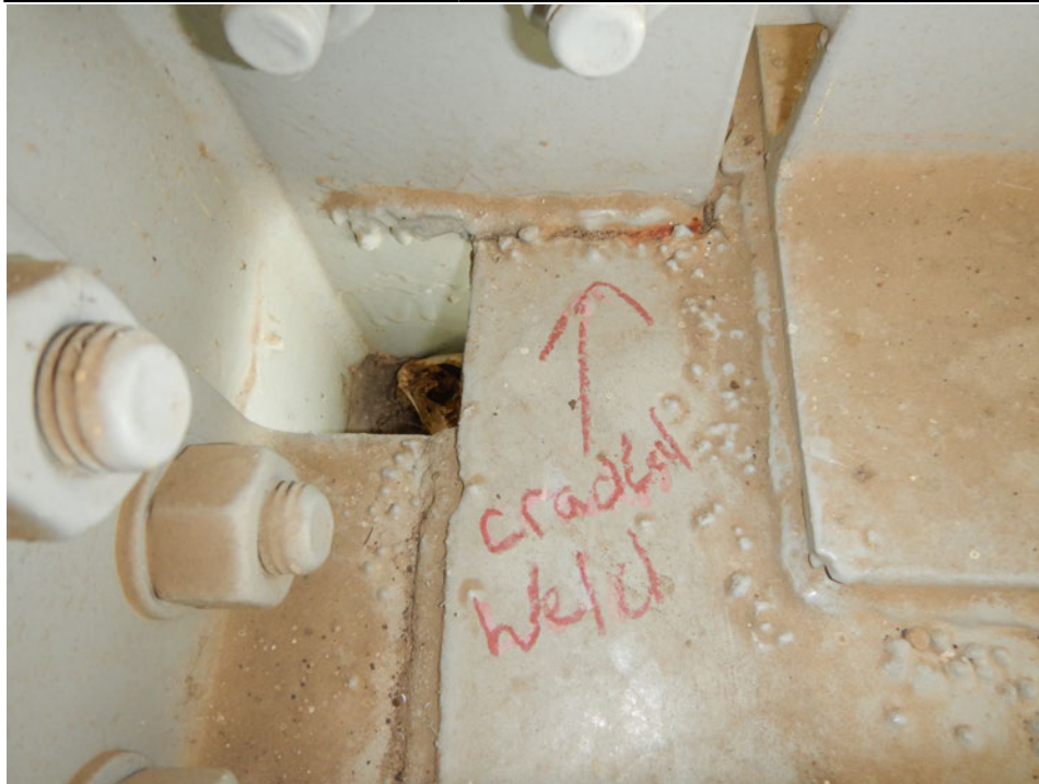
Photograph 40 - Looking west at the lower lateral bracing gusset plate connection to girder 3, span 6 at floor beam 5. Note: no change to crack along weld of the east face of the vertical stiffener to the lower lateral gusset plate.
