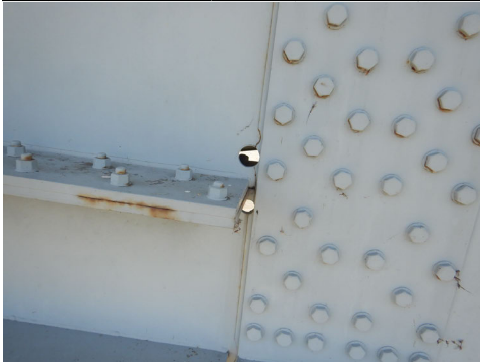
Photograph 26 - Looking south at end of the longitudinal stiffener for girder 4, span 4 near floor beam 5. Note: no change to crack in lower web arrested by drilled hole.
