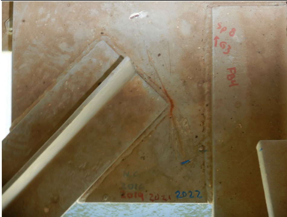
Photograph 43 - Looking south at the lower lateral bracing gusset plate for floor beam 4 at girder 3, span 8. Note: no change to cracks at lower lateral gusset plate connection to lateral bracing members.
