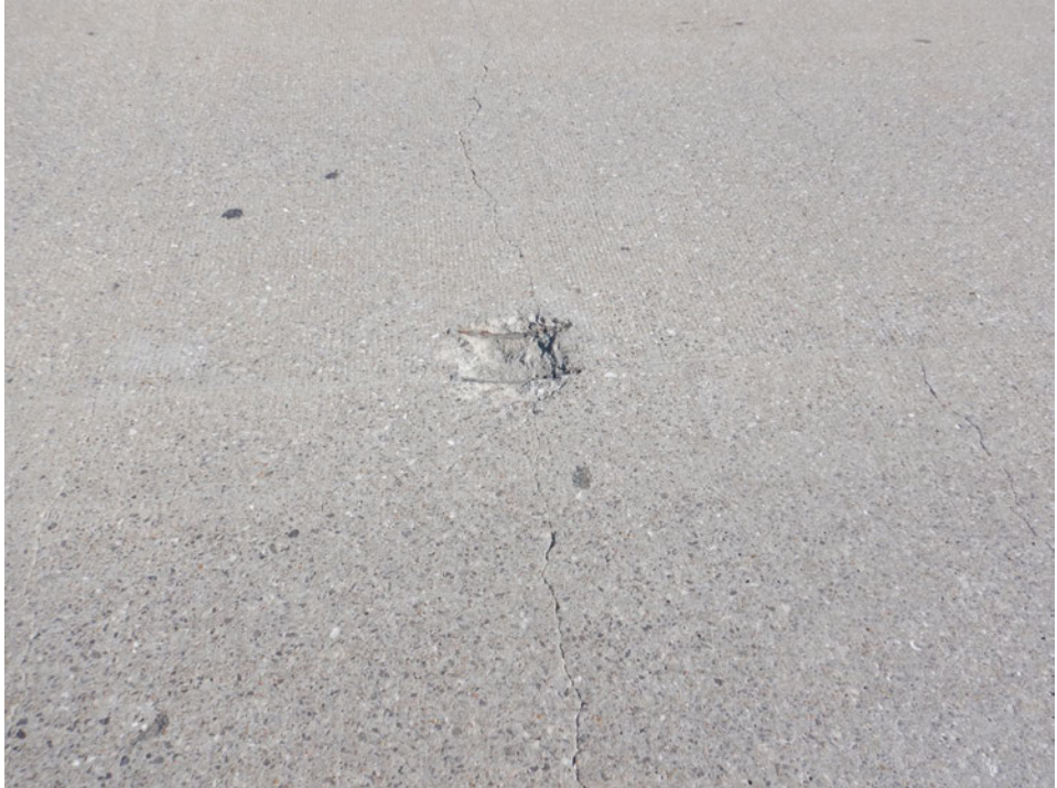
Photograph 9 - Looking north at the eastbound lanes in span 5. Note: 8-inch-diameter spall in the lane centerline.
