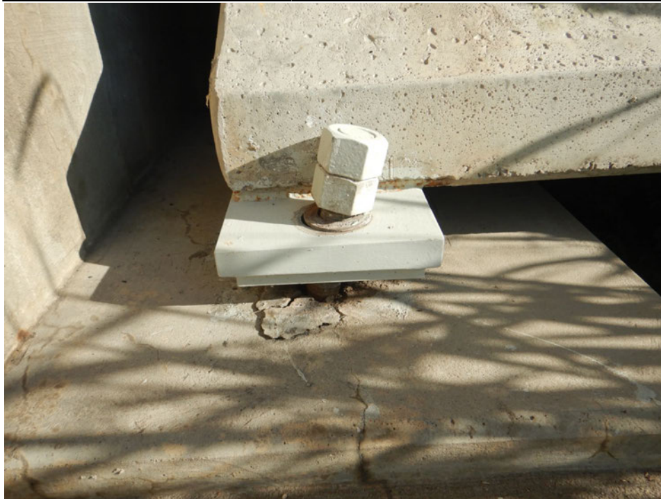
Photograph 45 - Looking north at beam 1 at the west abutment. Note: bent anchor bolt.
