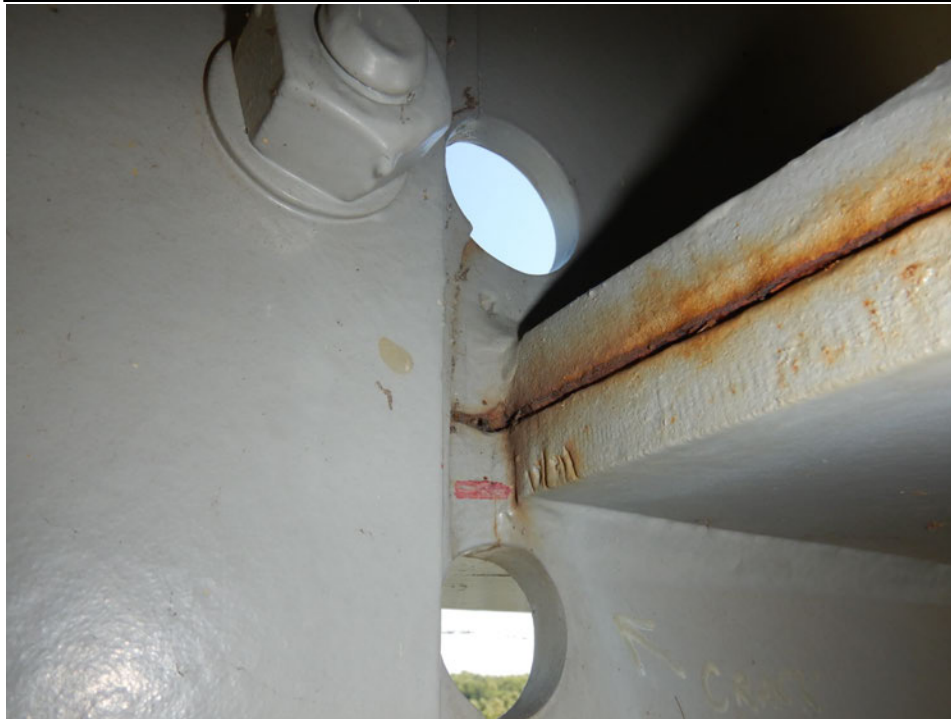
Photograph 25 - Looking north at girder 4, span 4 at end of horizontal splice near floor beam 5. Note: no change to crack in web of girder. Crack arrested by drilled holes.
