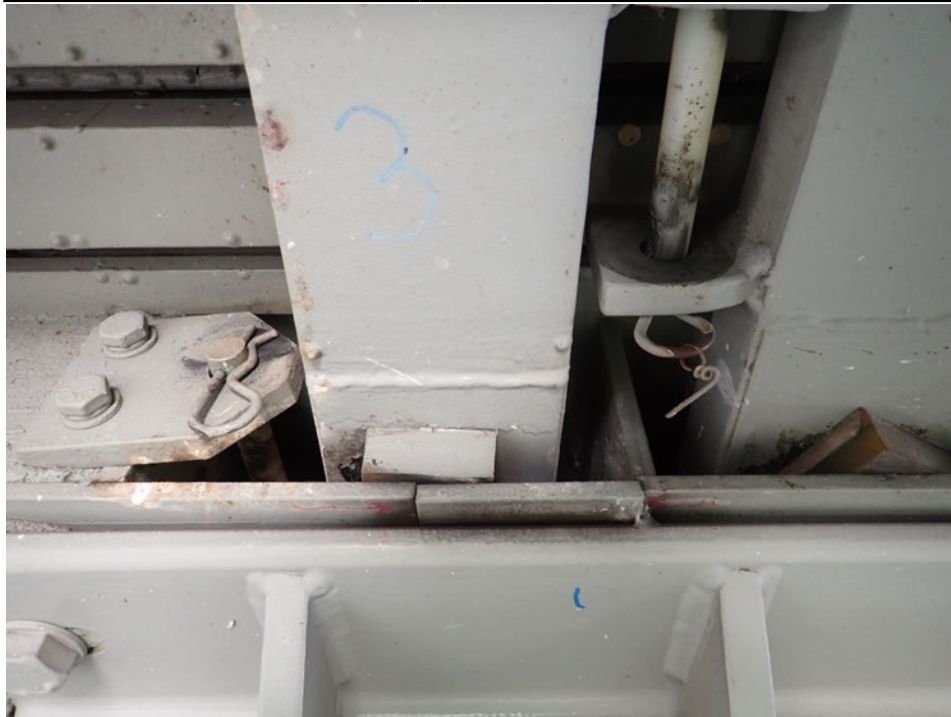
Photograph 16 - Looking east at support joint assembly 3 at the pier 3 modular joint. Note: both bottom plates of support boxes have fractured below the support bars.
