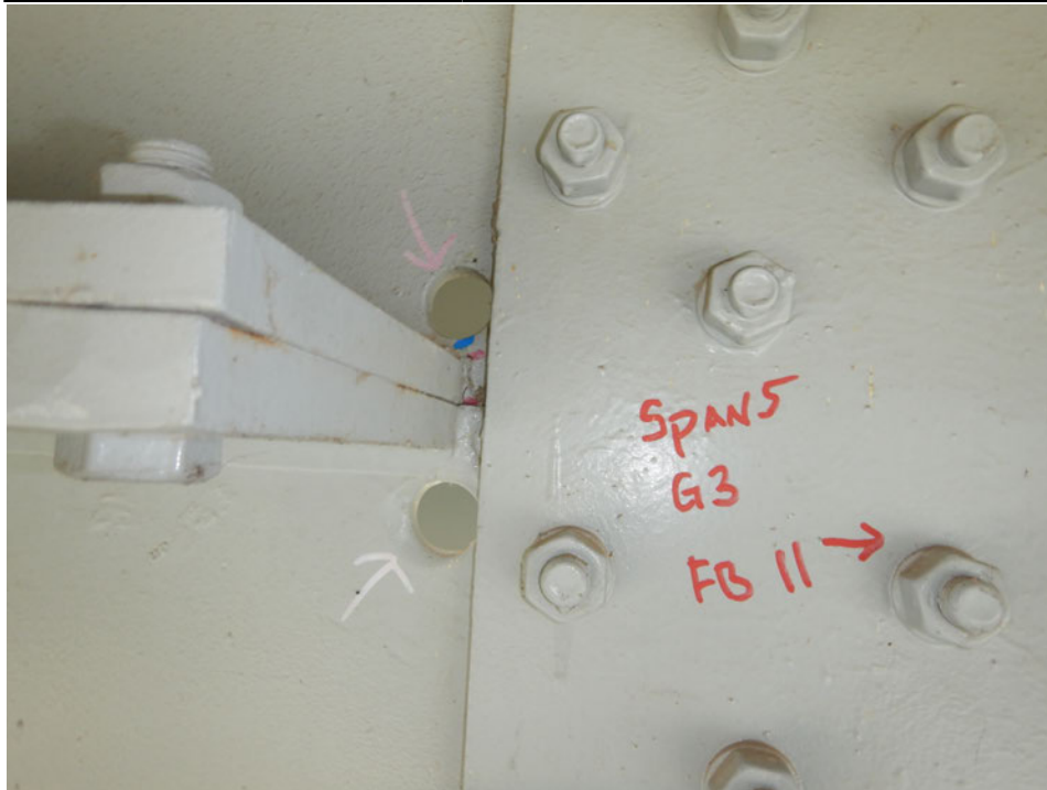
Photograph 31 - Looking south at the interior face of girder 3, span 5 near floor beam 11. Note: no change to crack at end of horizontal web splice, crack is still stopped short of arrest hole.
