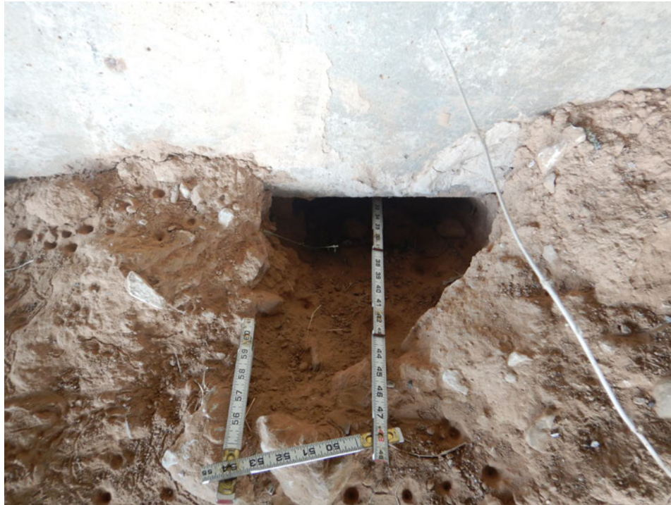
Photograph 55 - Looking west at the west abutment under beam 5. Note: 2-foot-deep erosion hole with 3 feet of penetration.
