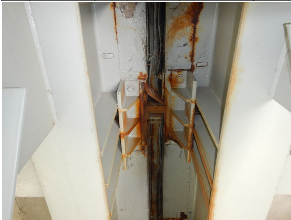
Photograph 18 - Looking north at support assembly 10 at the pier 6 modular joint. Note: no change to the one dislodged control bar.
