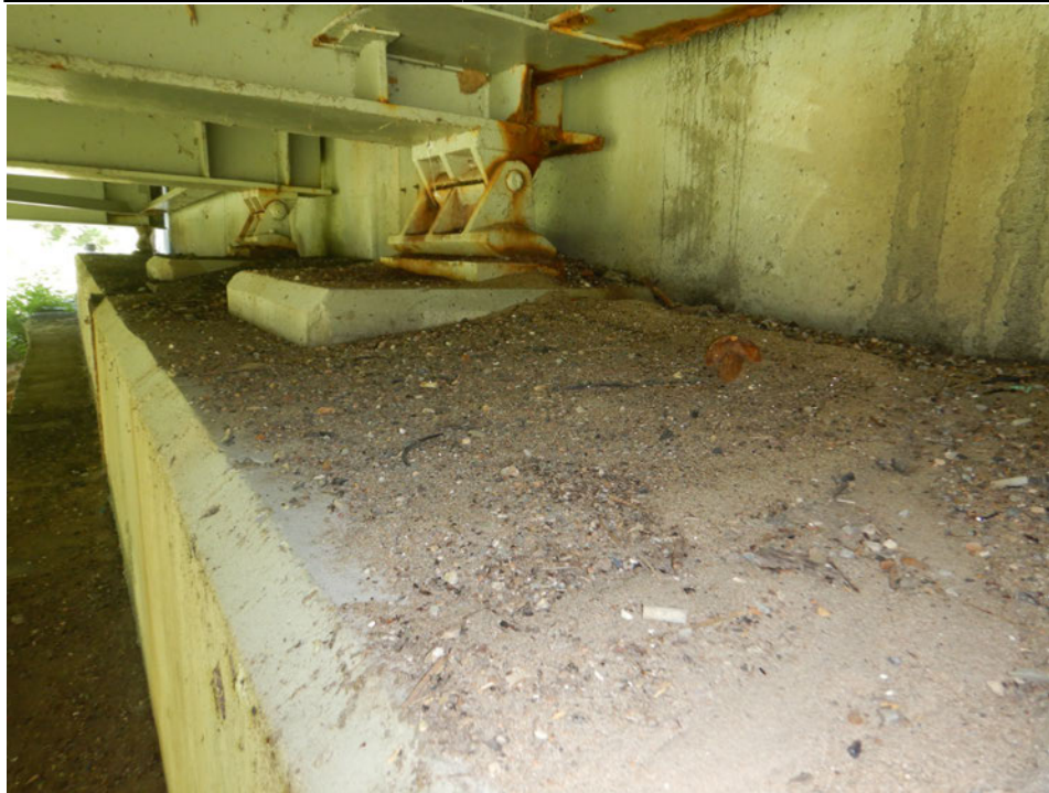
Photograph 51 - Looking northeast at the east abutment bearing seat between girders 1 and 2. Note: soil accumulation up to 4 inches high on the bearing seat.
