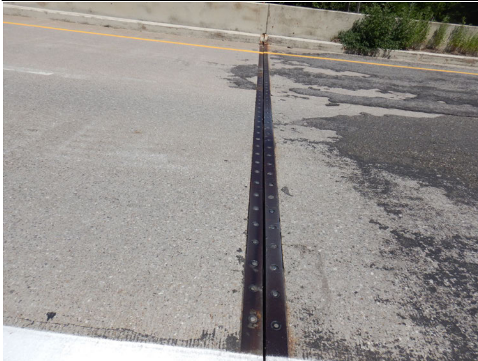
Photograph 14 - Looking north at the east abutment joint. Note: 1/2-inch vertical offset exists across the joint.
