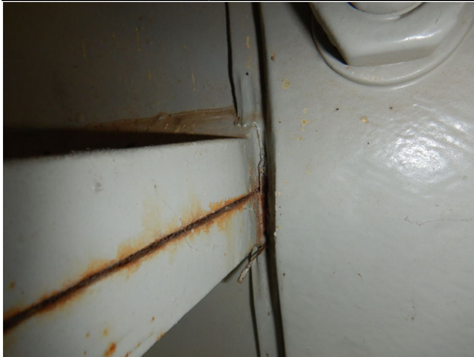
Photograph 22 - Looking south at girder 1, span 4 at end of horizontal splice near floor beam 5. Note: weld appears to be splintering. No crack observed.
