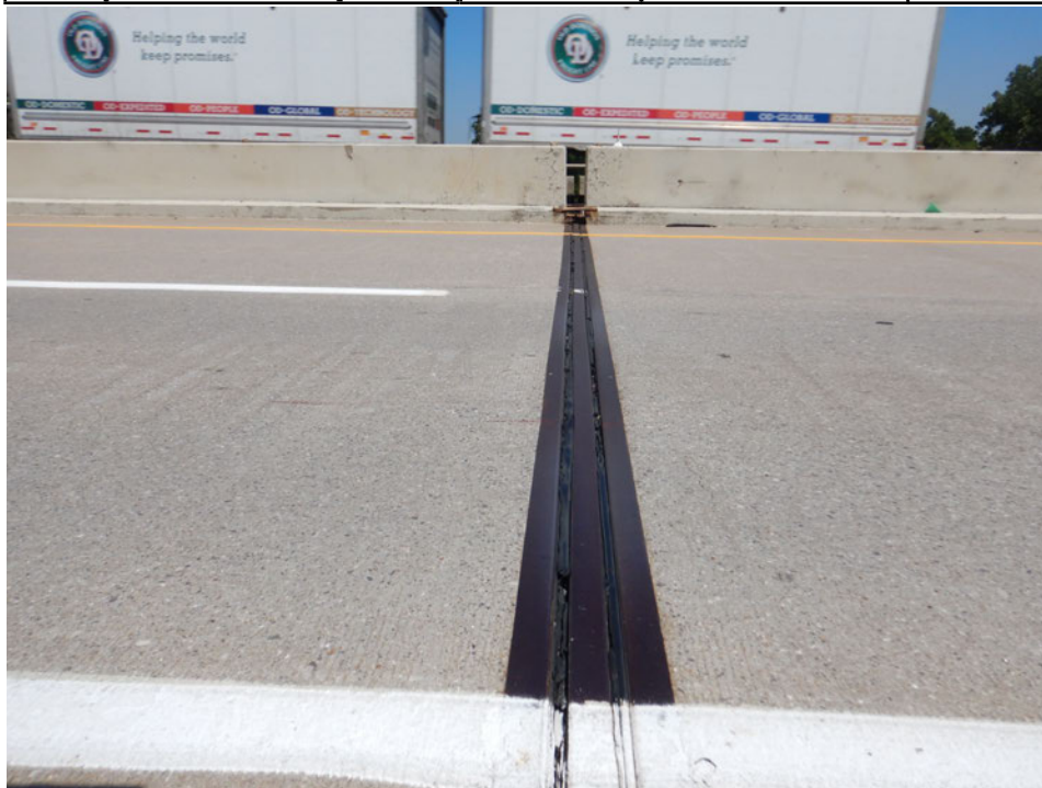
Photograph 12 - Looking north at the pier 10 joint. Note: joint open 3 3/4-inch at south curb. Joint seal torn for majority of joint.
