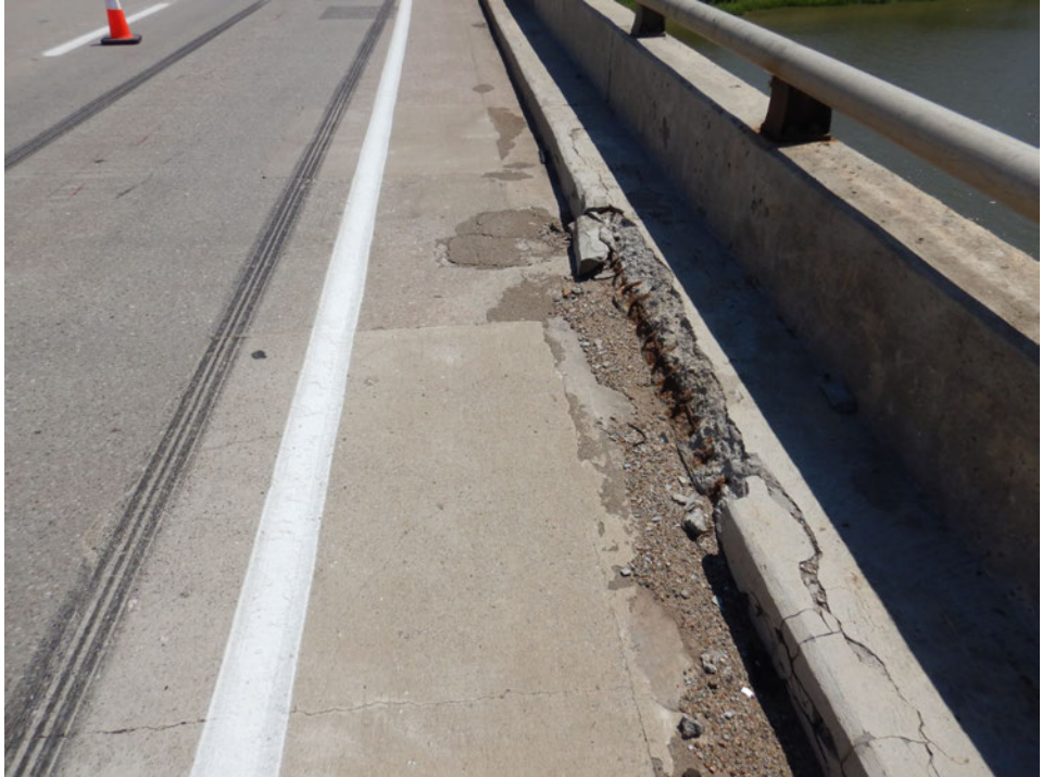
Photograph 10 - Looking east at the south curb of span 7 near pier 6. Note: two 6-foot-long spalls in the curb.
