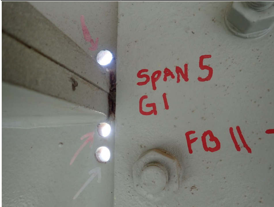
Photograph 28 - Looking south at the end of the longitudinal stiffener for girder 1, span 5 near floor beam 11. Note: no change to crack in upper web stopping short of the arrestor hole. No change to crack in lower web arrested by two 1/2-inch diameter drilled holes.
