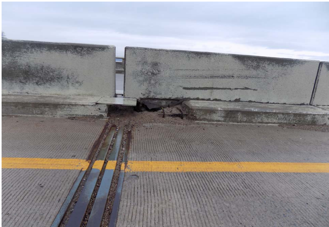
Modular Expansion Joint in Deck Slab
