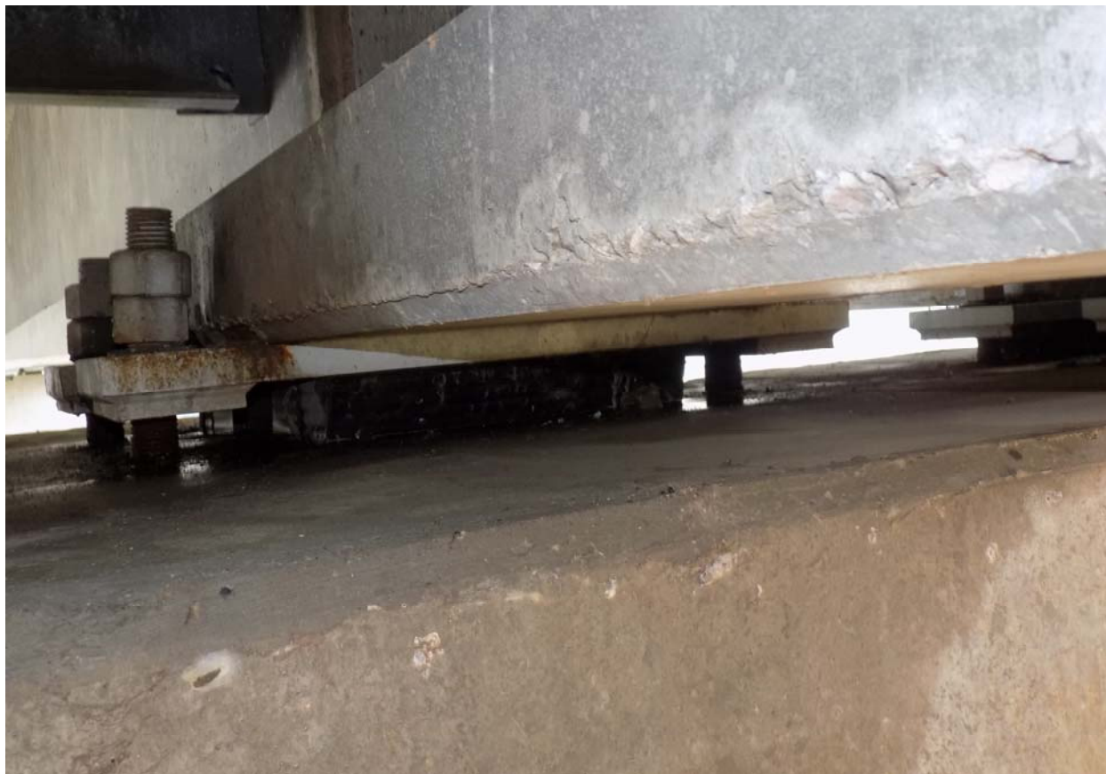
Painted Weathering Steel Bearing Assembly
