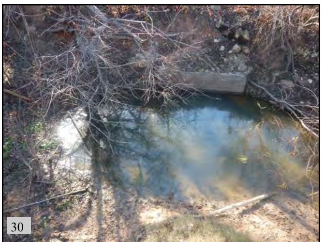
▲ (PS 7): View of flooded structure that OW 4a, 4b, and OW 5 flow into. View is to the south.
