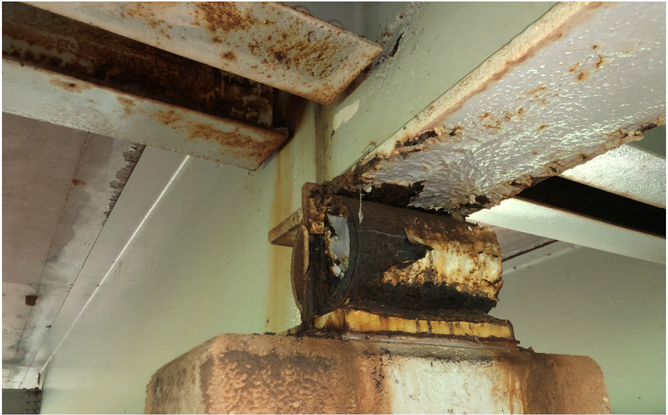
Fig. 7: Corrosion and Section Loss at Bearing and Beam End, West Pier.
