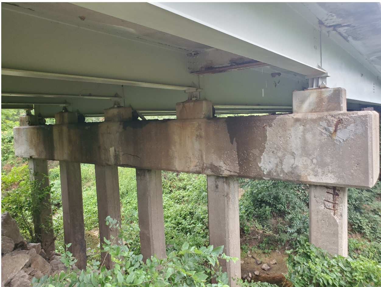
Fig. 12: Pier 1 – Pier 2, Facing West. Cracking in Cap. Spall at North Pile. Note water infiltration through deck joint.
