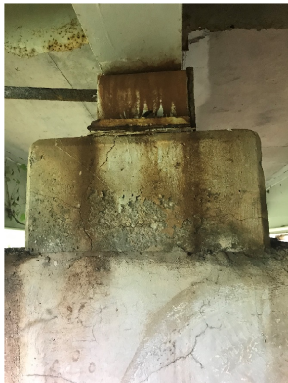
Fig. 15. Cracks in Pedestal, Pier 2
