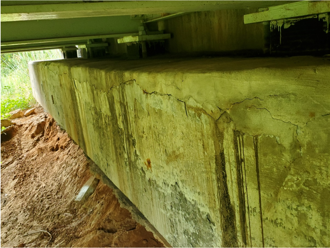
Fig. 10a: Longitudinal Cracking in face of Abutment Seat (Abutment 2, Facing Northeast)
