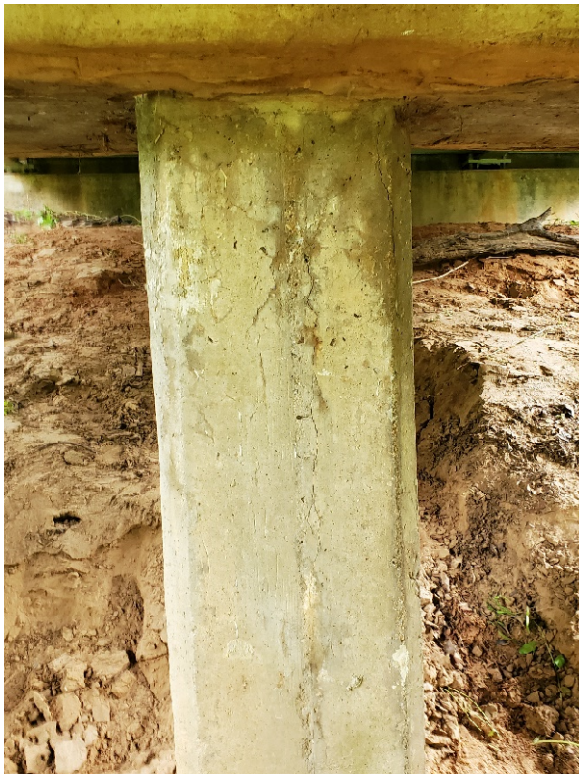
Fig. 14. Vertical Crack in Concrete Pile, Pier 1
