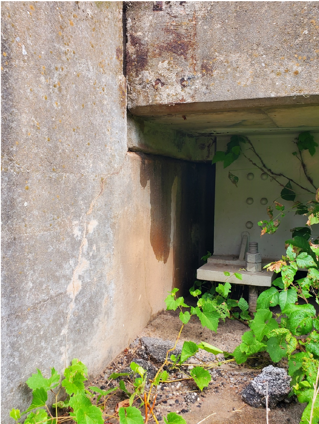
Fig. 11: Crack and Water Infiltration at Backwall, Abutment 1, South End.
