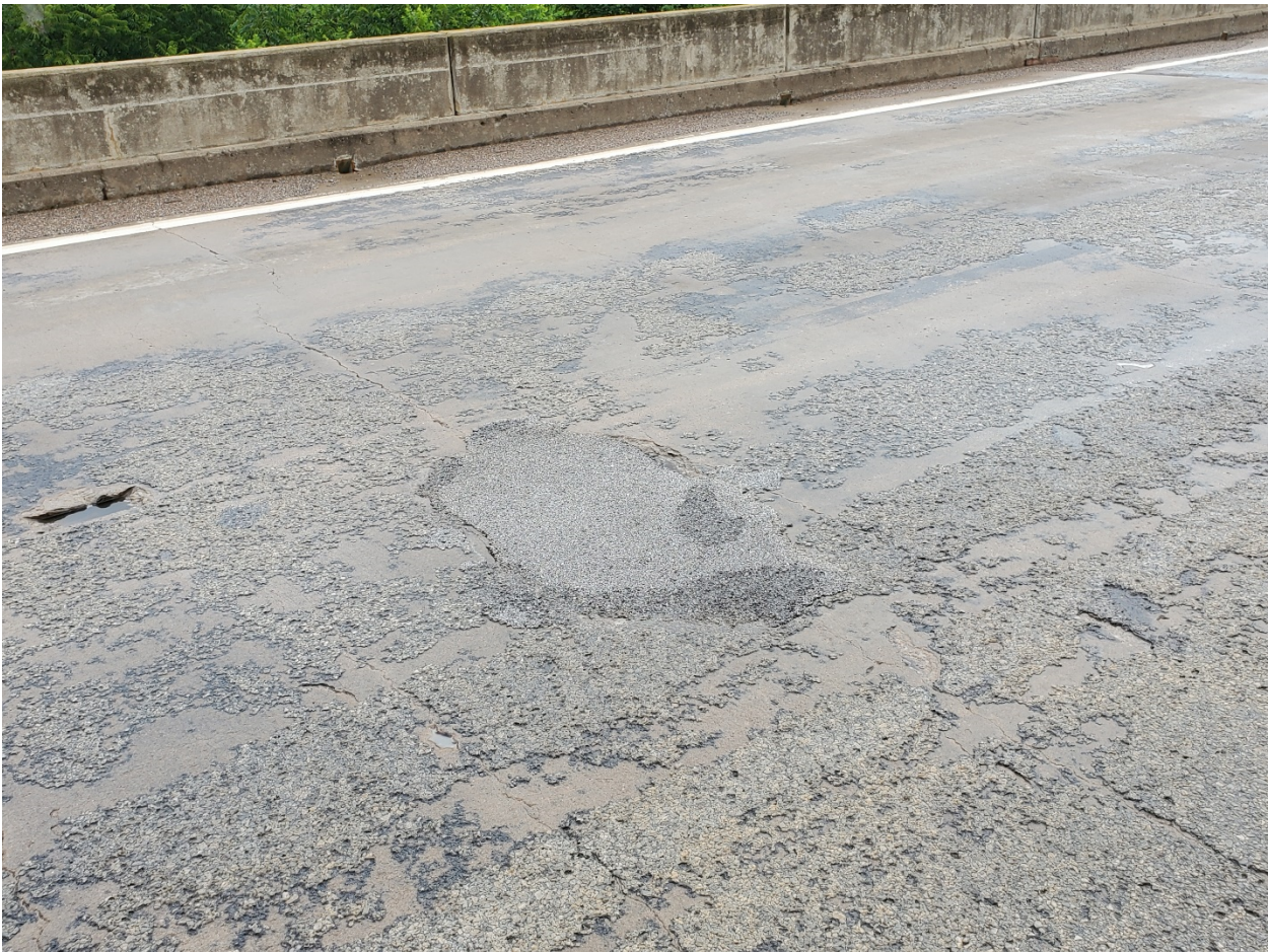
Fig. 1: Pop-outs and Pothole Repairs. Transverse Cracking in Deck. Deteriorated asphalt wearing surface.
