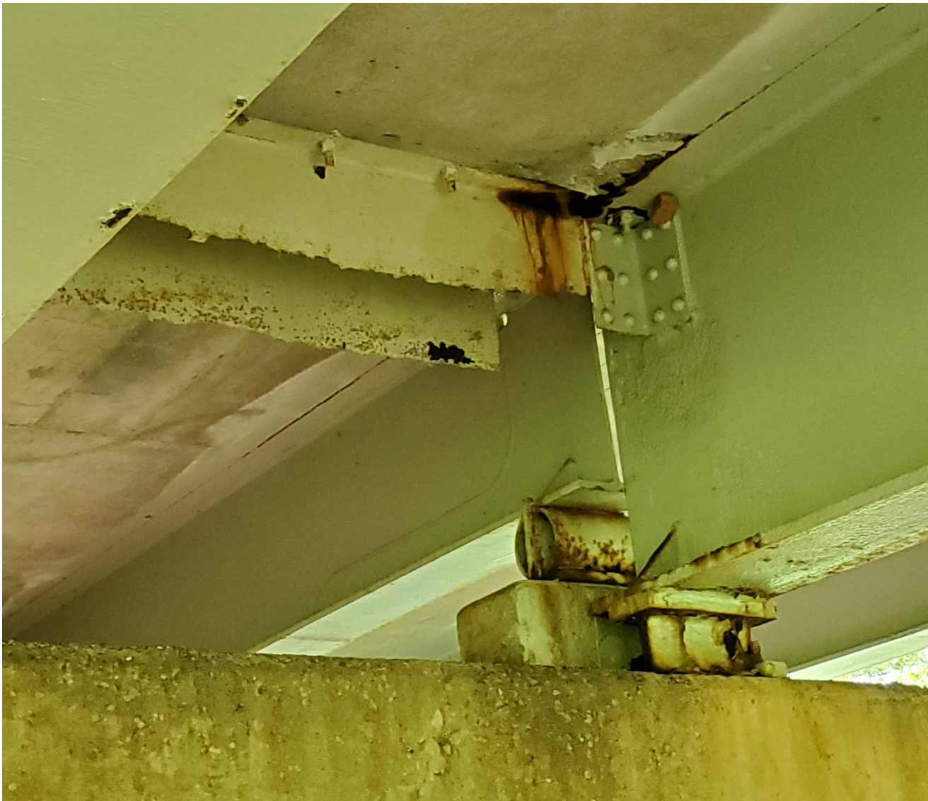
Fig. 6: Corrosion and Beam Ends and Diaphragms. Corrosion at top flange of beam. Some (previously painted) section loss at bottom flange of beam, complete section loss at bottom flange of end diaphragms. Corrosion at Bearings. Previously Repaired Beam End
