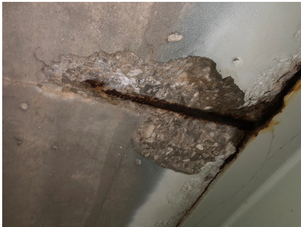
Fig. 3: Pop out with exposed Reinforcing Steel on Underside of Deck. Note corrosion of Top Flange.
