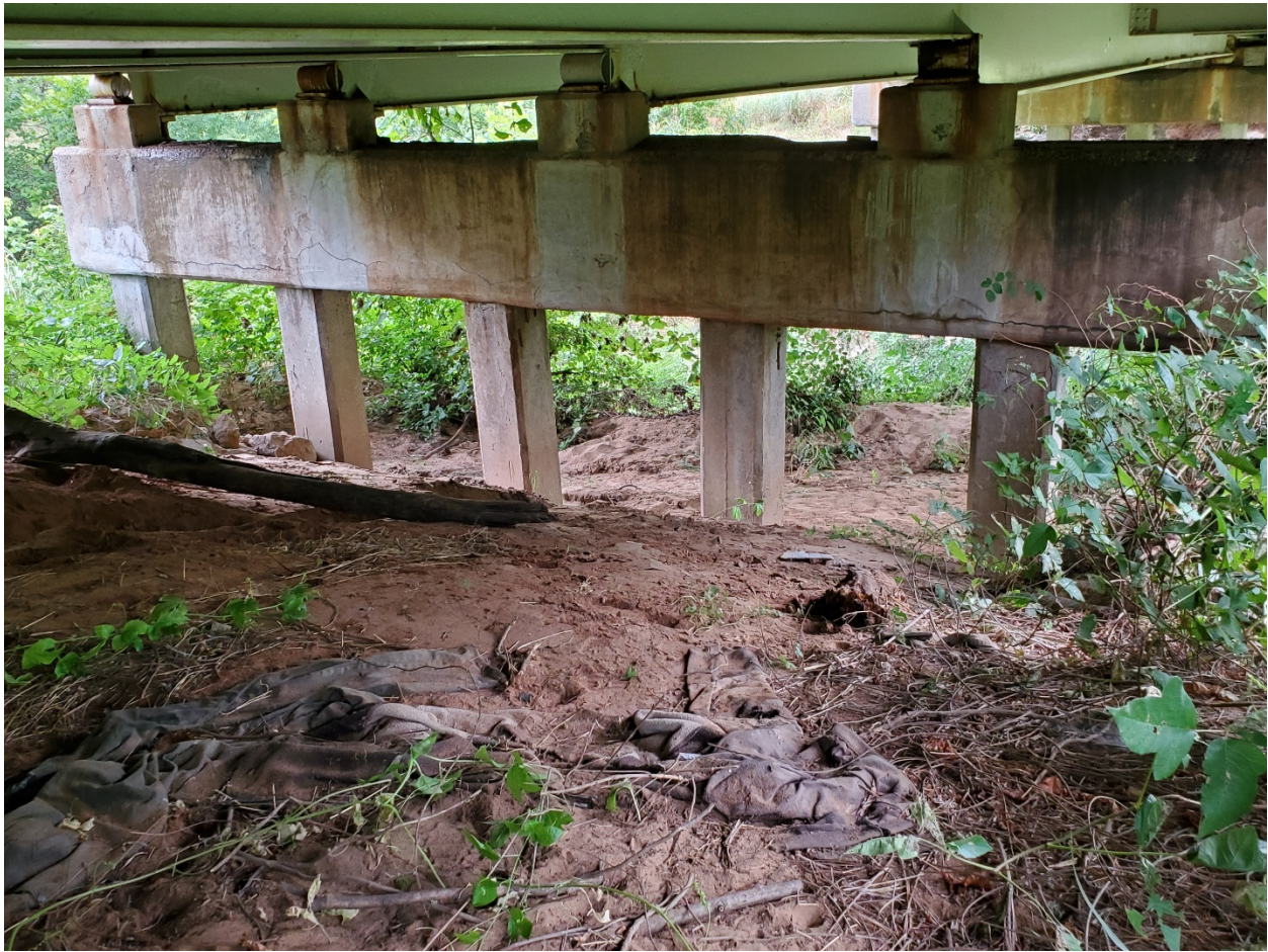
Fig. 13. Pier 1, Facing East. Longitudinal crack along bottom edge
