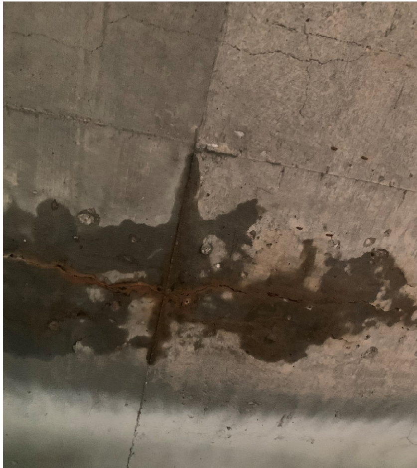
Fig. 2: Cracking, Efflorescence, and active leaking at Underside of Deck. (Condition common throughout)
