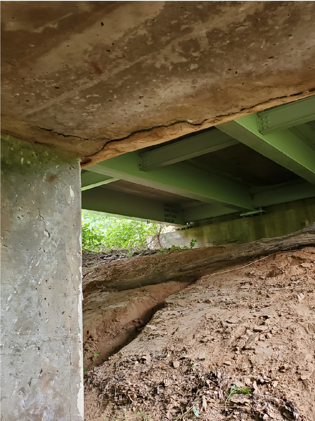
Fig. 16. Cracking in Concrete Pile and underside of Pier Cap. Pier 1, Facing West
