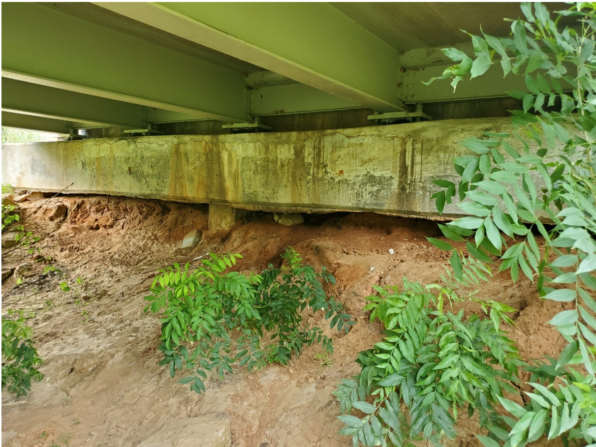
Fig. 9: Cracking in Abutment Seat and Exposed Piles at Abutment 2
