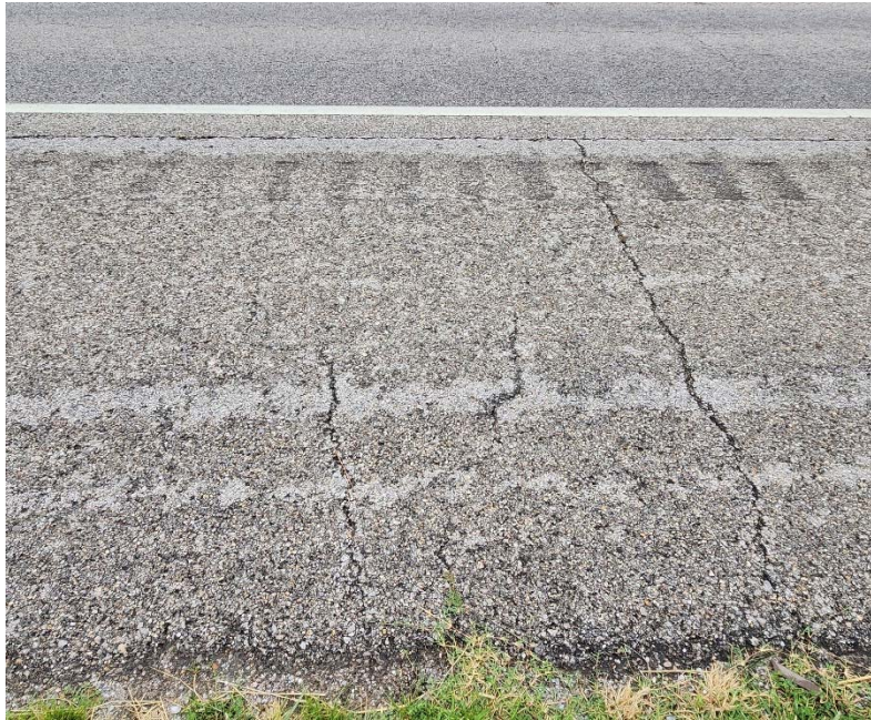
Photo #7 Minor to moderate severity transverse cracking near C-7.
