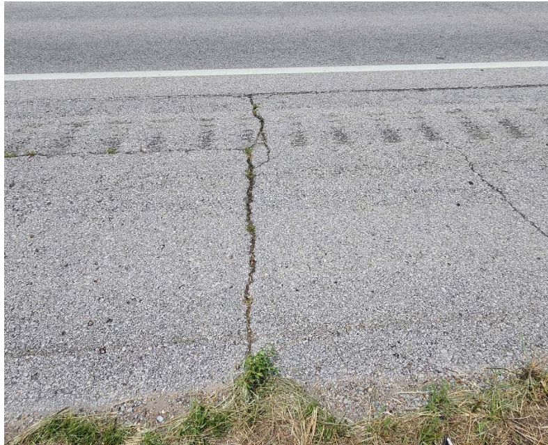
Photo #23 Moderate severity transverse cracking near C-23.
