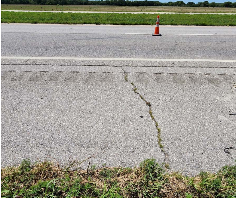
Photo #25 Moderate severity transverse cracking near C-25.
