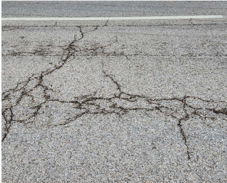
Photo #5 Moderate to major severity fatigue cracking near C-5.
