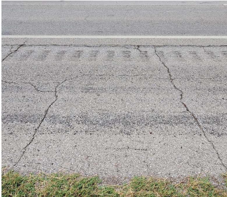
Photo #11 Minor to moderate severity longitudinal and transverse cracking near C-11. Also note the light severity asphalt bleeding.
