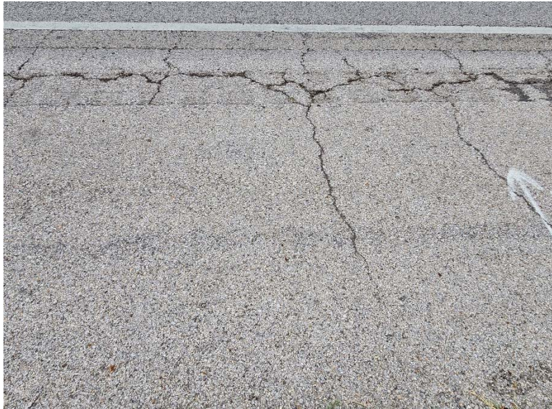
Photo #9 Moderate severity fatigue and transverse cracking near C-9. Also note the light severity asphalt bleeding.
