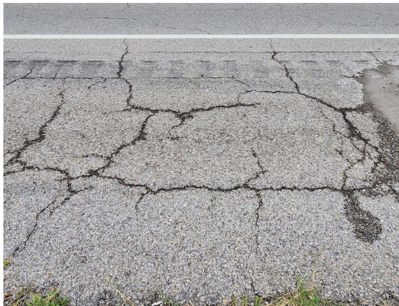
Photo #2 Major severity fatigue cracking near C-2.
