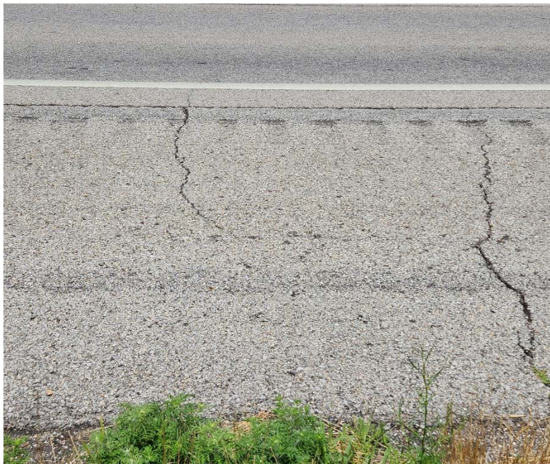
Photo #8 Minor to moderate severity transverse cracking near C-8. Also note the light severity asphalt bleeding.
