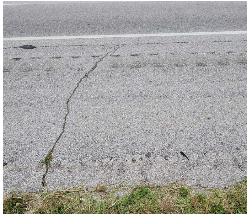
Photo #24 Moderate severity transverse cracking near C-24. Also note the light severity asphalt bleeding.
