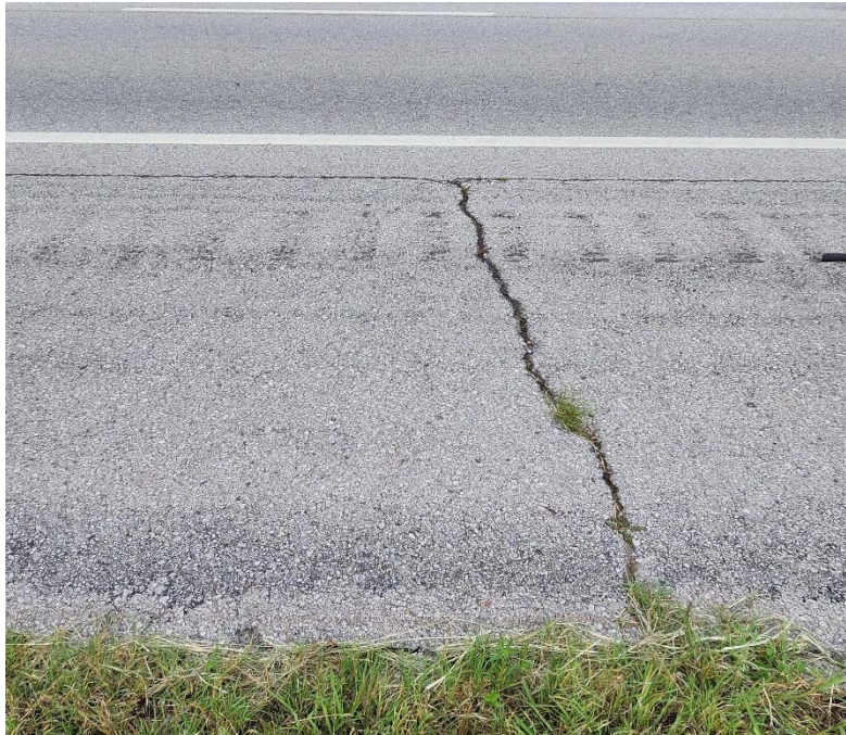
Photo #21 Moderate severity transverse cracking near C-21. Also note the light severity asphalt bleeding.
