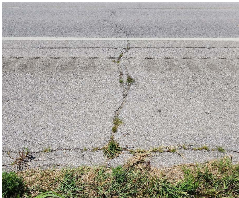
Photo #26 Moderate severity longitudinal and transverse cracking near C-26.
