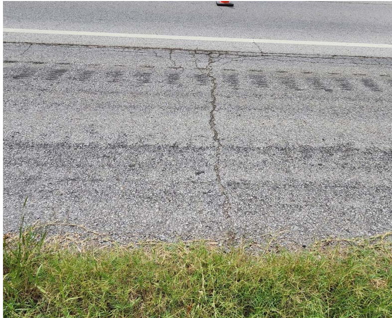
Photo #13 Minor to moderate severity transverse cracking near C-13. Also note the light severity asphalt bleeding.
