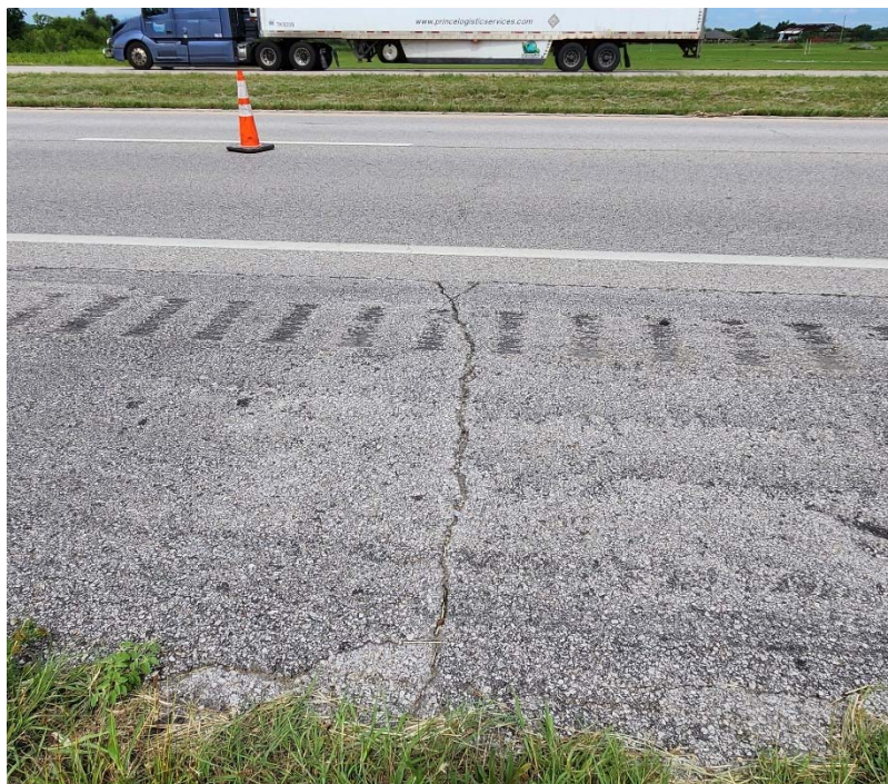
Photo #20 Minor to moderate severity transverse cracking near C-20. Also note the light severity asphalt bleeding.
