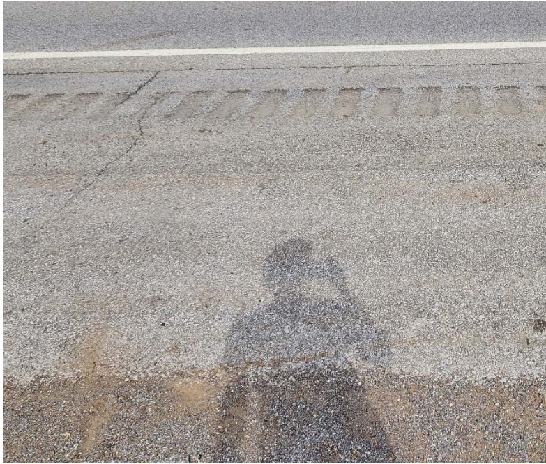
Photo #17 Minor severity transverse cracking near C-17.
