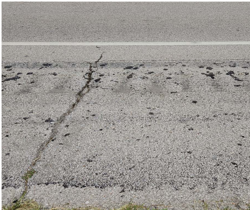
Photo #18 Moderate severity transverse cracking near C-18. Also note the light severity asphalt bleeding.
