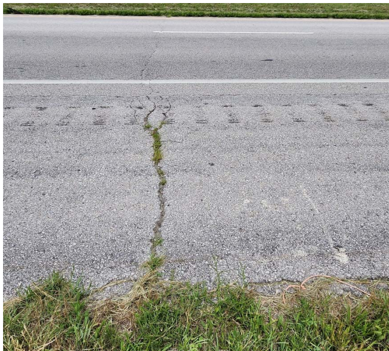
Photo #22 Moderate severity transverse cracking near C-22. Also note the light severity asphalt bleeding.
