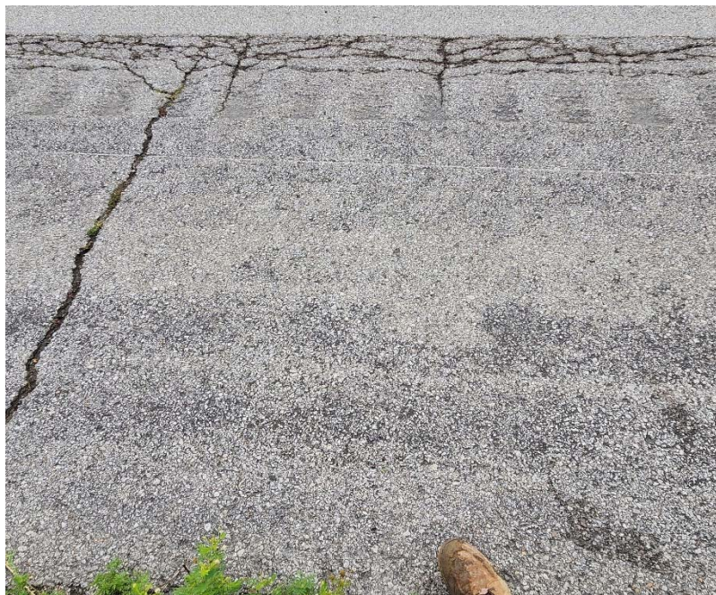
Photo #16 Moderate severity fatigue and transverse cracking near C-16. Also note the light severity asphalt bleeding.
