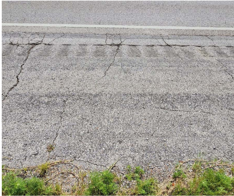
Photo #15 Minor to moderate severity fatigue and transverse cracking near C-15. Also note the light severity asphalt bleeding.
