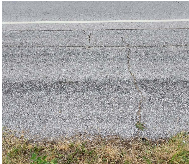
Photo #14 Minor to moderate severity transverse cracking near C-14. Also note the light severity asphalt bleeding.
