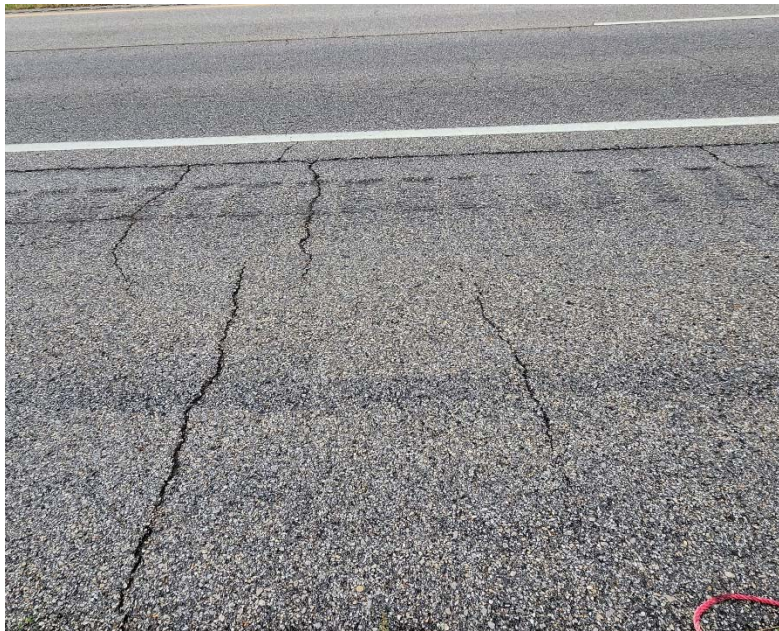
Photo #6 Minor to moderate severity transverse cracking near C-6. Also note the light severity asphalt bleeding.
