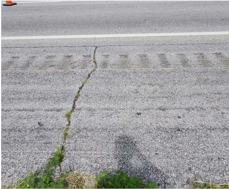
Photo #19 Moderate severity transverse cracking near C-19. Also note the light severity asphalt bleeding.
