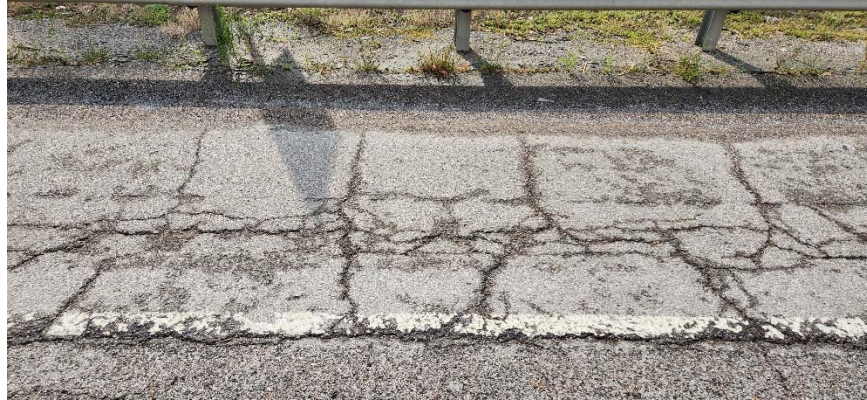
Photo #1 Major severity fatigue and transverse cracking near C-1.
