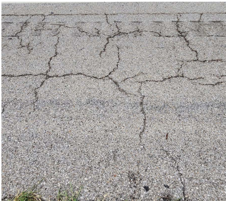
Photo #10 Moderate severity fatigue cracking near C-10. Also note the light severity asphalt bleeding.
