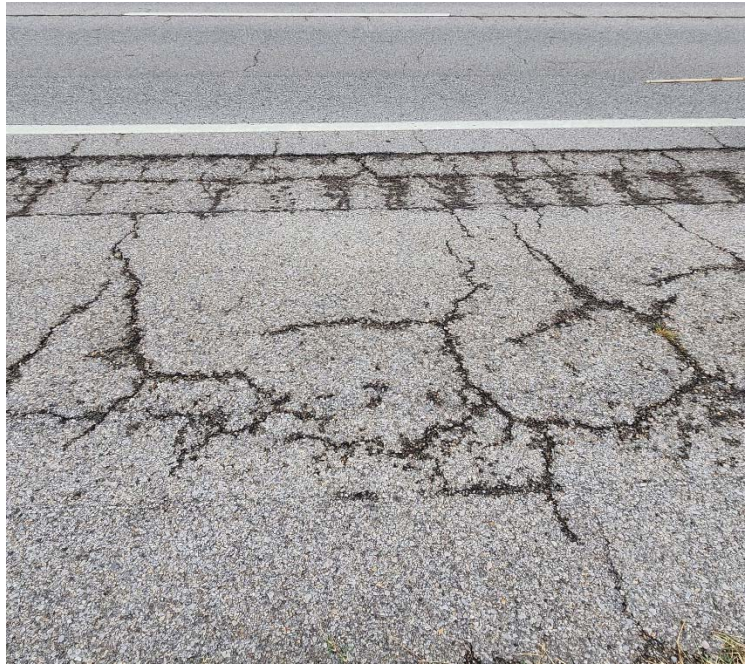
Photo #3 Moderate to major severity fatigue cracking near C-3.
