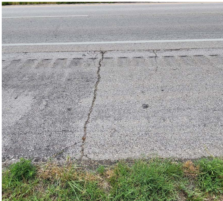
Photo #12 Moderate severity transverse cracking near C-12. Also note the light severity asphalt bleeding.
