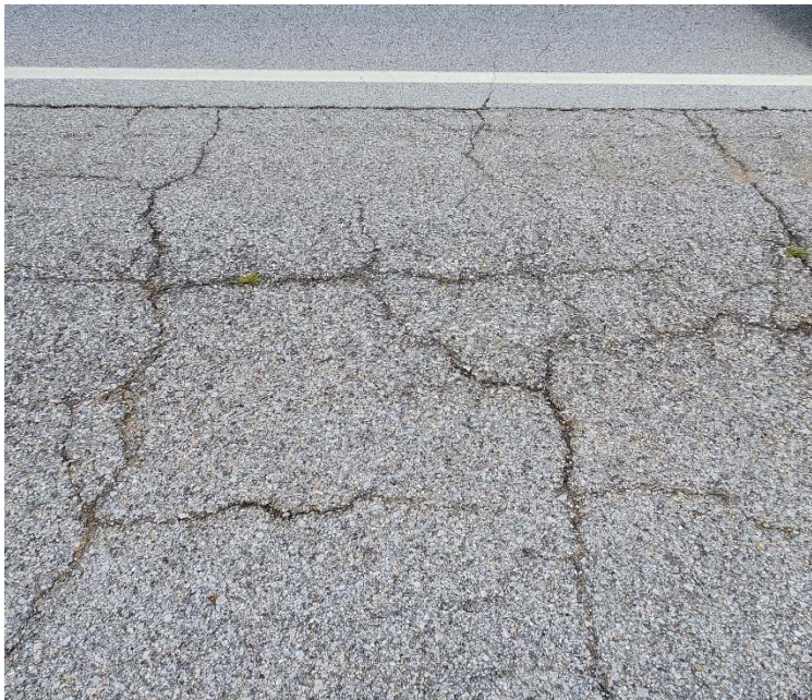
Photo #4 Moderate severity fatigue cracking near C-4.
