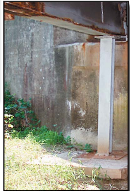
No shoulders Narrow bridge
