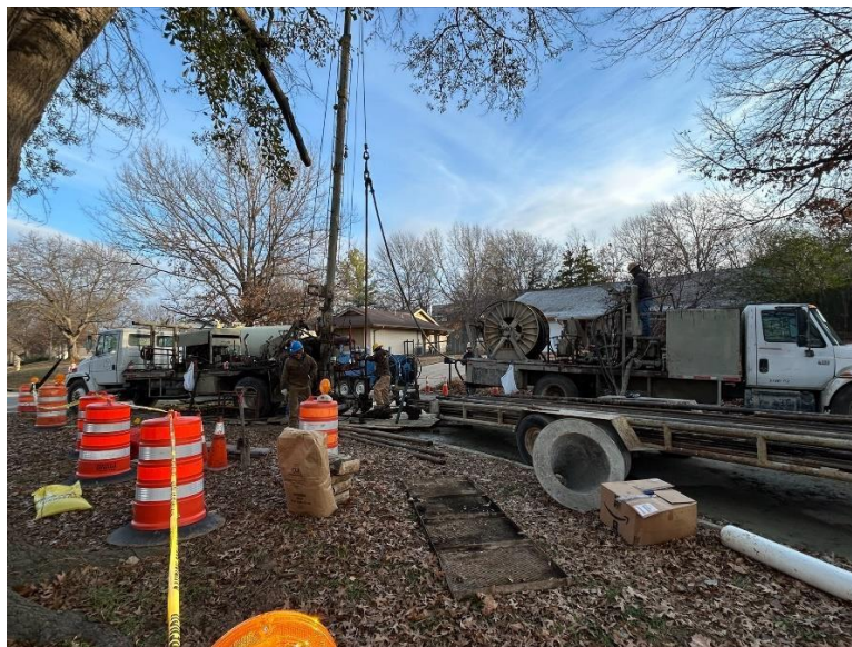
Plugging a Category 1 emergency SFL well (the “Mabel Castillo”) under a Tulsa neighborhood street, January 1, 2025
