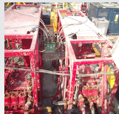
Rented, Ragged out Triplex Pumps
