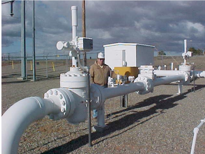
An orifice meter is used to measure CO 2 at the inlet to the Cortez PL
