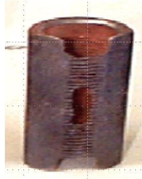
Corroded Tubing Coupling
