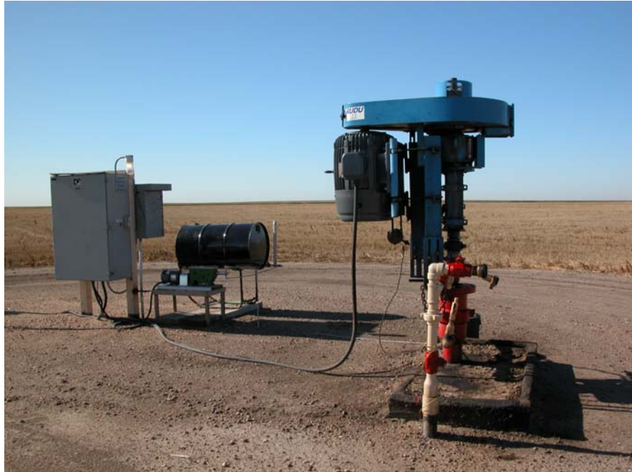
VIEW OF A PROGRESSIVE CAVITY PUMP AT A PRODUCTION WELL HEAD
