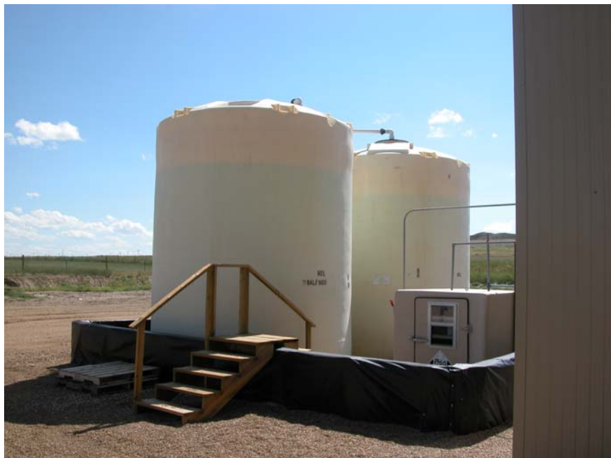
VIEW OF THE ACID FEED TANKS
