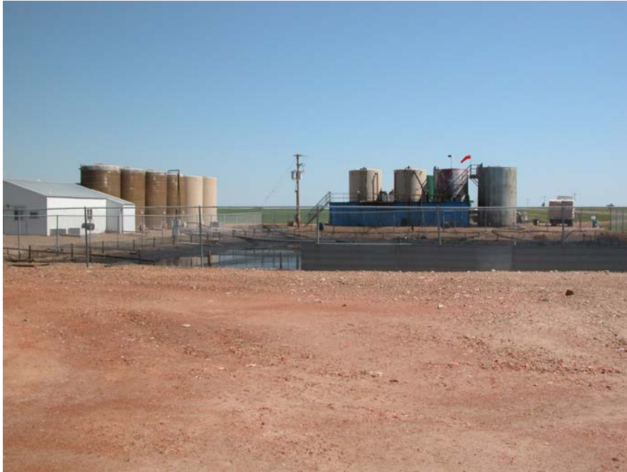
VIEW OF INJECTION WELLHEAD AT NANCE
