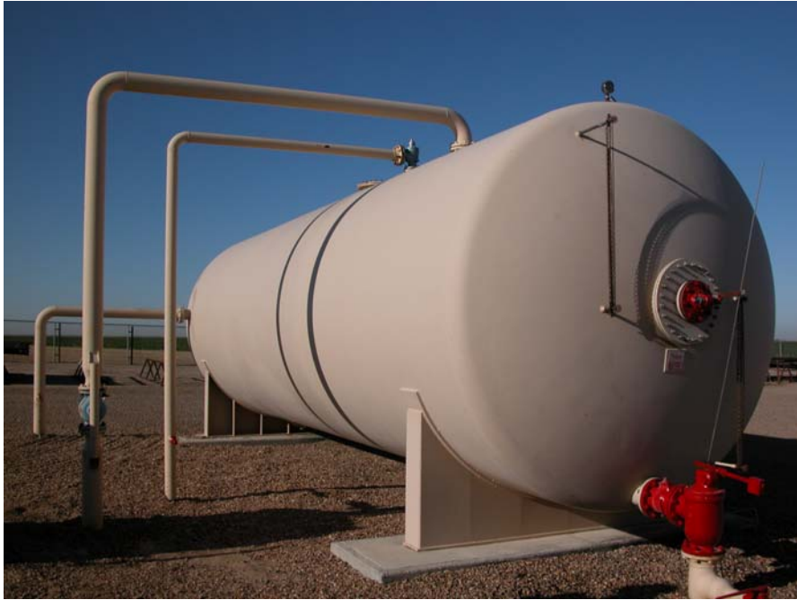
VIEW OF A THREE PHASE SEPARATOR TANK AT PETROSANTANDER
