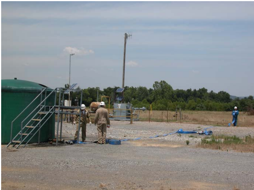
VIEW OF THE TEMPORARY INSTALLATION OF THE FLOOD IRRIGATION SYSTEM
