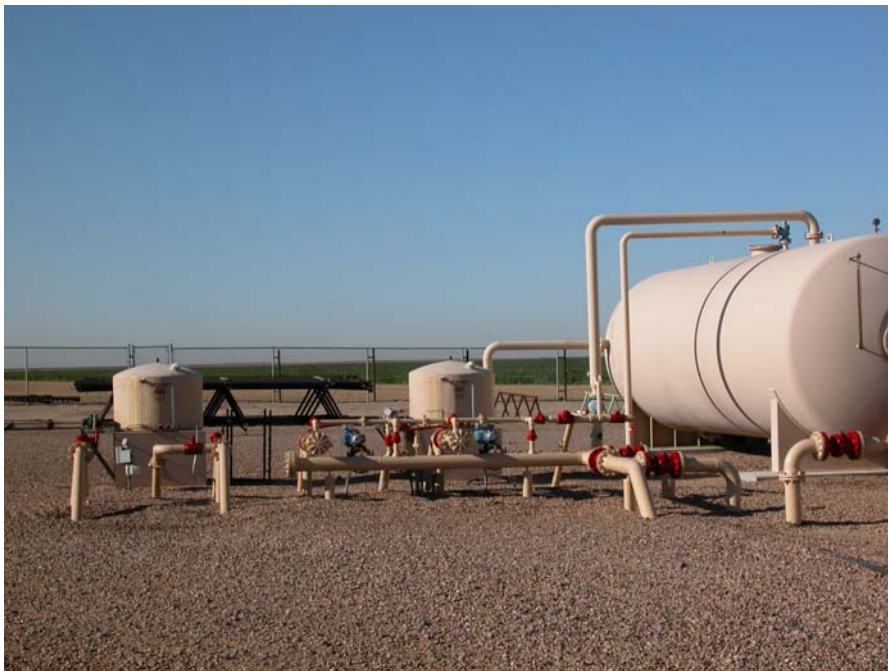
VIEW OF THE CHEMICAL INJECTION TANKS THAT TREAT THE WATER BEFORE STORAGE
