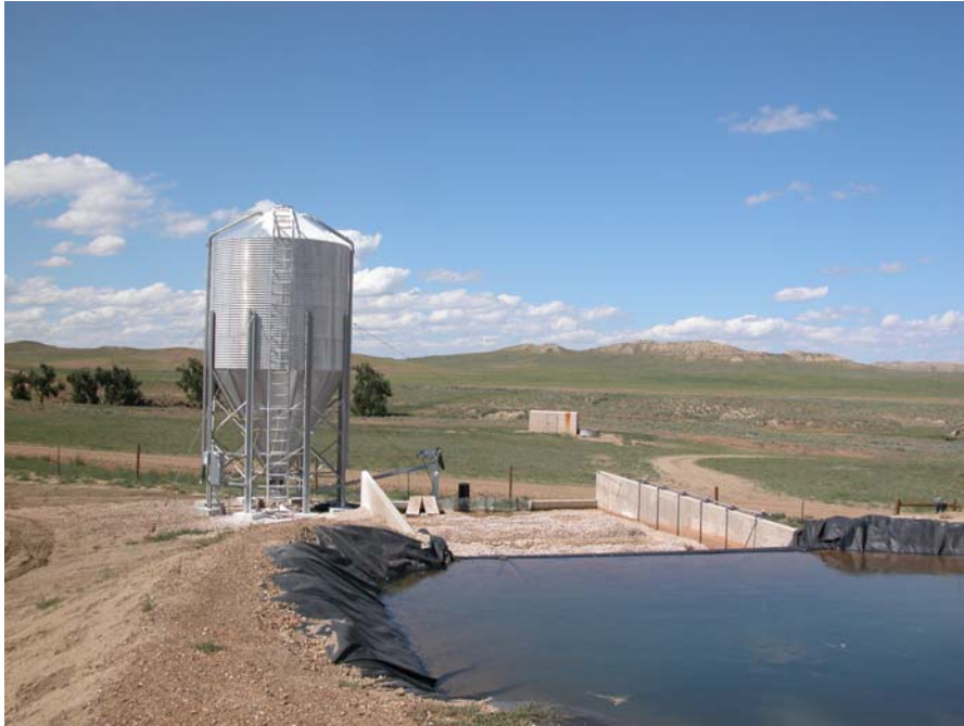
VIEW OF A LIME REACTOR BED TO ADJUST pH PRIOR TO DISCHARGE
