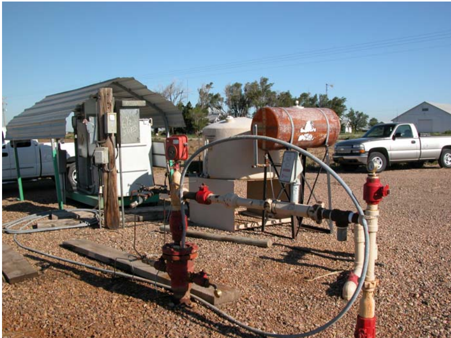
VIEW OF A WATER SUPPLY WELL THAT PROVIDES MAKEUP WATER
