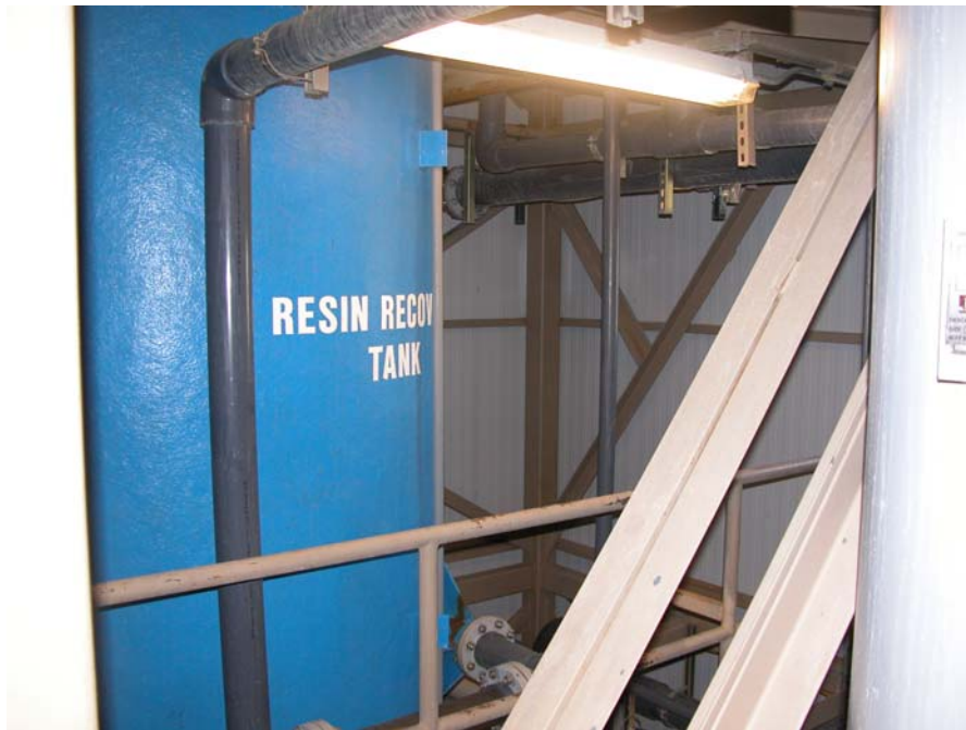
VIEW OF THE RESIN RECOVERY TANK
