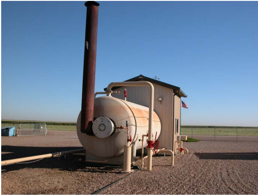
VIEW OF THE HEATER TREATER THAT SEPARATES THE WATER FROM THE OIL
