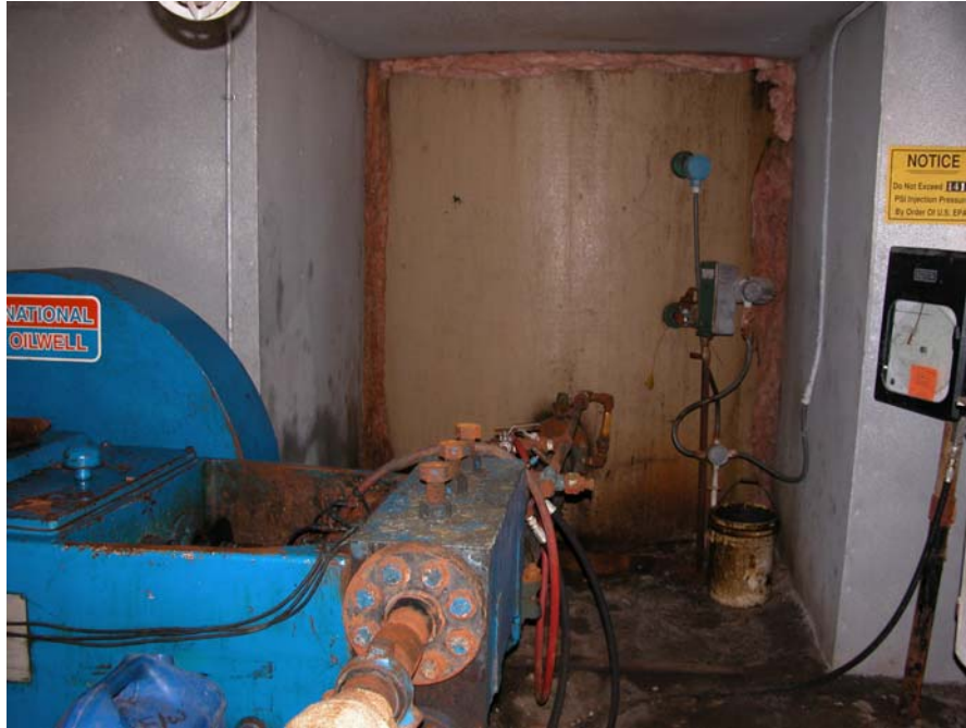
VIEW OF A TANK WITH THE WELL HEAD HOUSED NEXT TO IT
