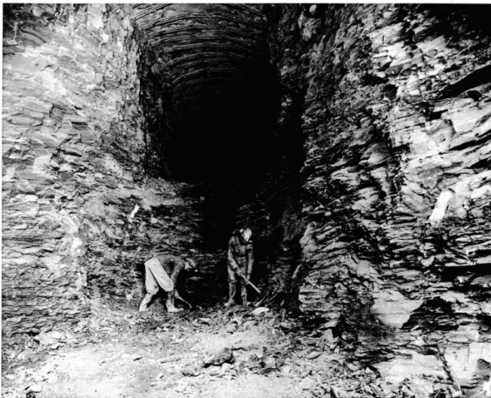
Figure 5-1 is a photograph of a hard rock cavern under construction in shale in Middletown, Ohio in 1959. Source: http://caplaconference.com/wp-content/uploads/2015/04/Pipelines .
