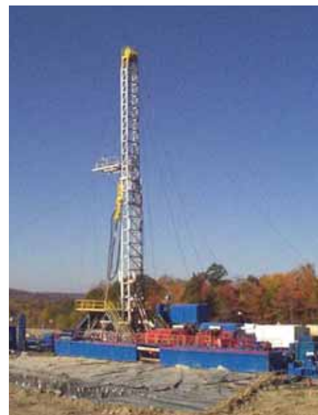
Through year-end 2004, New York's Trenton/Black River wells produced more than 110 Bcf of natural gas.
