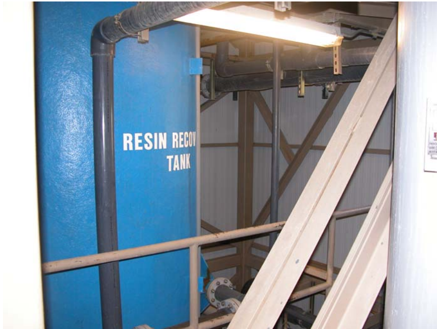
VIEW OF THE RESIN RECOVERY TANK
