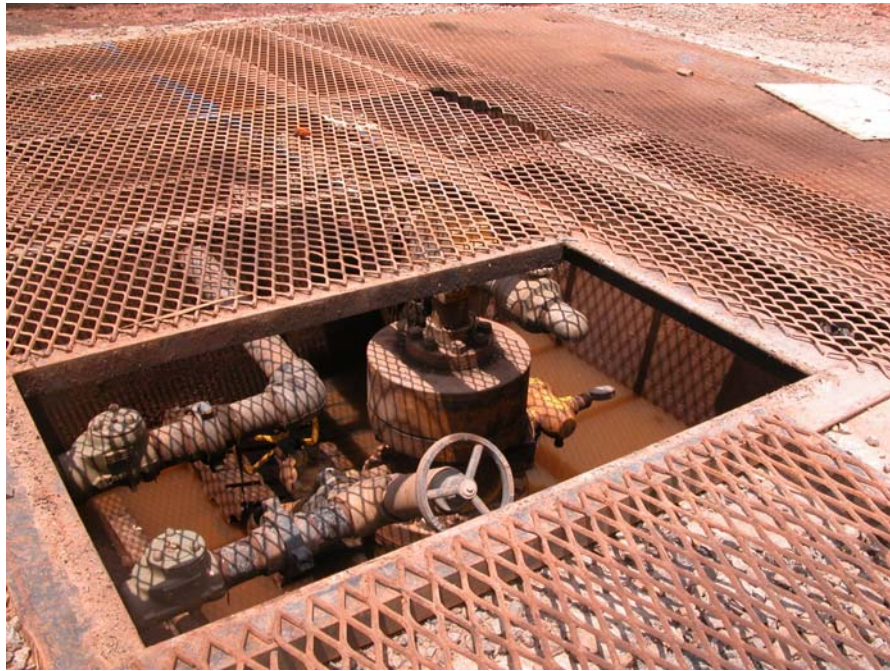
VIEW OF THE WELL HEAD OF A PRODUCING WELL
