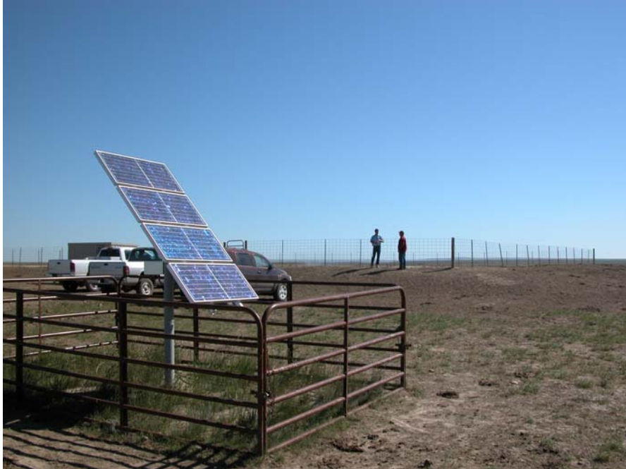
VIEW OF SOLAR PANEL AT REMOTE WELL LOCATION
