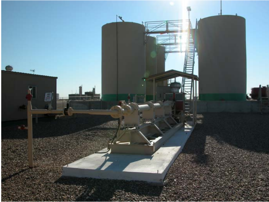
VIEW OF THE STORAGE TANKS AND ONE OF THE PUMPS
