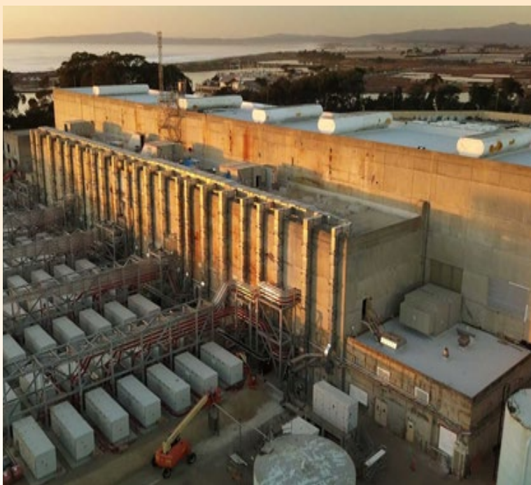
Vistra Energy’s Lithium-ion battery system Moss Landing, CA
