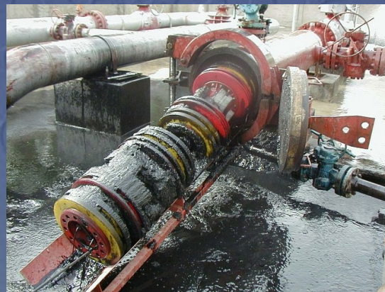
Pipeline Pigging – data driven corrosion inhibitor schedule*
