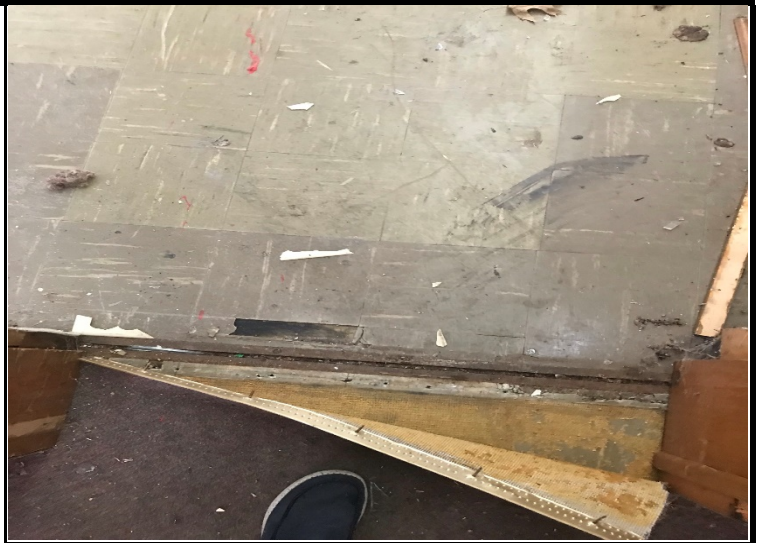
Photo 2: Asbestos Containing Floor Tile & Mastic Building B Room 10
