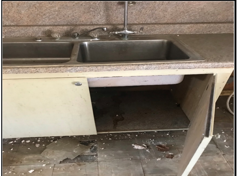
Photo 6: Asbestos Containing Sink Undercoat Building B Room 11
