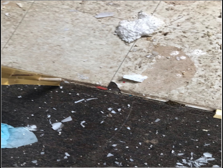
Photo 16: Asbestos Containing Floor Tile Mastic Under 12x12 Floor Tile Building C Room 24
