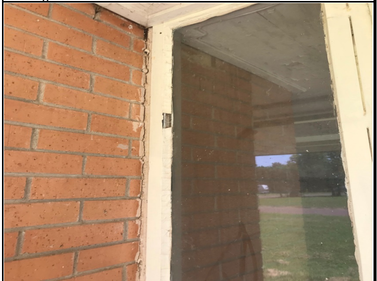
Photo 12: Asbestos Containing Window Glaze Building A South Side
