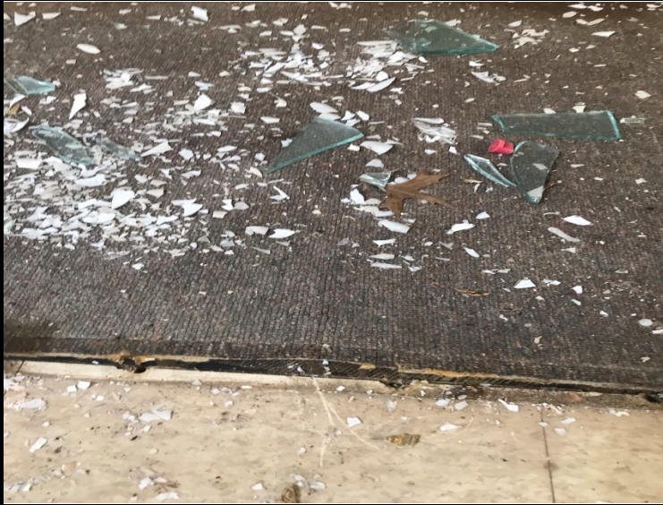
Photo 15: Asbestos Containing Floor Tile & Mastic Under Carpet Building C Room 24
