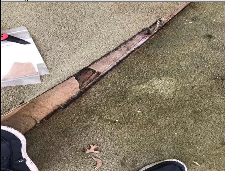
Photo 11: Asbestos Containing Floor Tile & Mastic Under Carpet Building A Room 17
