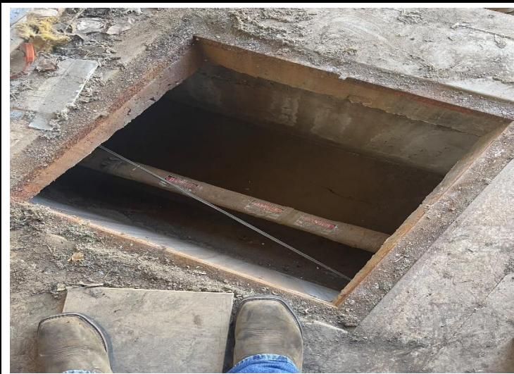
Photo 1: Parkside - Mand Hole in North Building - TSI
