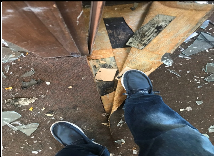
Photo 1: Asbestos Containing Floor Tile & Mastic Underneath Carpet Building B Room 4
