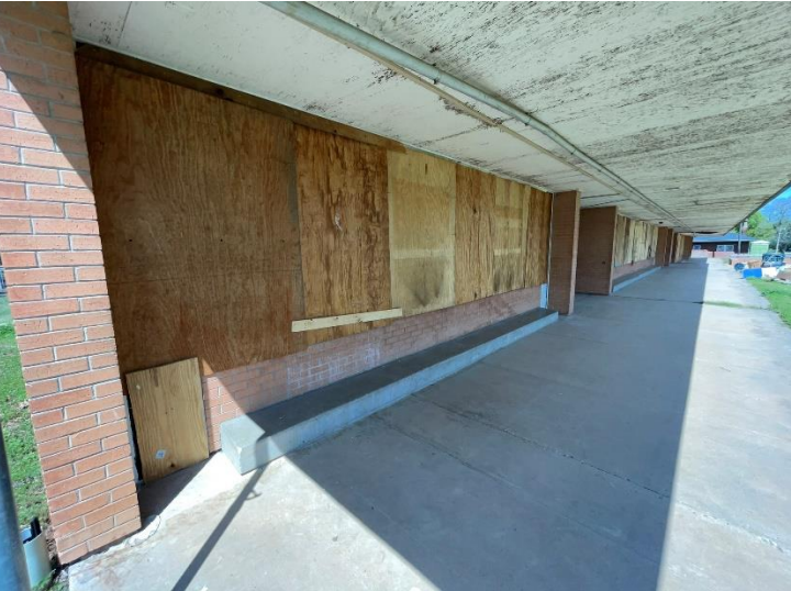
Photo 4: Parkside - South Building - Window Glaze Abated and Window Boarded
