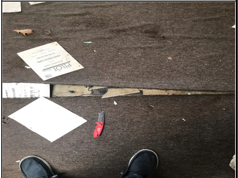
Photo 10: Asbestos Containing Floor Tile & Mastic Under Carpet Building A Room 18
