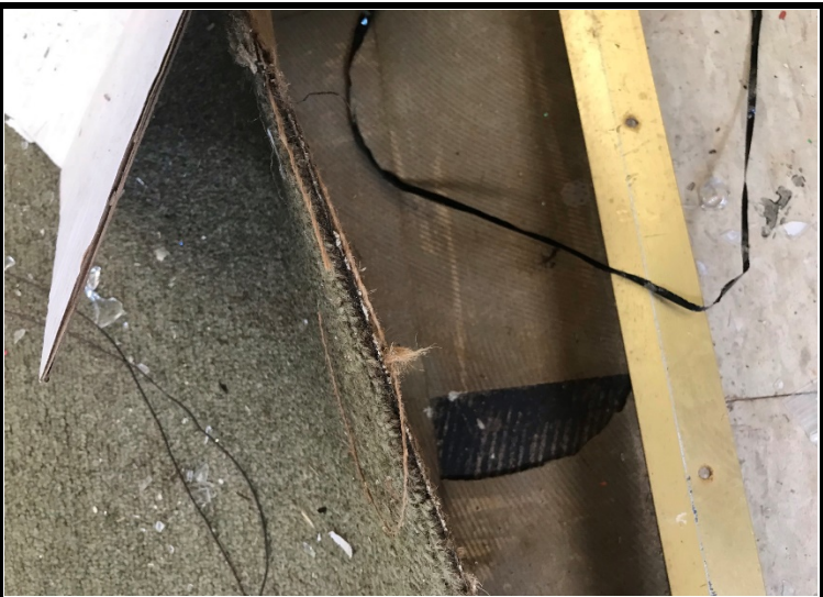
Photo 14: Asbestos Containing Floor Tile & Mastic Under Carpet Building C Room 23
