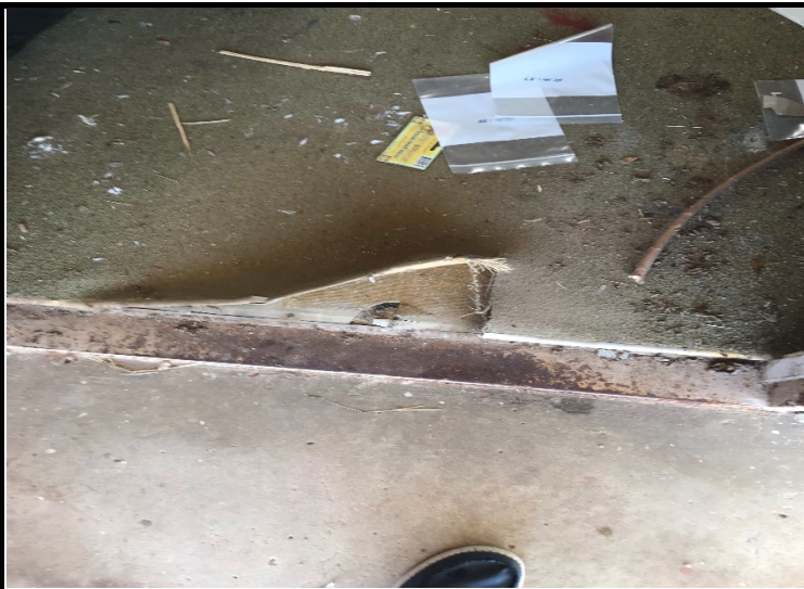
Photo 13: Asbestos Containing Floor Tile & Mastic Under Carpet Building C Room 20
