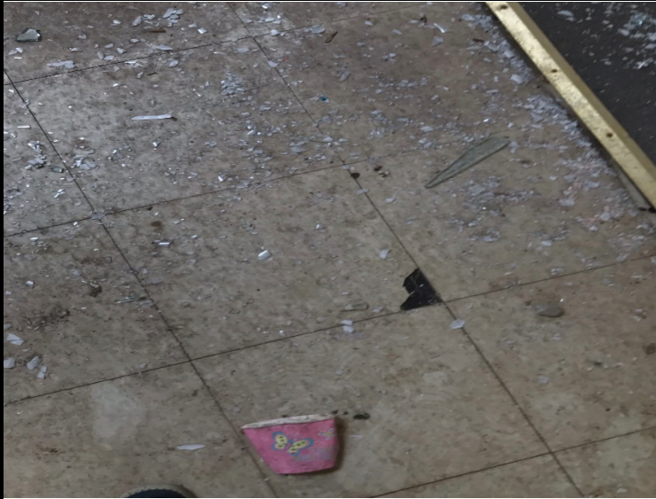
Photo 17: Asbestos Containing Floor Tile Mastic Under 12x12 Floor Tile Building C Room 26
