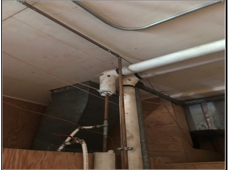
Photo 4: Asbestos Containing Pipe Insulation Building B Room 13
