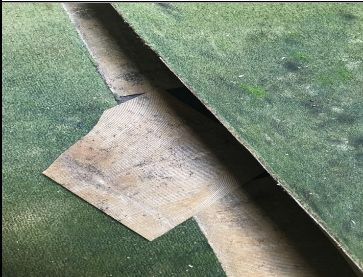
Photo 9: Asbestos Containing Floor Tile & Mastic Under Carpet Building A Room 19
