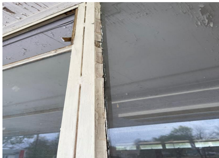
Photo 2: Parkside - North Building - Window Glaze
