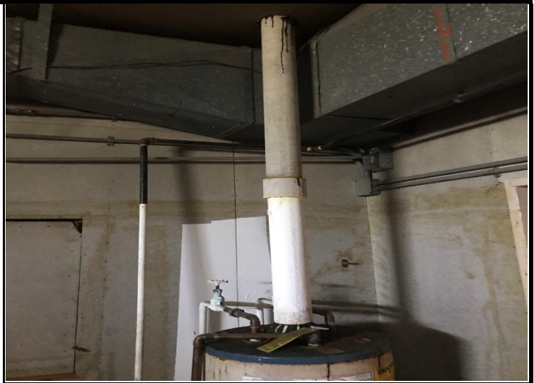
Photo 8: Asbestos Containing Transite Flue Building A Room 16
