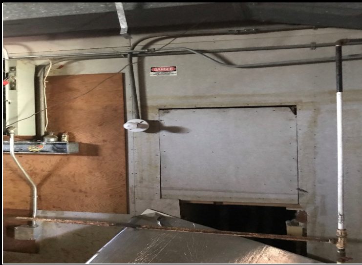
Photo 7: Asbestos Containing Transit Panels Building A Room 16
