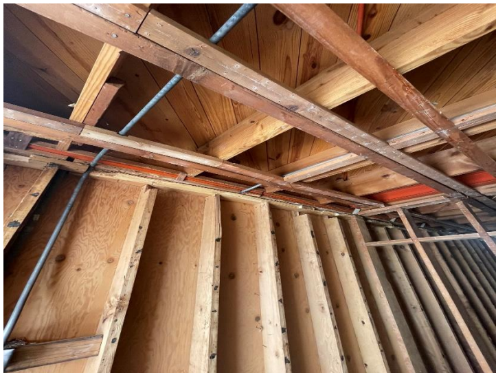
Photo 4: Parkside - South Building - Transit Abated
