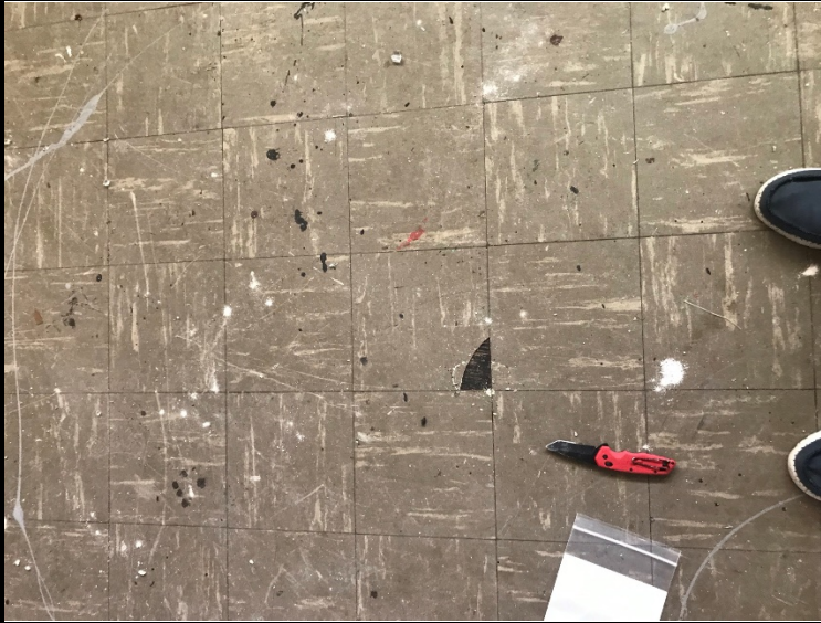
Photo 3: Asbestos Containing Floor Tile & Mastic Building B Room 10
