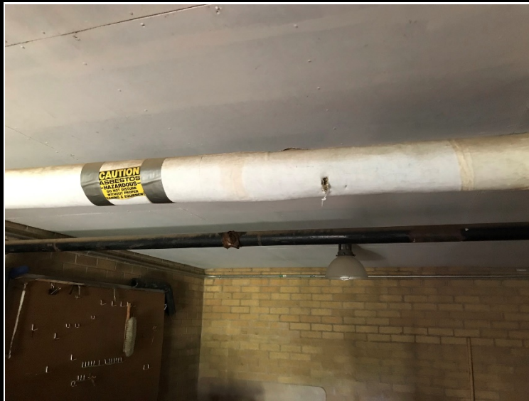
Photo 9: Asbestos Containing Pipe Insulation Ceiling Building 3 Custodial Room
