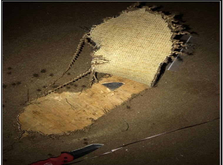
Photo 10: Asbestos Containing Floor Tile & Floor Tile Mastic Under Carpet Library Work Room
