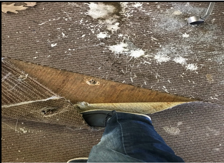
Photo 7: Asbestos Containing Floor Tile & Mastic Under Carpet Building 2 Room 8
