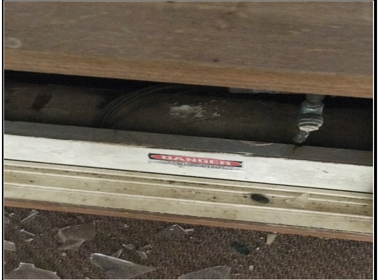
Photo 6: Asbestos Containing Pipe Insulation Under Sink Building 2 Room6
