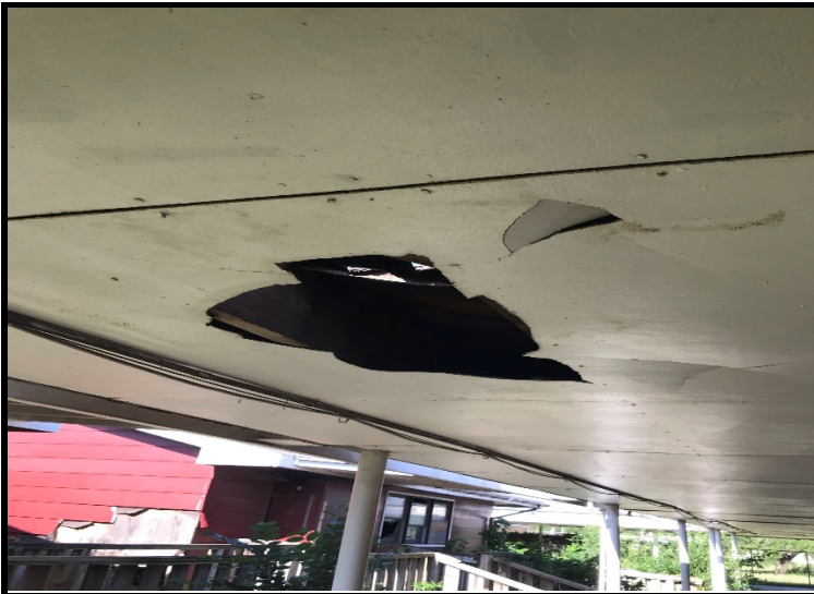
Photo 1: Asbestos Containing Transite Panels Middle Breeze Way
