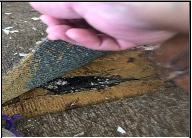
Photo 2: Asbestos Containing Floor Tile Under Carpet Building 1 Room 1
