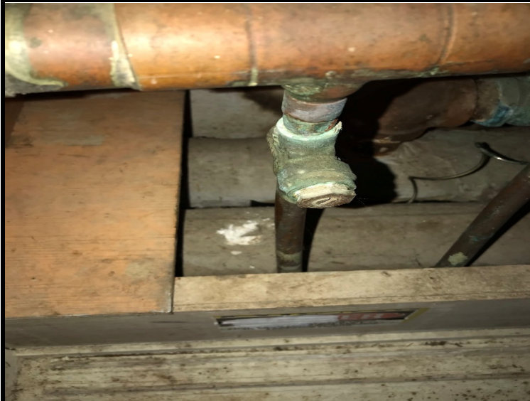
Photo 3: Asbestos Containing Pipe Insulation Under Sink Building 1 Room2
