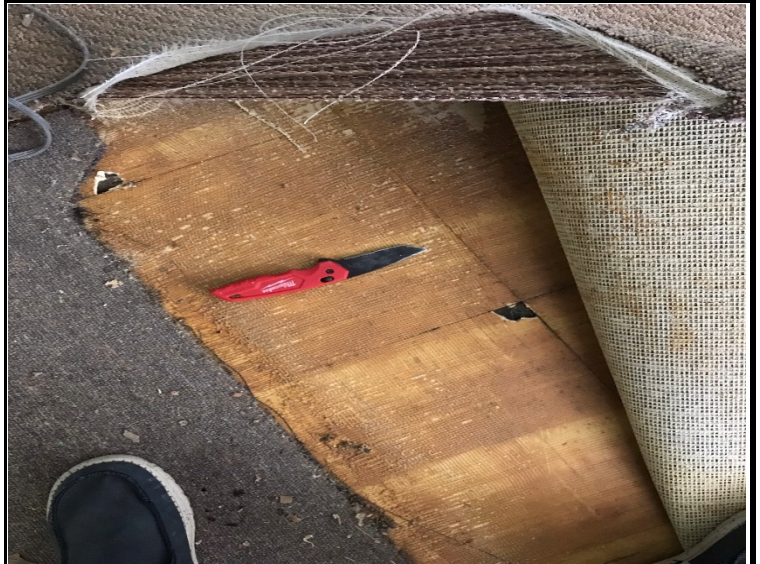
Photo 4: Asbestos Containing Floor Tile Mastic Under Carpet & 12x12 Floor Tile Building 2 Room 6
