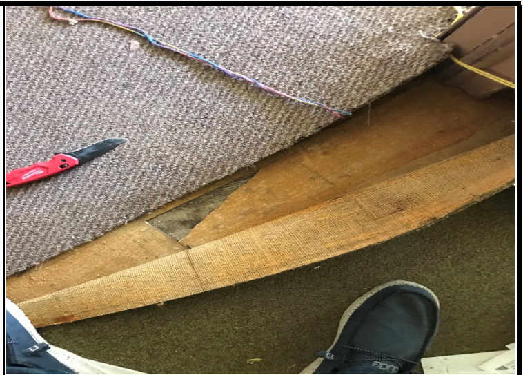
Photo 8: Asbestos Containing Floor Tile Under Carpet Building 2 Room 9B
