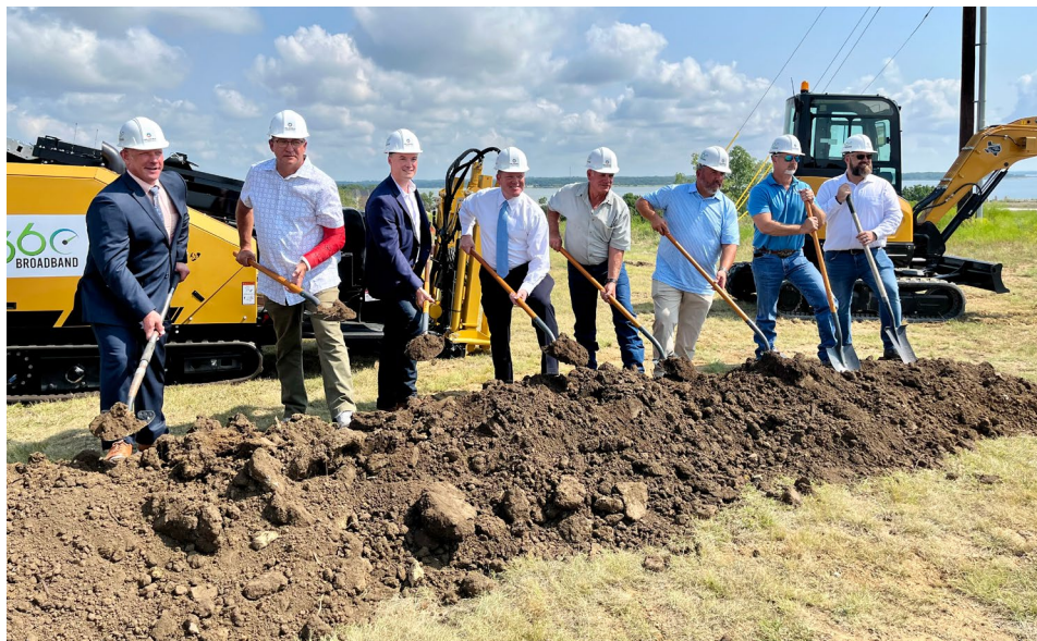
The OBO and 360 Broadband launched the first official groundbreaking for high-speed internet at an event along the banks of Lake Texhoma in Marshall County.
