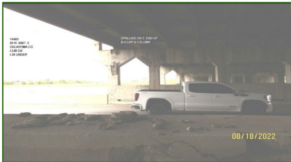
Figure 4. Existing Bridge Condition: Spalling
