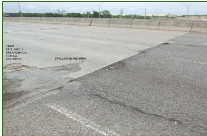
Figure 3. Existing Bridge Condition: Pavement
